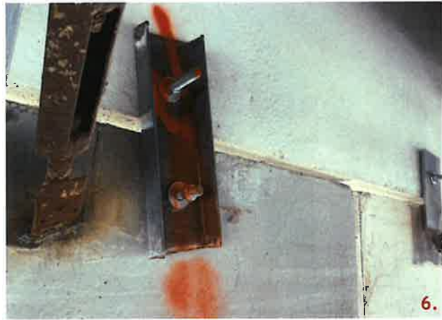
One connection point of panel 214 was field modified in similarity to FM-16.2. This connection is not installed with the appropriate hardware and does not meet the requirements of the approved FM.
