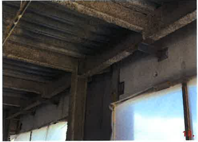
Panels 203B-2 & 249-3, connection points detailed 11 do not have 3/8x6x6 plates with slotted holes welded to the embedded plate.
