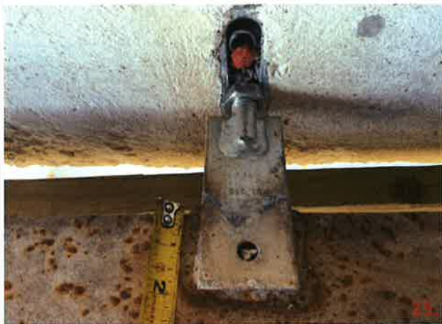
Panel 104 and 130 at connection points 03 have PSA straps that have a weld length of approximately 2" on each side and the end of the strap (three sides).
