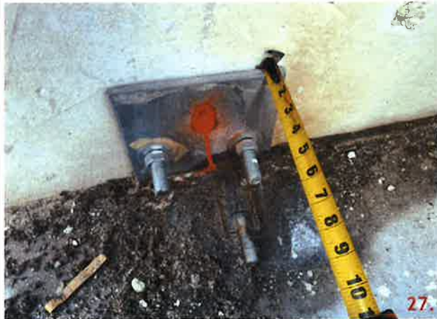
Panel 207-2 & 235-2 have connection points that has been field modified similar to FM-9.2. A 6" PSA strap was used at this connection instead of a 3/8x3x5 plate. The plates attached to the panel are 1/2" thick. FM9.2 requires 3/4" plates.
