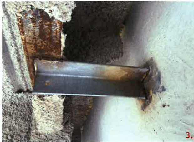
Panel 217A-2, connection points detailed 11 do not have 3/8x6x6 plates with slotted holes welded to the embedded plate. These connections are welded directly to the embedded plate and structural steel.
