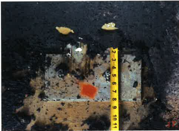
Panel 202-2 and 233-1 are connected to the slab with a PSA strap that is welded to plate 1/2"x6"x12". This plate is anchored to the slab with (2) 5/8" anchors. These anchors are approximately 5" from the edge of the slab.
