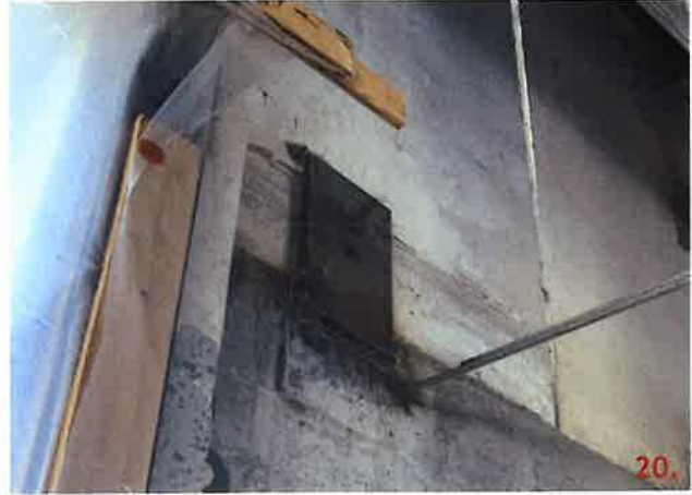
Panel 228-1 is not connected to panel 223-1 as detailed on 16.
