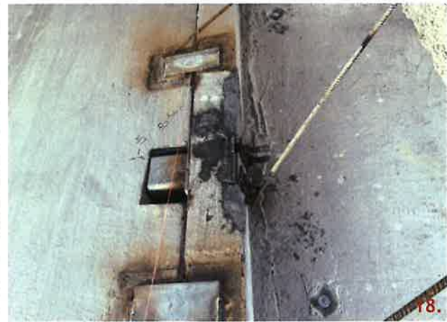
Panel 246 at grid line 5 has one HSS6x3x3/8 and p7 plate bolted through the panel edge. This connection meets the requirements of the approved field modification FM18-3.
