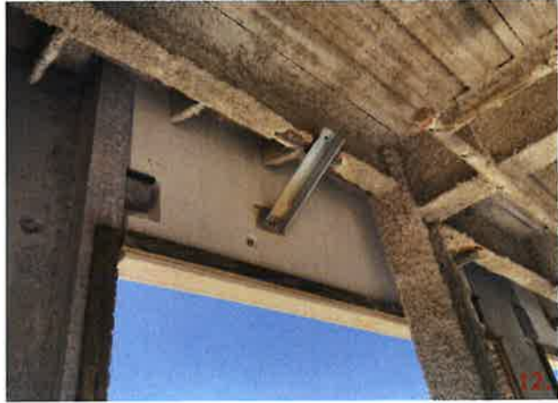
Panel 217 at elevation 34'-0" at grid line 3 has one L4x4x3/8 that is installed at an angle due to misalignment of the embed plate.
