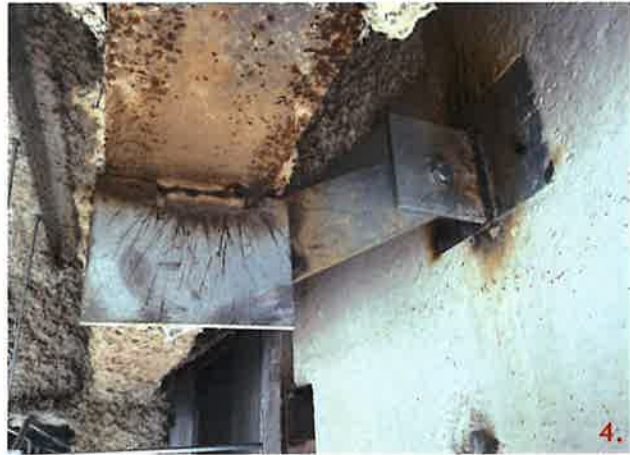
Panel 217-3, has been been modified with FM-11.1. This detail requires the use of a L4x4x3/8 to be welded to the structural steel. This connection has a 6x8x3/8 plate instead. EOR, is this structurally acceptable?
