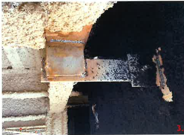
Panel 109A has been modified with FM-11.1. This detail requires the use of a L4x4x3/8 to be welded to the structural steel. This connection has a 6x6x3/8 plate instead.
