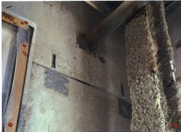
Panel 225-2 is not connected to panel 219-1 as detailed on 16.
