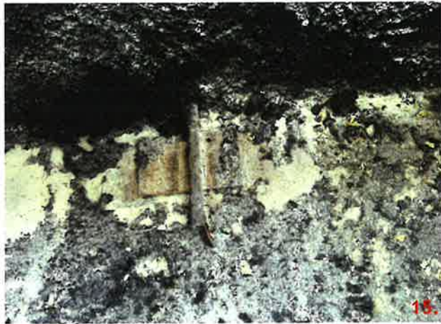
Panel 114 has two connections detailed 09 that have been field modified similar to FM 10-4.
