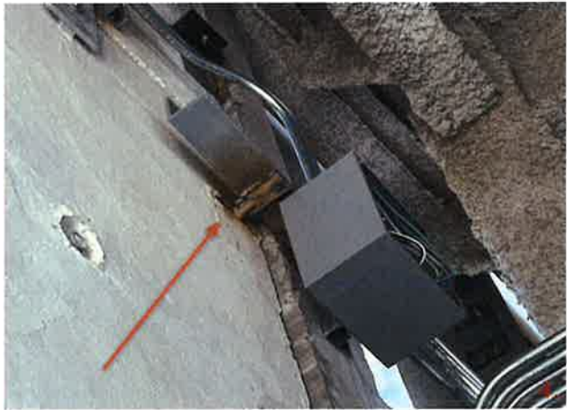
Panel 243 near grid line 4 at elevation 16'-0" has an angle welded to the plate and the 6" PSA strap.
