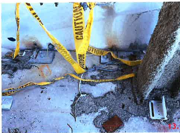
Panel 129-2 is connected to the slab at two connections with a PSA strap that is welded to plate 1/2"x6"x12". This plate is anchored to the slab with (2) 5/8" anchors. These anchors are approximately 4" from the edge of the slab.
