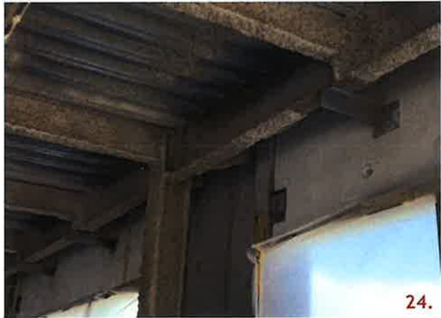
Several connections detailed 11 do not have the 3/8x6x6 plate with 13/16 x 2" slotted hole welded to the embedded plate in the panels. The L4x4x3/8 are welded directly to the embedded plates.
