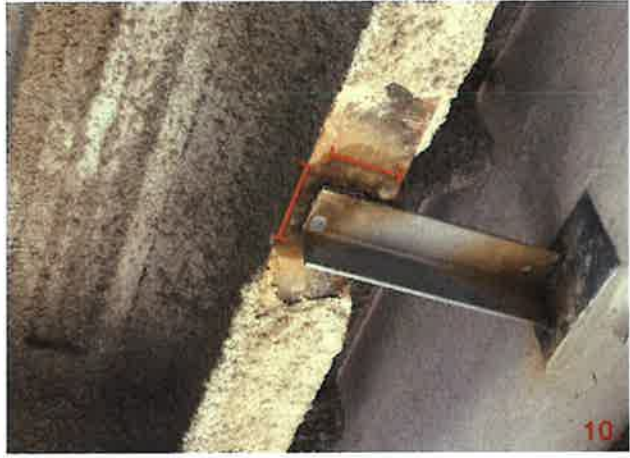
Both panels 217 at elevation 34'-0" near grid line 5 and 6 have L4x4x3/8 that are welded with 6" of 1/4" fillet weld to the beam but not in the detailed locations.
