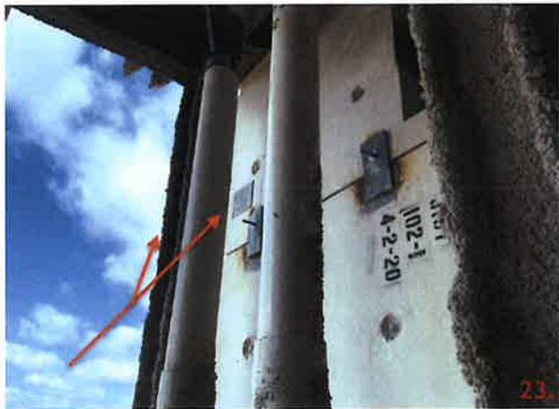
Panel 103-2 is not connected to the structural steel as detailed on 28.
