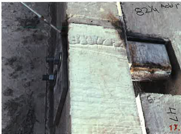
Panel 247 at grid line 4 has two HSS6x3x3/8 and p7 plate bolted through the panel edge. The lower connection at approximately elevation of 6" only has two (2) 3/4 threaded rods at this connection.
