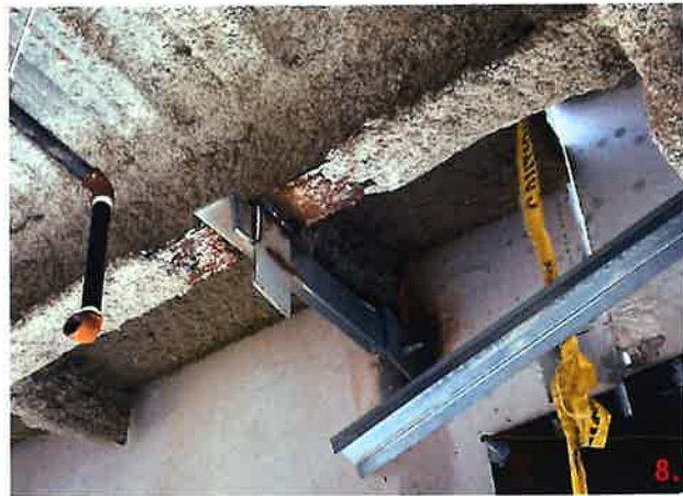
Panel 229-1 has been modified with FM-11.1. This detail requires the use of a L4x4x3/8 to be welded to the structural steel.
