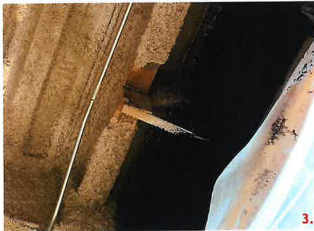
Panel 217-2 & 217-1 have been modified with FM-11.1. This detail requires the use of a L4x4x3/8 to be welded to the structural steel. This connection has a 6x8x3/8 plate instead.
