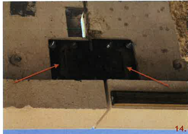
The P7 plate is missing from panel 228 at grid line 3 at elevation 49'-4". Field modification FM18-7 was used at this location. The welds of the connection are on the vertical leg of the 3/4x8"x1'-4" plate and do not have a 1" return.
