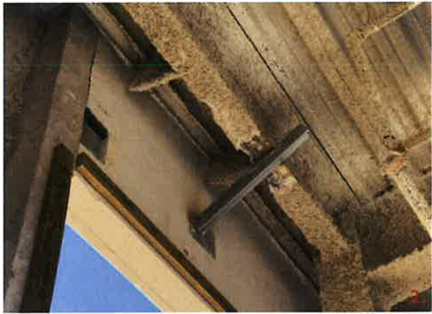
Panel 217 at elevation 20'-0" at grid line 3 has one L4x4x3/8 that is installed at an angle due to misalignment of the embed plate.
