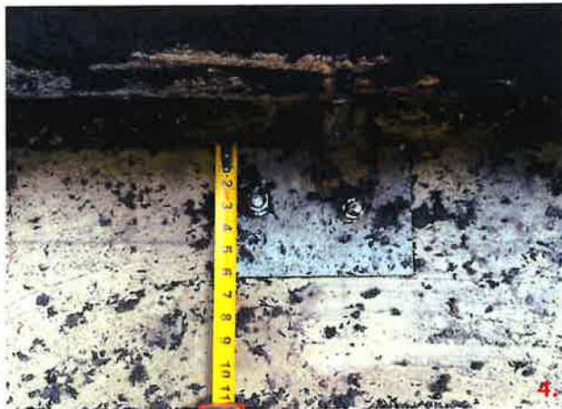
Panel 109B at one connection point detailed 10 is connected to the slab with a PSA strap that is welded to plate 3/8"x6"x8".
