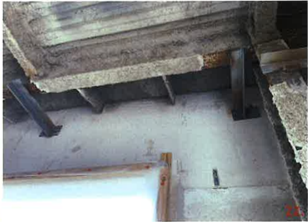
Panels 235-2 & 236-2 have several connections that are not installed as detailed on 23. A plate was used to weld to the angle instead of the PSA strap.
