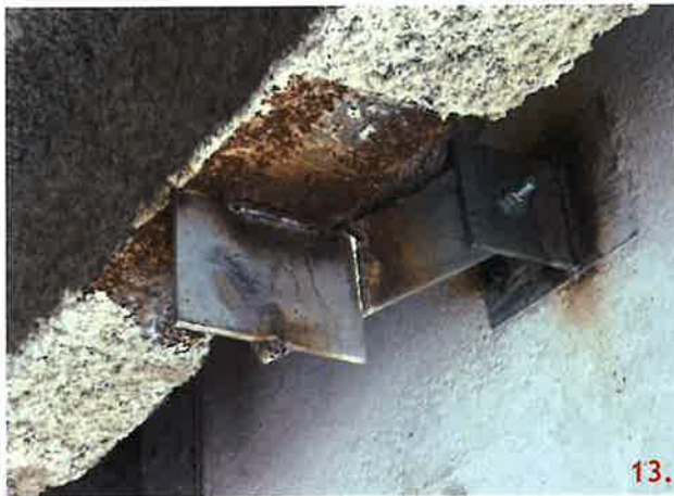
Panel 217B-3 at the east end, has been modified with FM-11.1. This detail requires the use of a L4x4x3/8 to be welded to the structural steel. This connection has a 6x8x3/8 plate instead.
