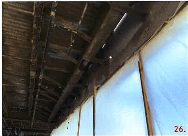
Panel 208, 209, 237, 238 connection points detailed 21 do not have 3/8x6x6 plates with slotted holes welded to the embedded plate. These connections are welded directly to the embedded plate and Structural steel.
