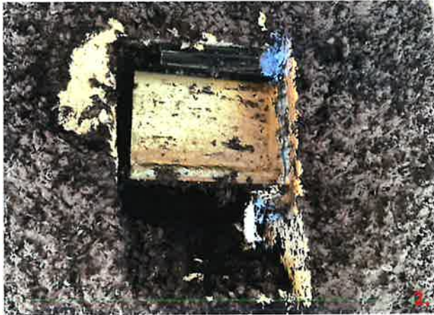
An example of FM18.2 on panels 109 that have been completed as detailed.
