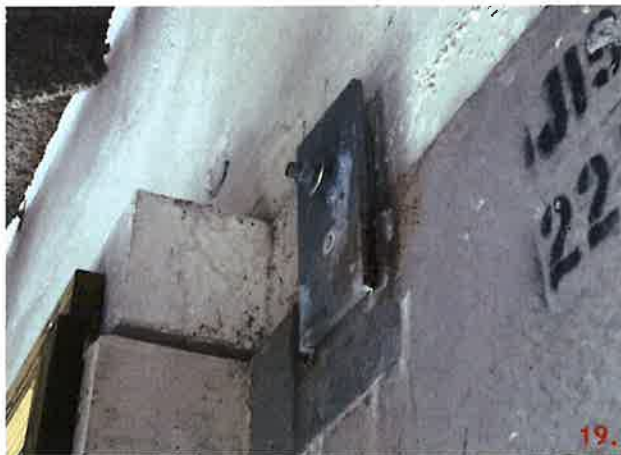
Connection of panel 223 and 228 at elevation 44'-0" at grid line 4 has a 3/4 threaded rod nut that is loose.
