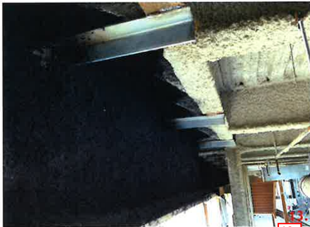
Panel 118 has four connections detailed 11. The L4x4x3/8" is welded directly to the embedded plate.
