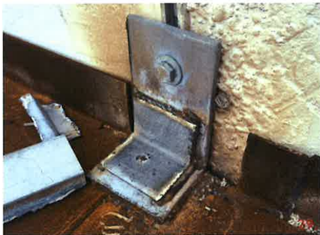
Panel 104-1 has two PSA inserts that are too high.
