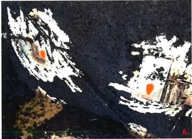
Panels 107-6 and 112 have connection points detailed 16 where PSA insets and embed plates that do not align. The plates are only welded on one side to the embed plate.
