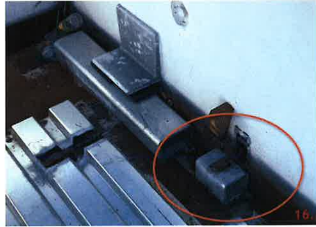
Near grid line 3 at elevation 66'-4" on panel 232 the HSS installed at this location is not the size noted on the field modification.
