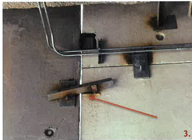
Panel 211B has a plate anchored to the panel and an angle welded to the plate and the 6" PSA strap.
