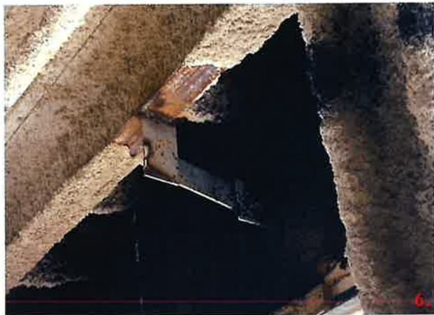
Panel 217-4 & 217-3 have been modified with FM-11.1. This detail requires the use of a L4x4x3/8 to be welded to the structural steel. This connection has a 6x8x3/8 plate instead.
