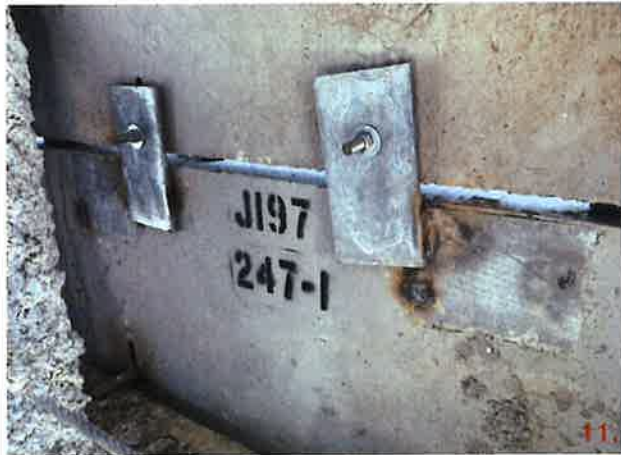
Panel connections of 247 and 223 at elevation 34'-0" at grid line 4 are not aligned with the embed plate. The plates are only welded on one side.
