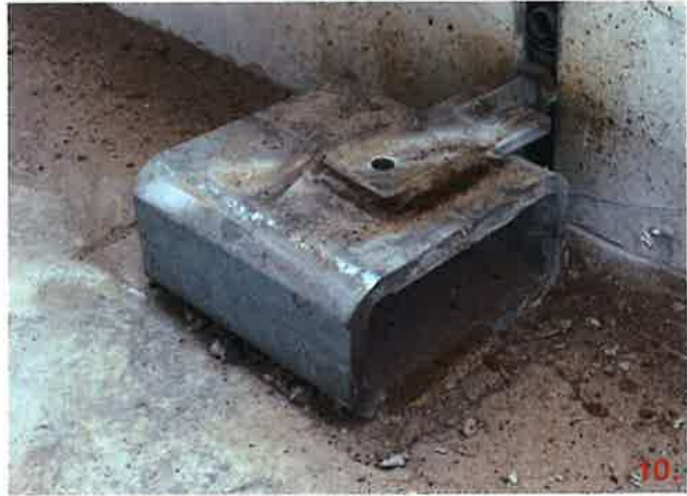
Panel 217A-2 has a PSA insert that is installed too high. A HSS3x6X6" is welded to the embedded plate with a 3" 3/16 fillet each side. The PSA strap is welded to the HSS.
