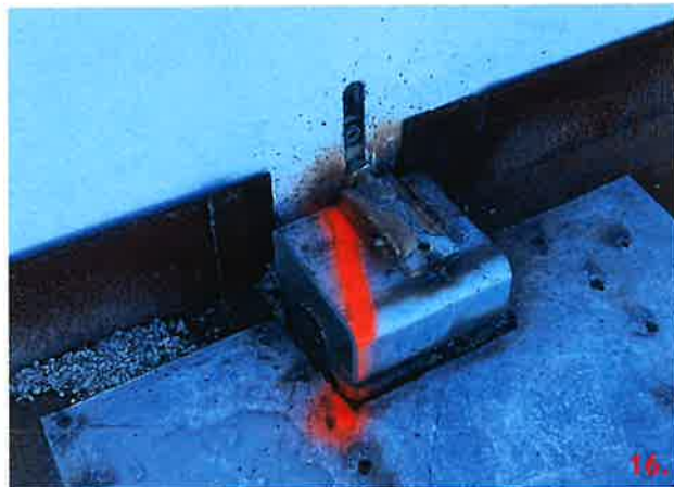
Panel 130-1 has a connection point detailed 02 that has a HSS6x3x3/8 6" length below the PSA strap. A FM was not provided for this connection.
