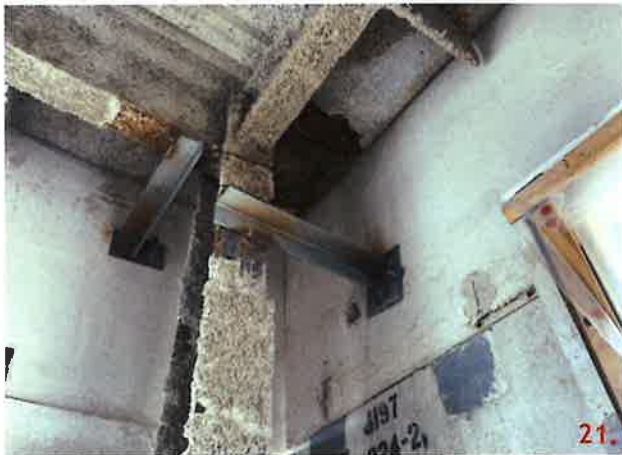
Panel 229 is not connected as detailed on 28. The embedded plate was not installed in the panel. A plate has been anchored to the panel.
