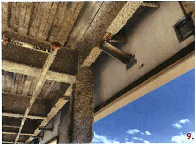
Panel 217 at elevation 34'-0" at grid line 6 has one L4x4x3/8 that is installed at an angle due to misalignment of the embed plate.
