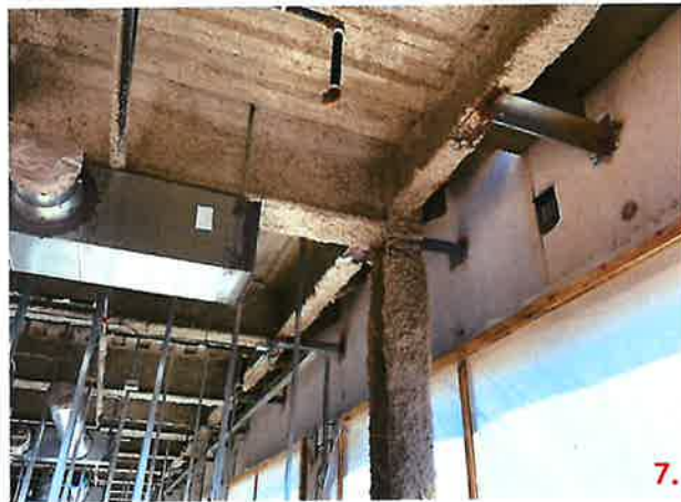
Panel 225-1, 226-1, 227-2, 228-2, connection points detailed 11 do not have 3/8x6x6 plates with slotted holes welded to the embedded plate. These connections are welded directly to the embedded plate and Structural steel.
