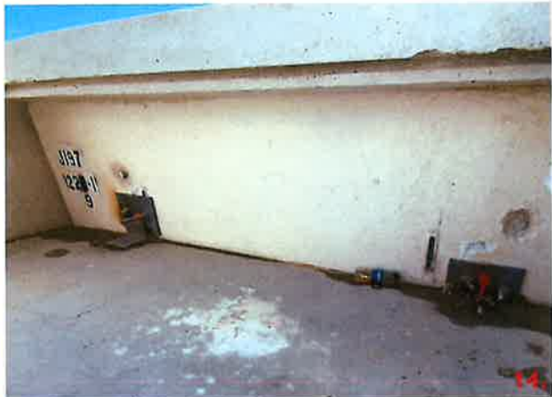
Panel 229-1 has two connections detail 10 that have been field modified.
