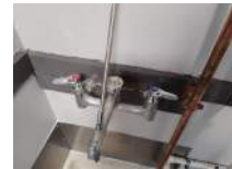
Mech Closet 11 Darryl Dilmore Aug 30, 2022 9:46 AM
