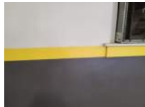
Wall at Top of West Bleachers From South to North Photo 2 Darryl Dilmore Aug 30, 2022 11:08 AM
