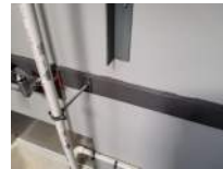
Mech Closet 9 Darryl Dilmore Aug 30, 2022 9:46 AM
