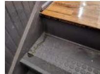
Women's Locker Stairwell Top Tread Photo 3
