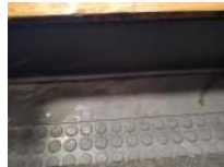
Women's Locker Stairwell Top Tread Photo 2
