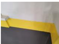
Wall at Top of West Bleachers From South to North Photo 7 Darryl Dilmore Aug 30, 2022 11:09 AM
