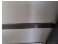
Mech Closet 8 Darryl Dilmore Aug 30, 2022 9:46 AM
