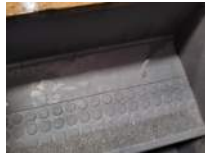
Women's Locker Stairwell Top Tread Photo 1
