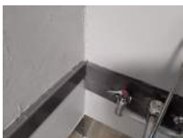
Mech Closet 12 Darryl Dilmore Aug 30, 2022 9:46 AM
