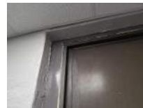
Mech Closet 18 Darryl Dilmore Aug 30, 2022 9:47 AM
