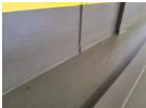
Wall at Top of West Bleachers From South to North Photo 1 Darryl Dilmore Aug 30, 2022 11:08 AM
