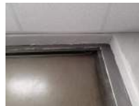
Mech Closet 17 Darryl Dilmore Aug 30, 2022 9:47 AM
