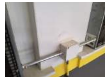
Wall at Top of West Bleachers From South to North Photo 4 Darryl Dilmore Aug 30, 2022 11:09 AM
