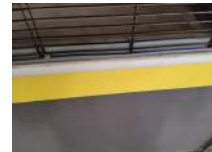
Wall at Top of West Bleachers From South to North Photo 6 Darryl Dilmore Aug 30, 2022 11:09 AM
