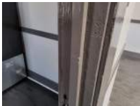
Mech Closet 1 Darryl Dilmore Aug 30, 2022 9:45 AM
