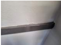
Lobby 59 Darryl Dilmore Aug 30, 2022 10:00 AM
