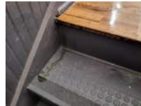
Women's Locker Stairwell Top Tread Photo 3
