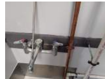
Mech Closet 10 Darryl Dilmore Aug 30, 2022 9:46 AM
