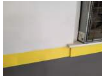
Wall at Top of West Bleachers From South to North Photo 3 Darryl Dilmore Aug 30, 2022 11:08 AM
