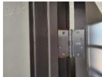
Mech Closet 2 Darryl Dilmore Aug 30, 2022 9:45 AM
