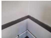
Mech Closet 7 Darryl Dilmore Aug 30, 2022 9:46 AM
