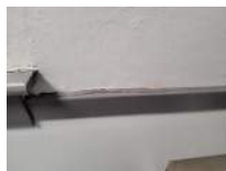
Mech Closet 13 Darryl Dilmore Aug 30, 2022 9:46 AM
