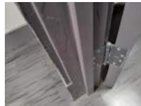
Mech Closet 3 Darryl Dilmore Aug 30, 2022 9:46 AM
