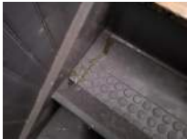
Women's Locker Stairwell Top Tread Photo 4
