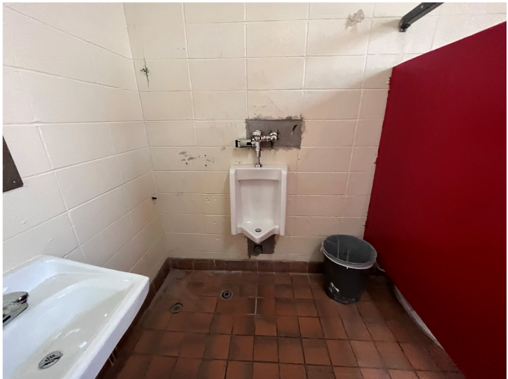
Figure 2 – New Touchless Fixtures at Leflore County
