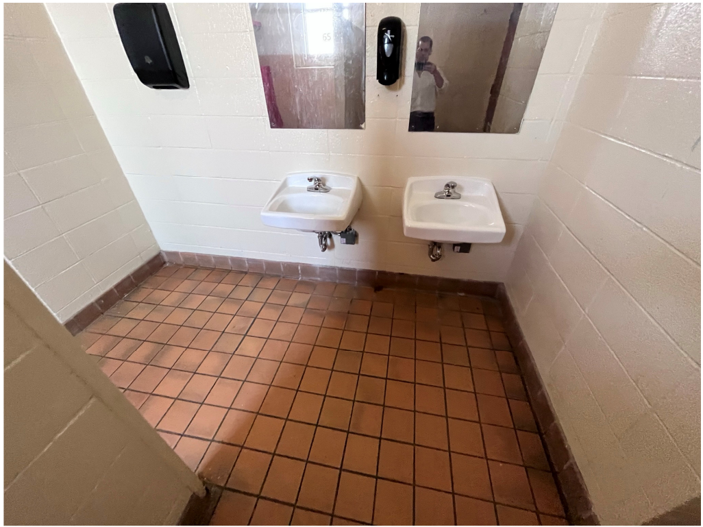
Figure 3 – New Touchless Fixtures at Leflore County
