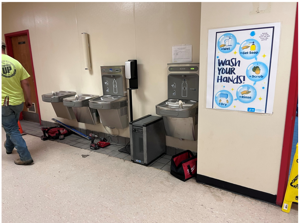
Figure 2 – New Water Fountains at Leflore County
