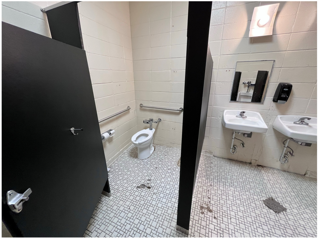
Figure 3 – This does not look like it meets our minimums; check A-401d/8 for conformance
