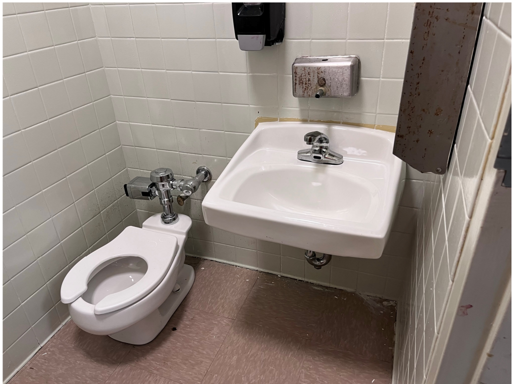
Figure 2 – New Toilet Fixtures at Davis Elementary
