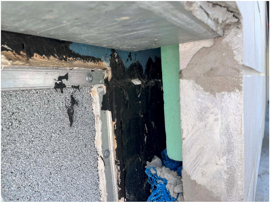
Figure 46 – TEHS: NE Roof Connection at Lobby: foam in gap; cover with metal flashing
