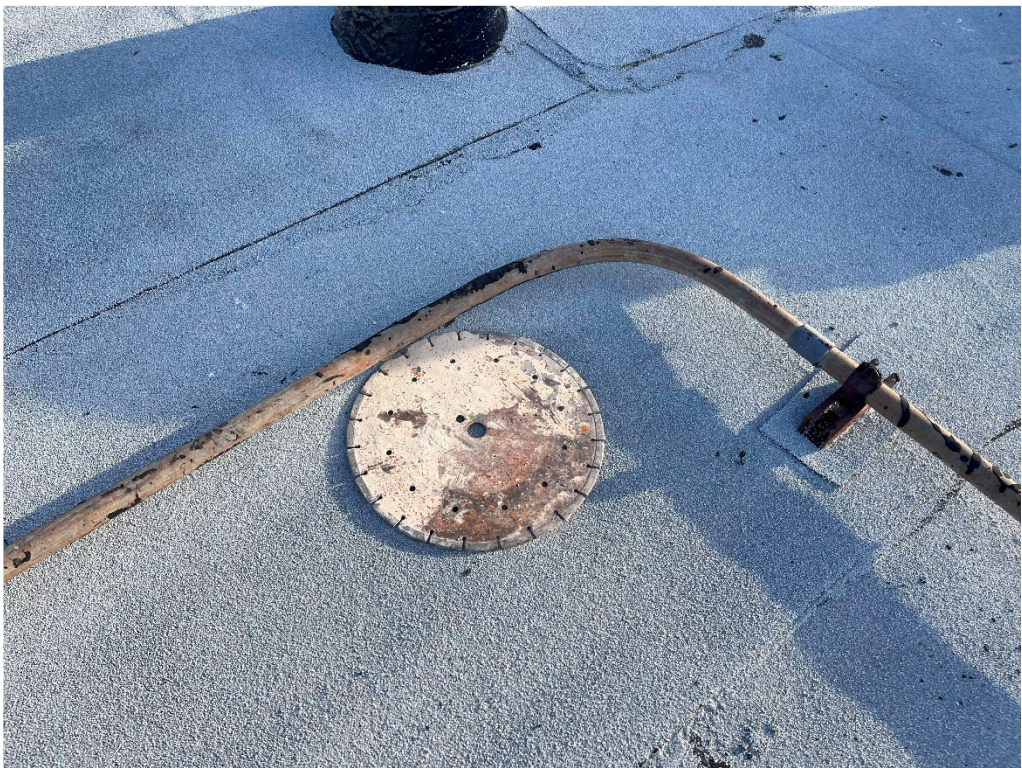
Figure 6 – GHS: contractor is reminded to clean up and the end of each; hazards like the type shown could cause damage to property or injury to person if left on the roof, unsecured over night
