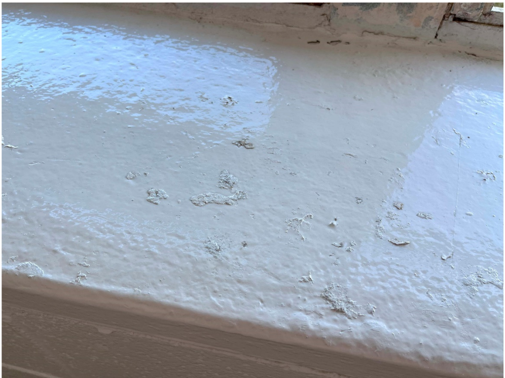
Figure 22 – GHS: debris noted beneath paint at existing seal shall be removed prior to paint
