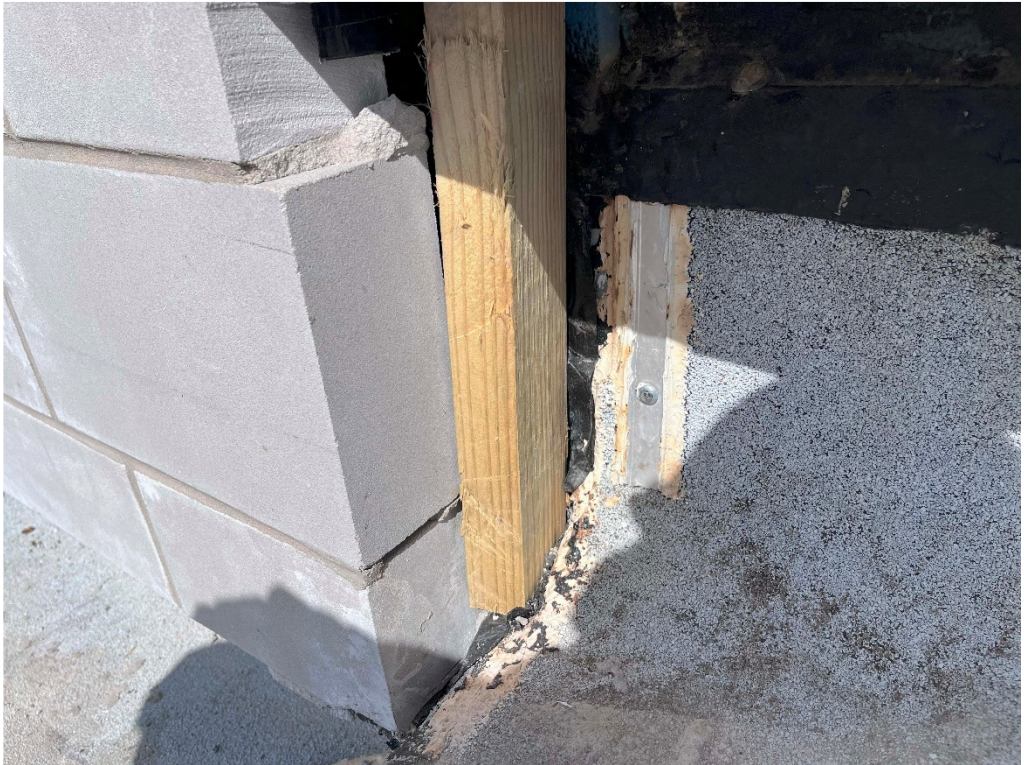
Figure 47 – TEHS: SE Roof Connection to Lobby: remove deadwood; foam in gap and install metal flashing in place
