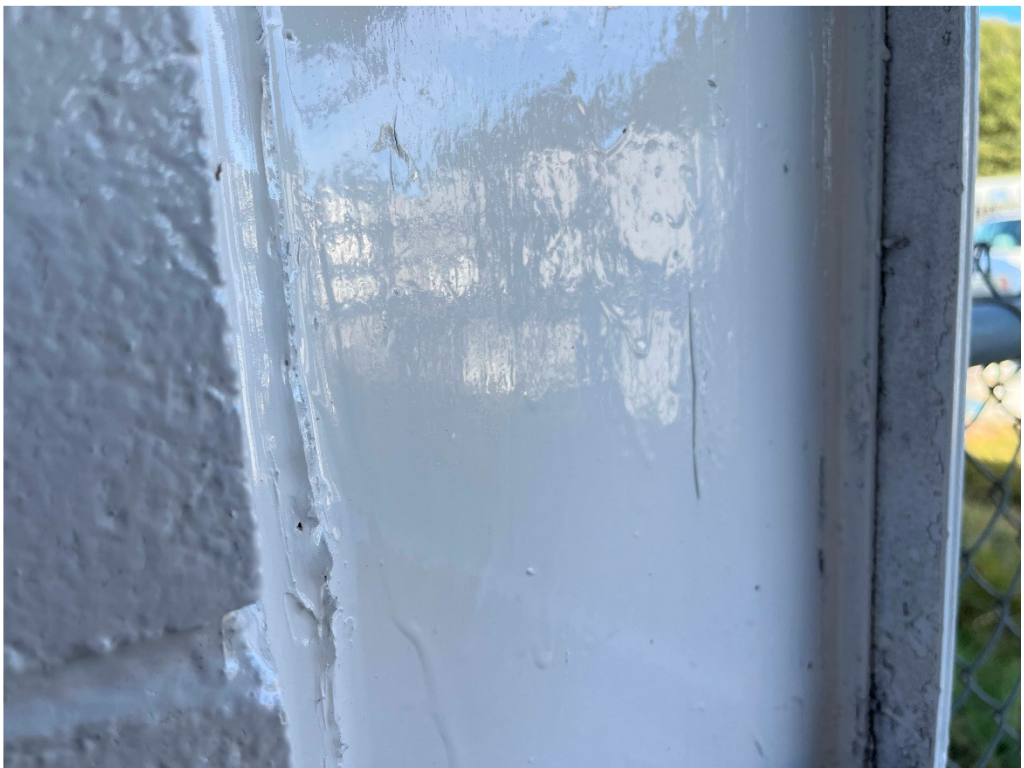
Figure 24 – GHS: drips and runs in paint shall be sanded, removed, and repainted
