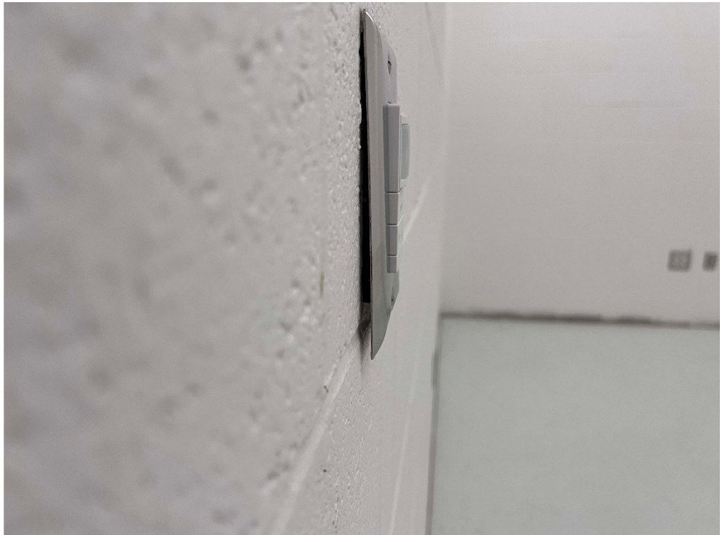
Figure 36 – TEHS: contractor is reminded to install all electrical plates flush with wall surface
