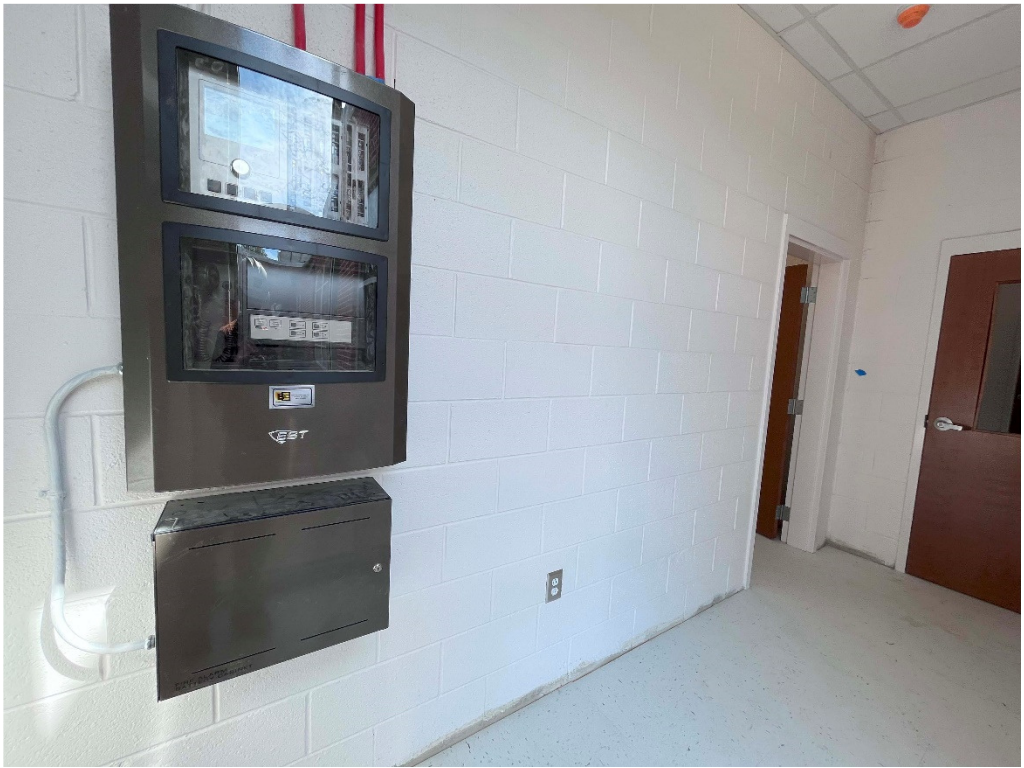
Figure 34 – TEHS: fire alarm equipment installed
