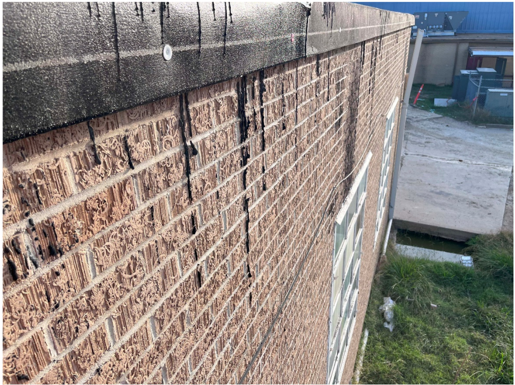
Figure 2 – GHS: contractor reminded to clean all asphalt from face of brick
