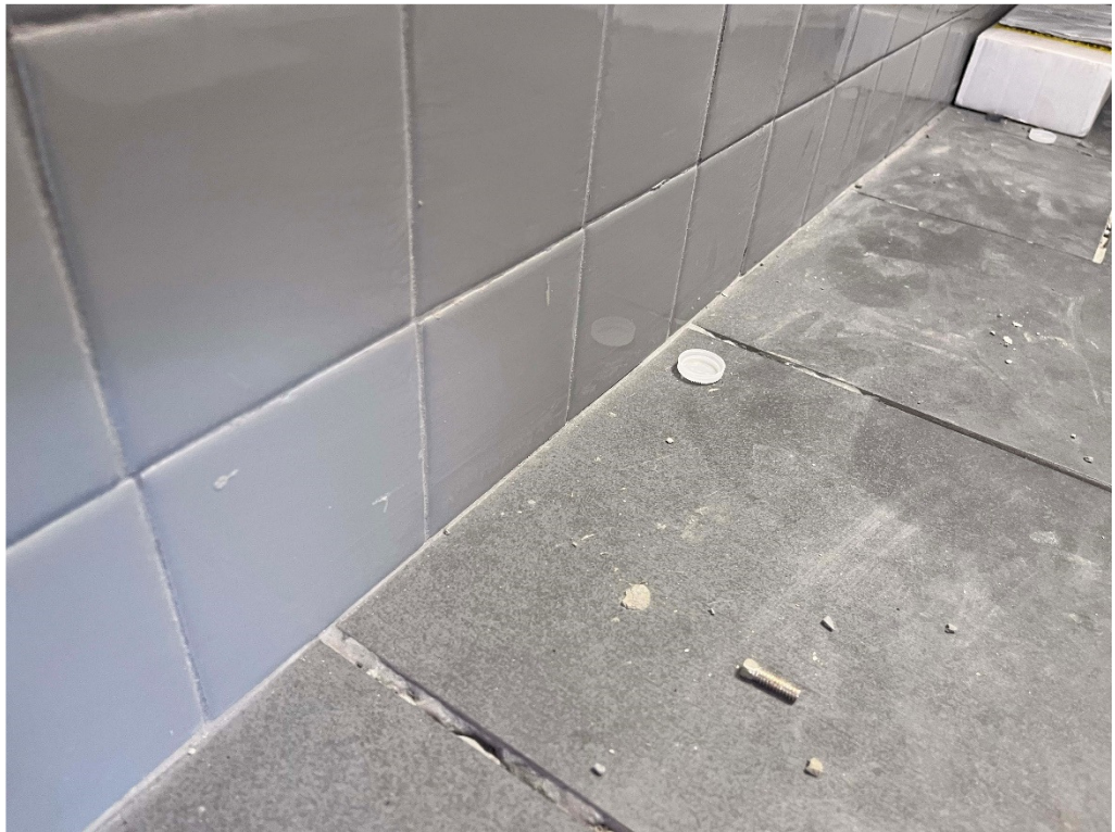
Figure 38 – TEHS: cove tile missing from toilet rooms; a credit in lieu of replacement could be considered; make proposal
