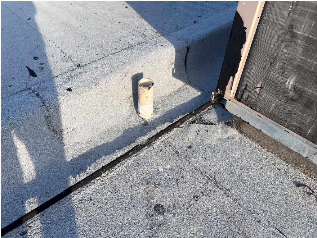
Figure 5 – GHS: this pipe does not appear to meet 12 MIN clearance requirements
