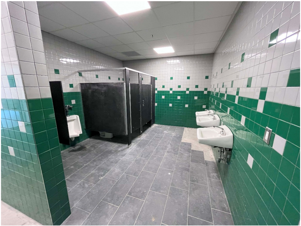
Figure 41 – TEHS: progress noted at toilet rooms; NOTE cove tile missing here also
