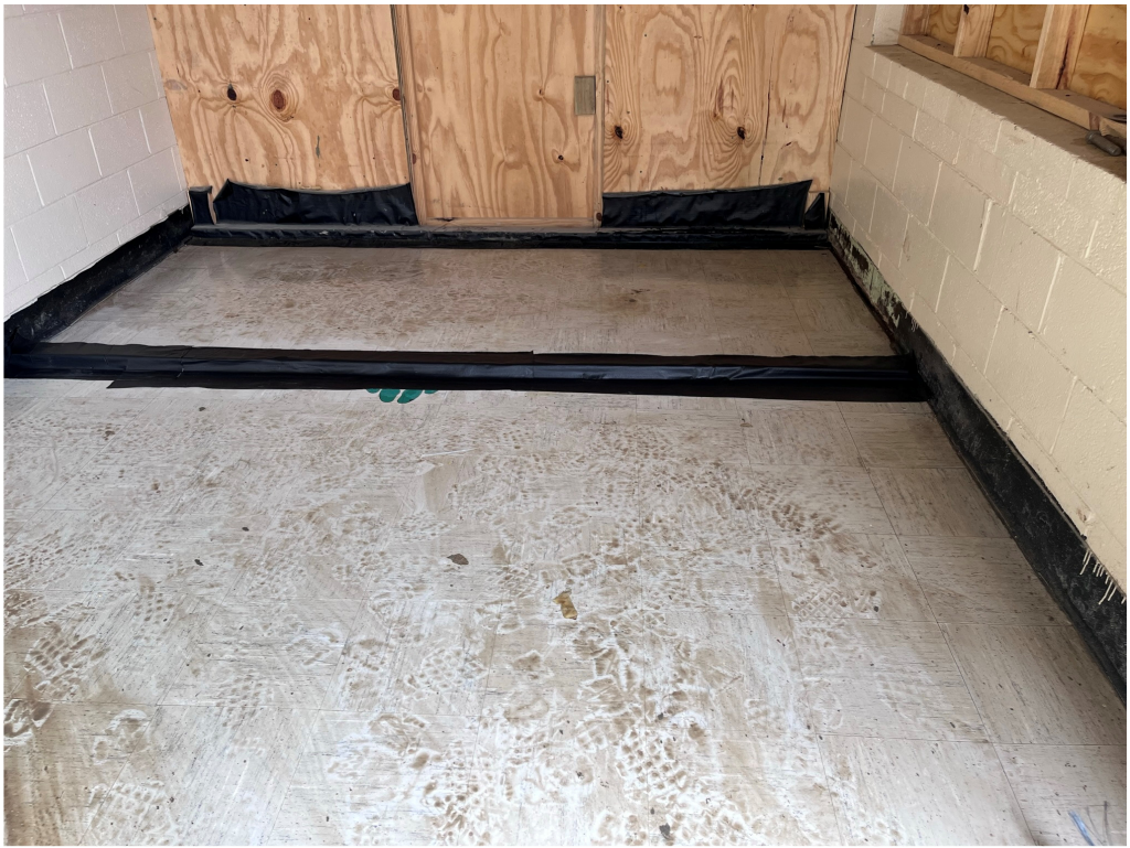
Figure 31 – Contractor Dams appear to be working at keeping water from main building
