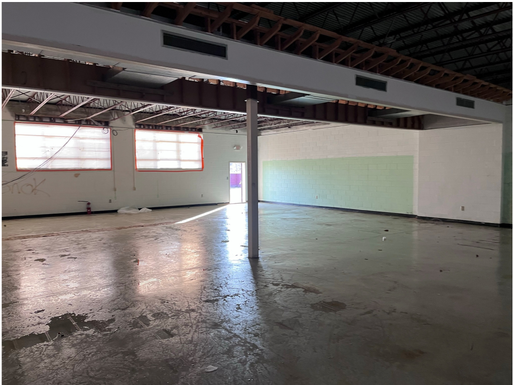
Figure 7 – Media Center Demolition; Sweating is an issue and needs to be addressed to prevent degradation of existing materials to remain
