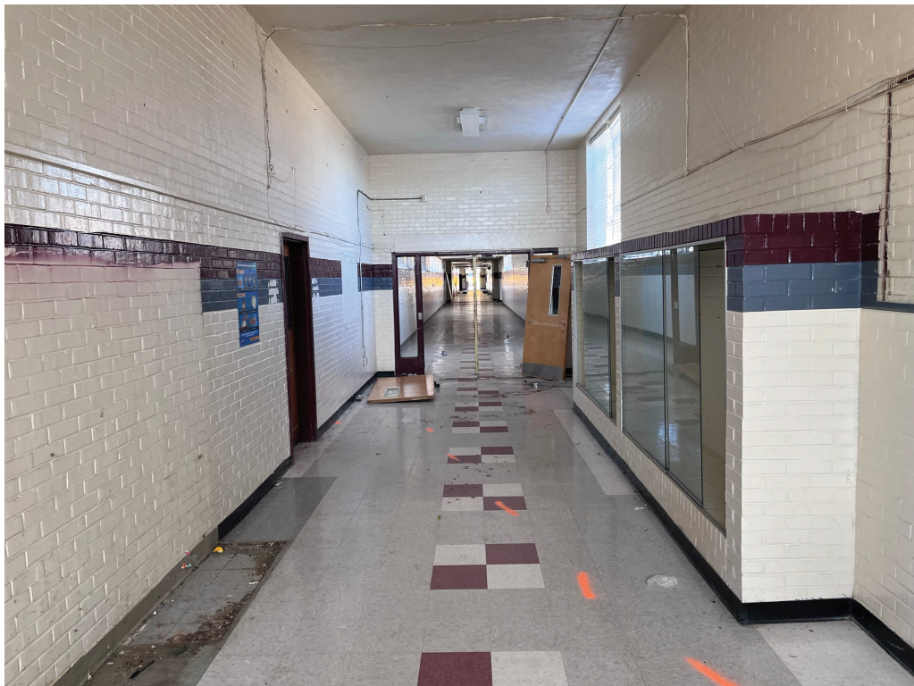
Figure 2 – Wall on right called to be removed
