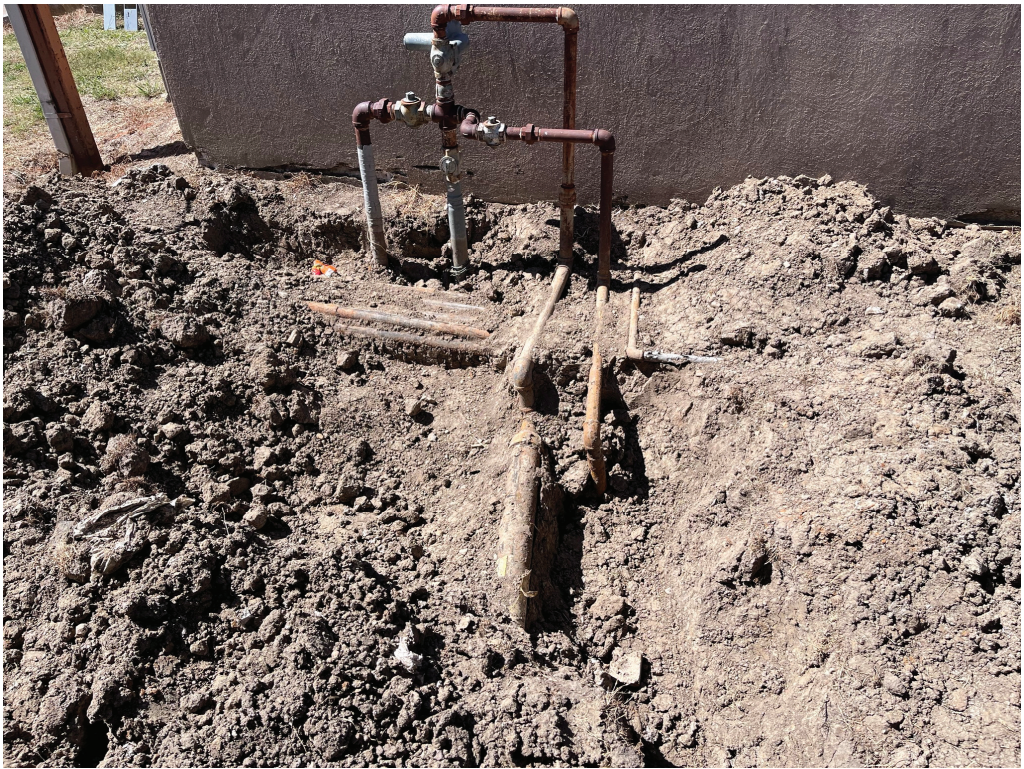
Figure 11 – S Gas intro at building
