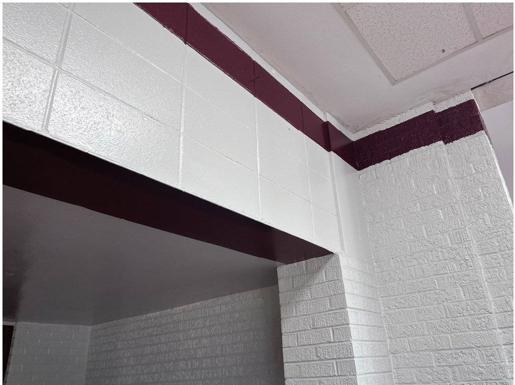
Figure 14 – Beam at Pilaster in question
