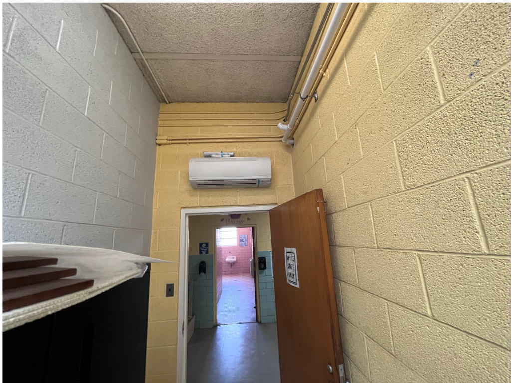
Figure 18 – AW James Typical Wall Unit Set
