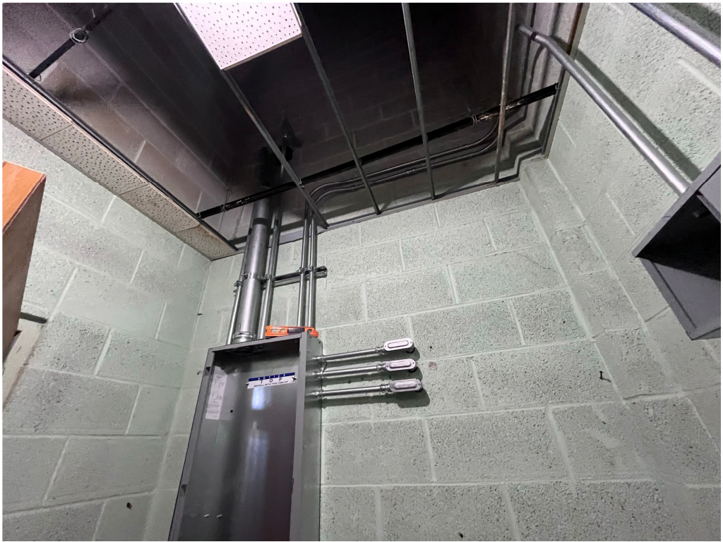
Figure 22 – AW James Electrical
