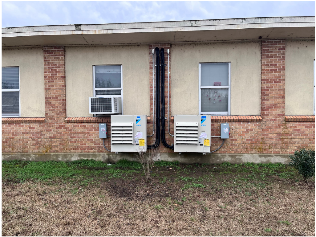
Figure 5 – Unit ARE lined up equal distance from brick edges and this is acceptable
