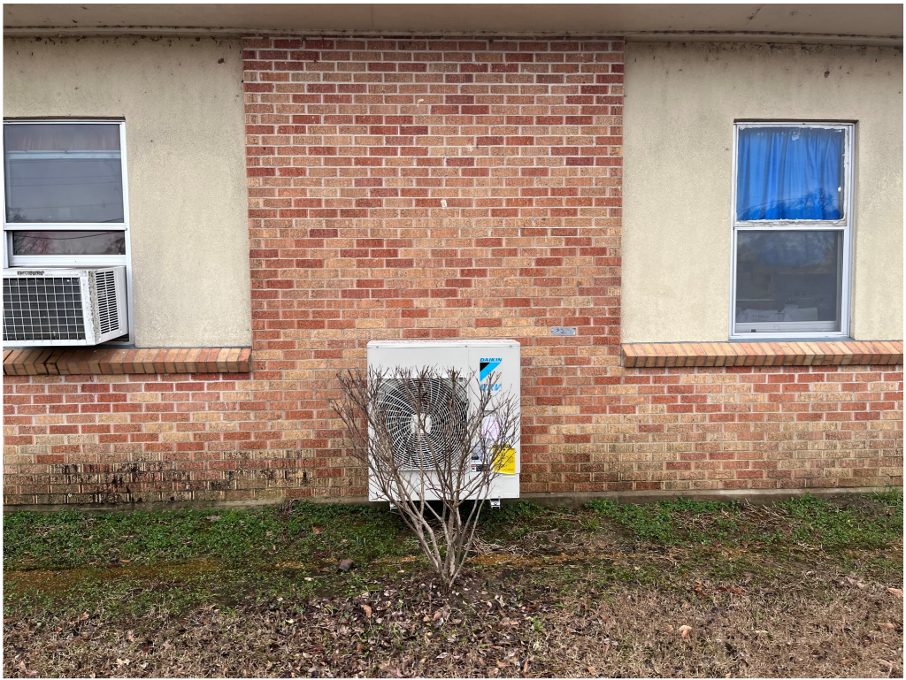
Figure 7 – Unit Centered is good install
