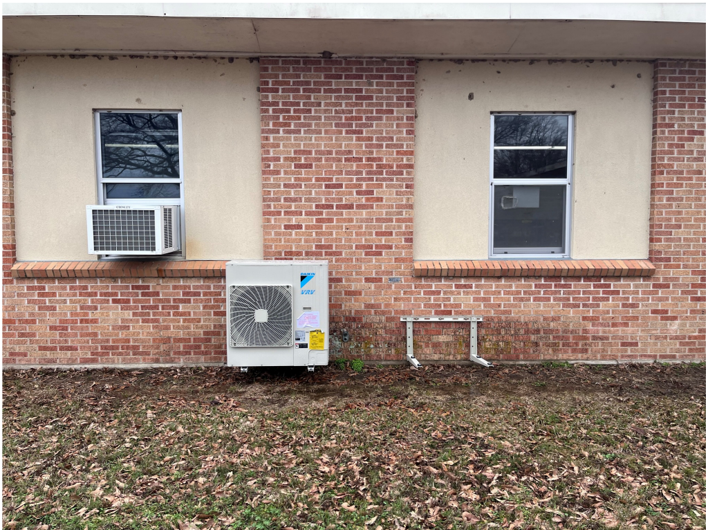
Figure 9 – Unit mis-aligned are not acceptable
