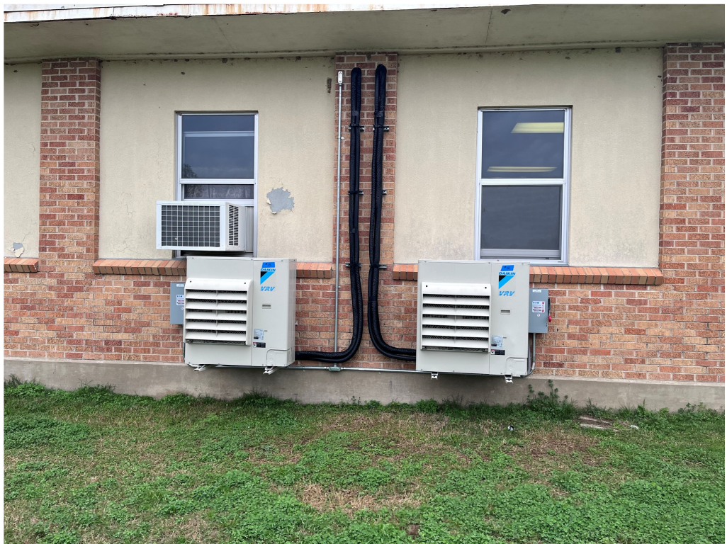
Figure 6 – Units ARE NOT lined up as in submitted diagram; this is not acceptable
