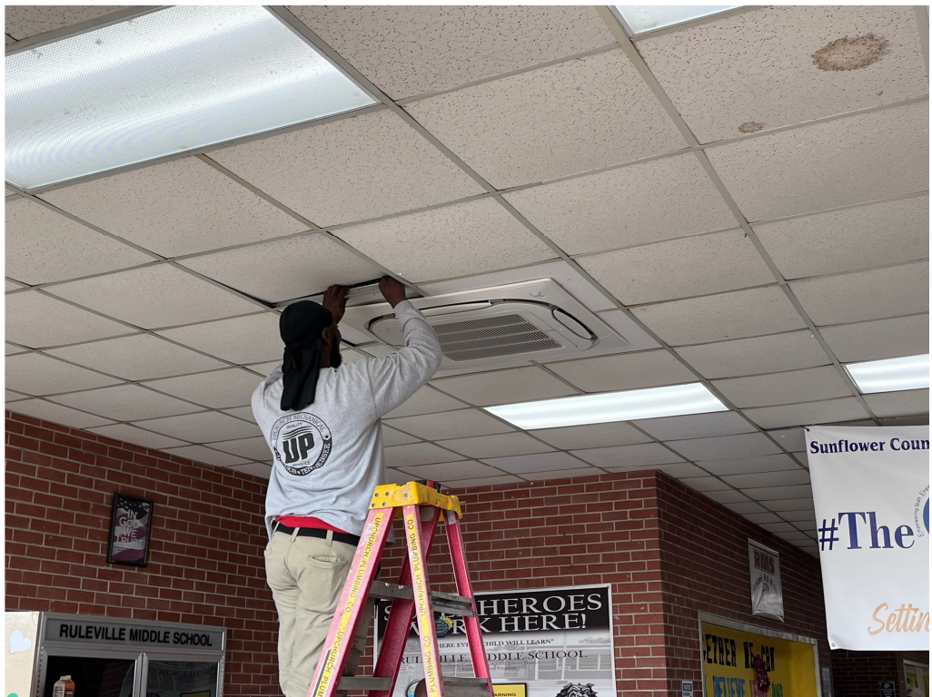
Figure 12 – Cassette location at Ruleville Middle Lobby
