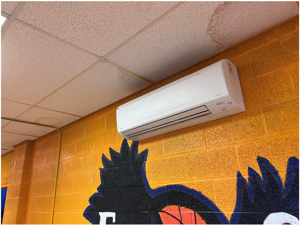
Figure 9 – Typical install at front lobby of Gym at Drew Hunter
