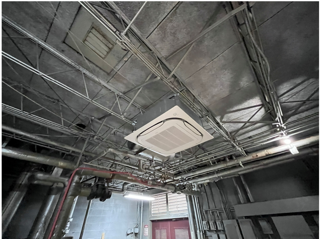
Figure 15 – Utility at Ruleville Middle cassette hung
