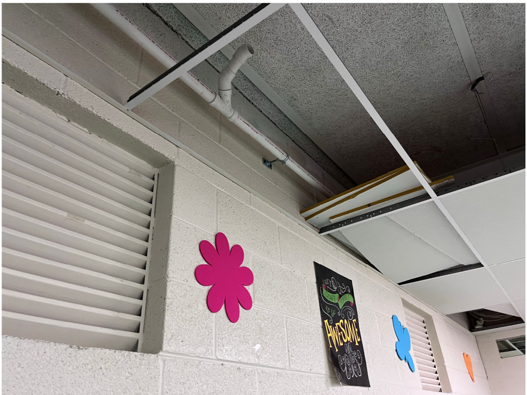
Figure 2 – Condensate Lines for cassettes above ceiling at Drew Hunter
