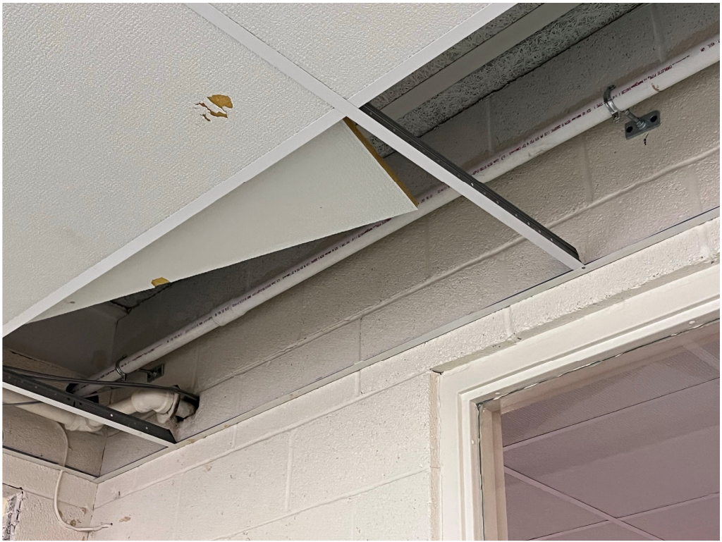
Figure 3 – Condensate Lines for cassettes above ceiling at Drew Hunter
