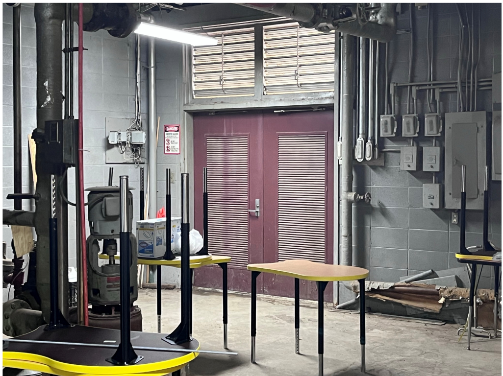
Figure 16 – Ruleville Middle Utility Room needs insulation if boiler no longer in use
