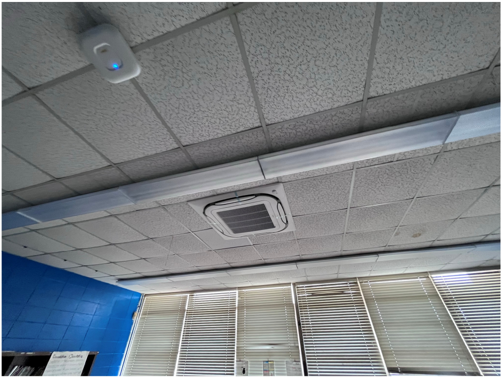
Figure 13 – Cassettes in Ruleville Middle are installed offset to avoid line of lighting
