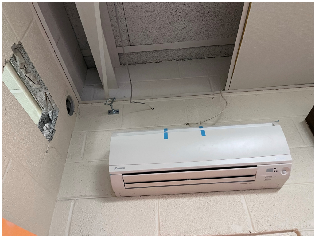
Figure 8 – Fresh air duct may pose servicing hazard at this location in Drew Hunter Teachers Lounge
