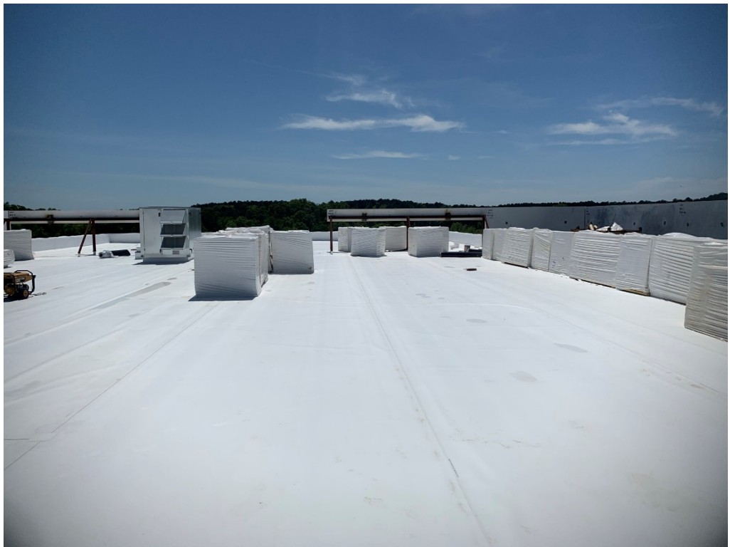
Figure 26 – Bare Decking on other Side of roof insulation stacks
