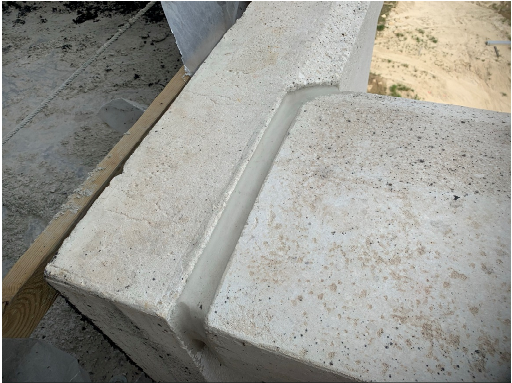
Figure 13 – Example of a good caulk line to Balcony
