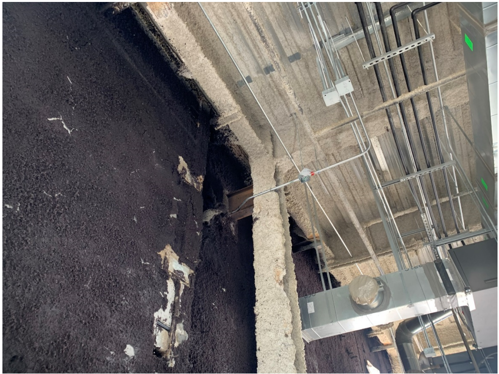
Figure 17 – Structural steel exposed without fire proofing
