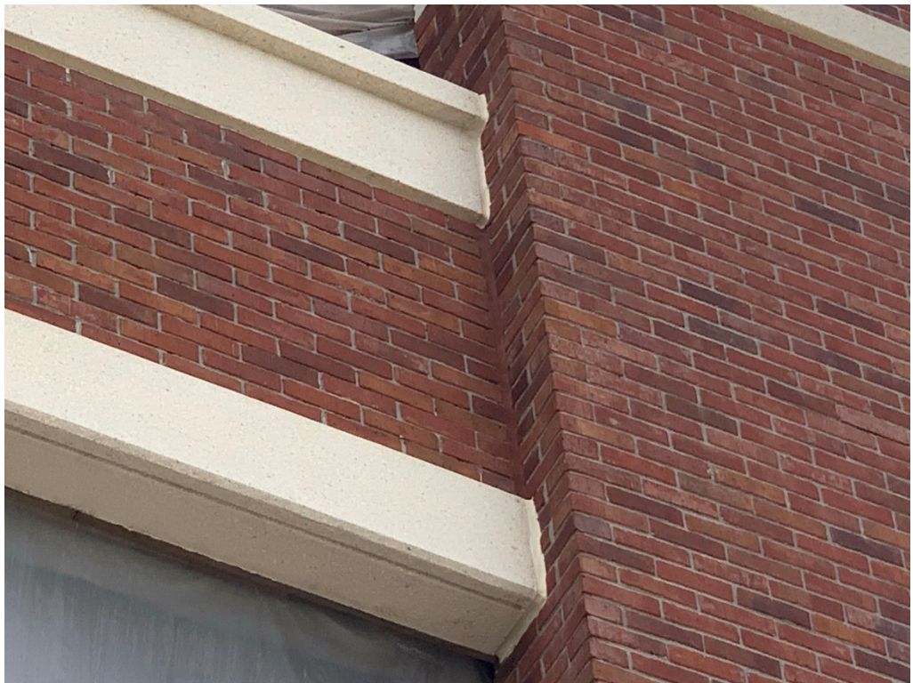
Figure 6 – Sealant work here is not satisfactory
