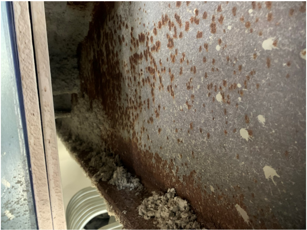
Figure 19 – Structural steel exposed without fire proofing (boxed in at north stair well by installed drywall)
