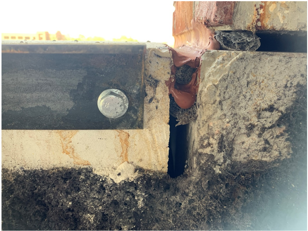
Figure 9 – Example of double Sealant (horizontal joint still needs to be removed and double sealed)
