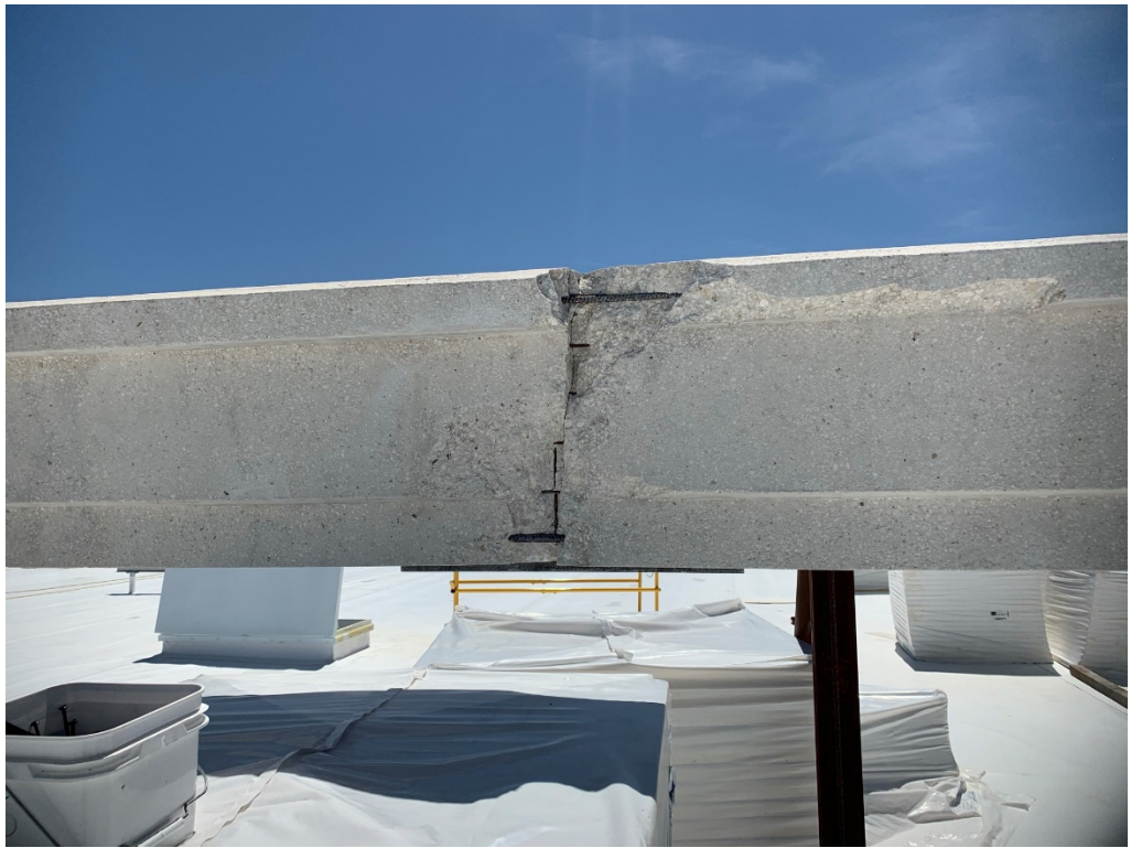
Figure 25 – Damaged Precast at Return over Roof
