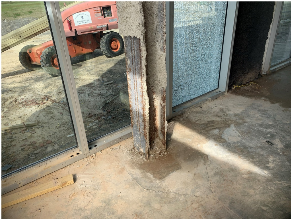
Figure 16 – Example of Degradation of Fire proofing due to weather
