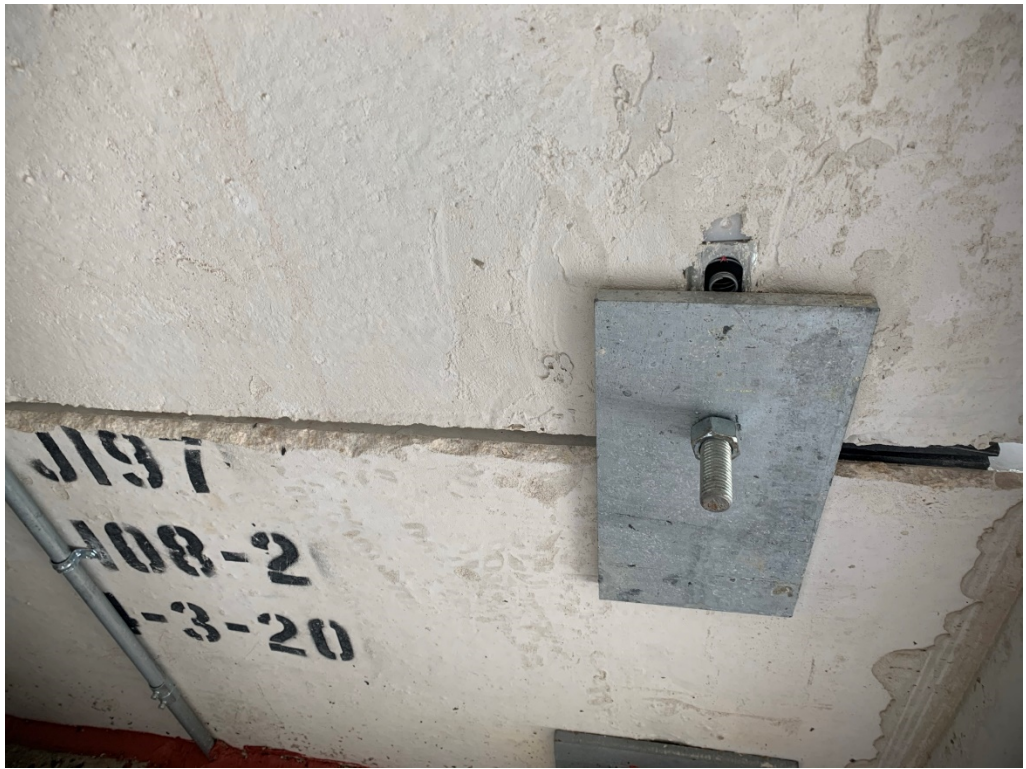
Figure 11 – Plate Missing Weld Plate (solution?)
