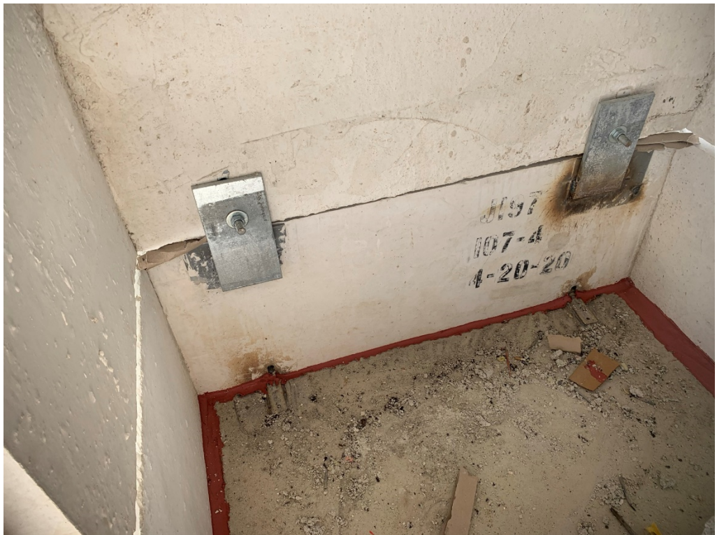
Figure 10 – Plate Missing Weld on left
