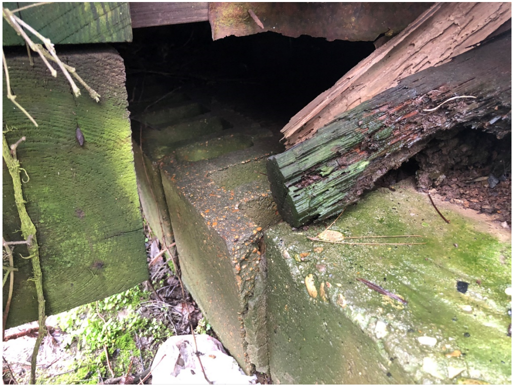
Figure 9 – Un-mortared blocks at slab to east of wash bay (concrete floor on interior)
