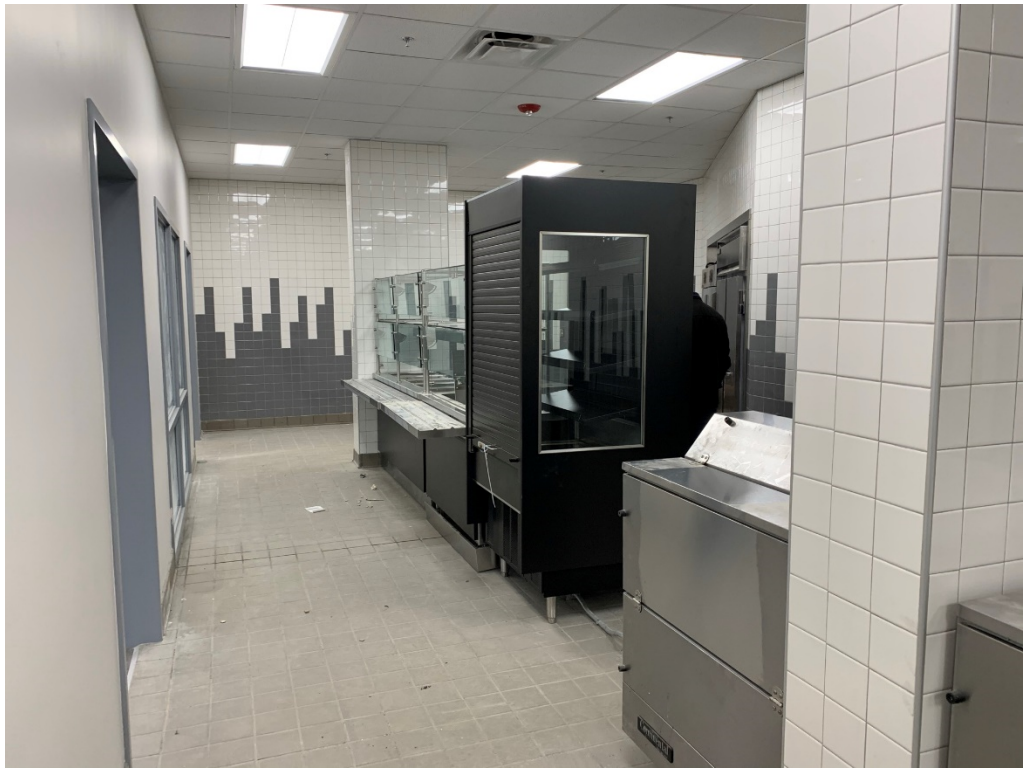
Figure 17 – Kitchen Equipment Installed
