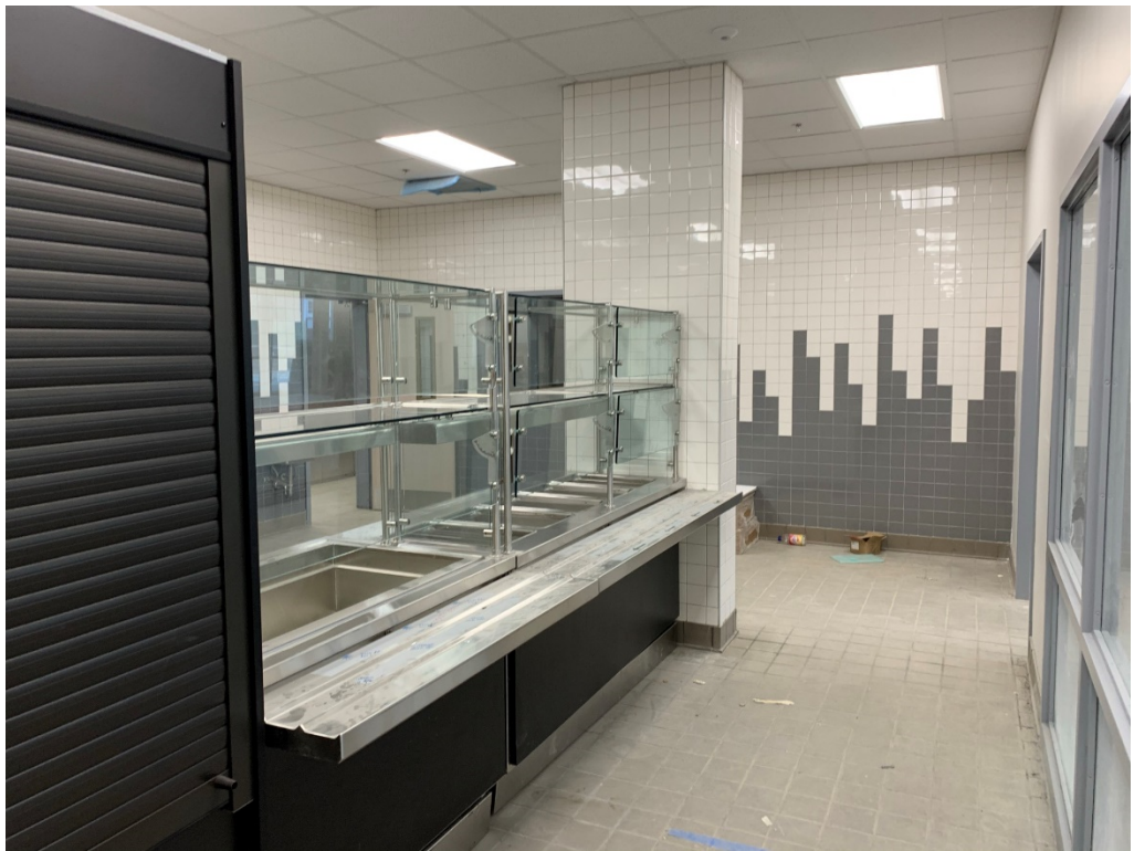
Figure 16 – Kitchen Equipment Installed
