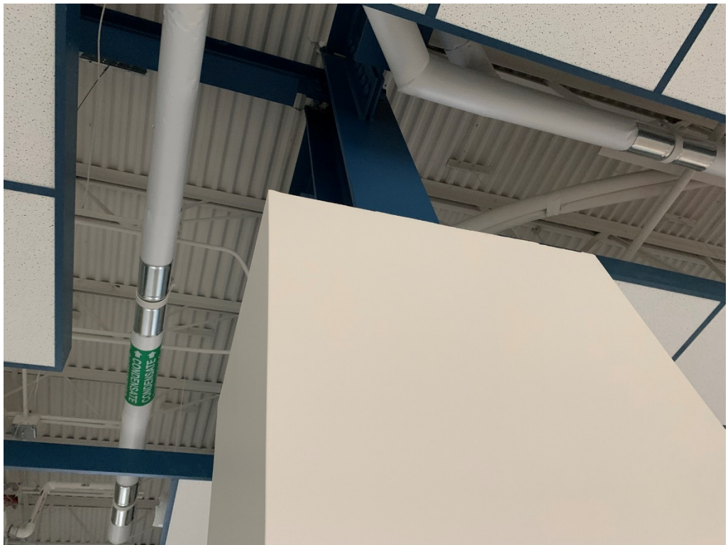
Figure 8 – Tops of all Columns need to be straight and finished smooth
