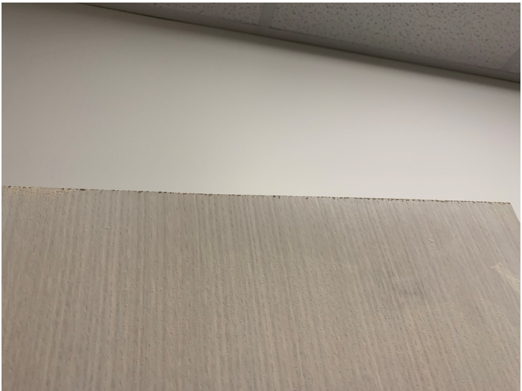
Figure 10 – Field Cuts at doors need to be finished
