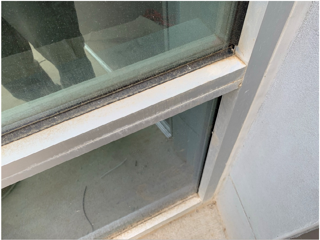
Figure 21 – There are Gaps in Gasketing around windows that need to be filled
