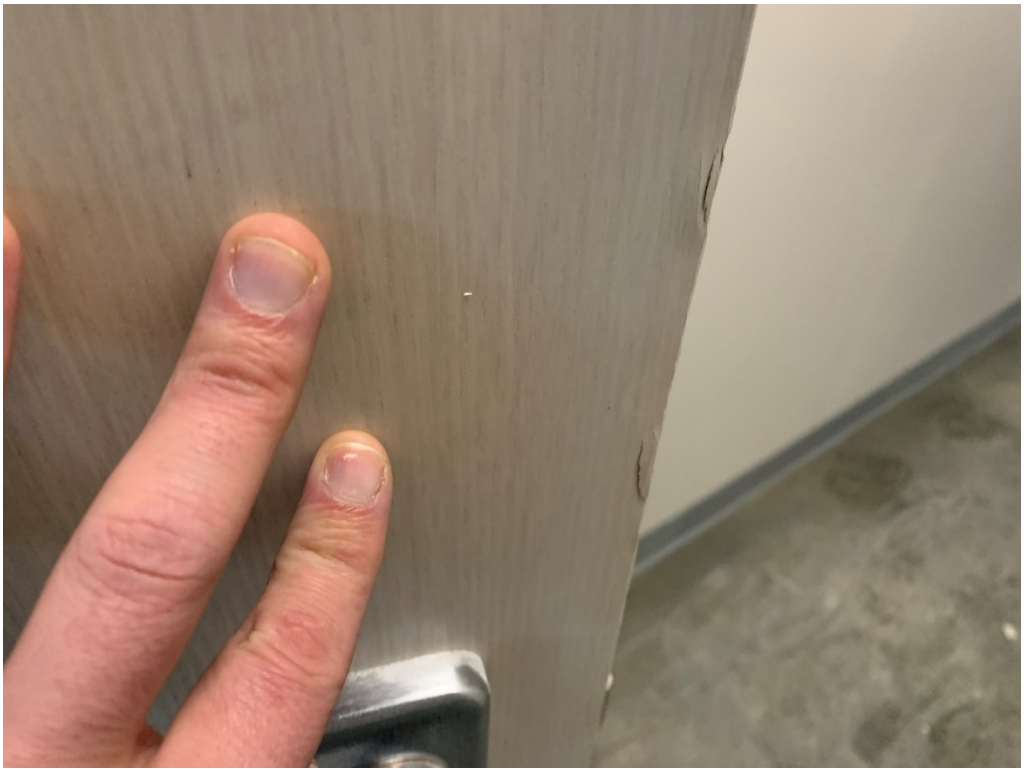
Figure 9 – Damage at New Door Panels in Administration Offices
