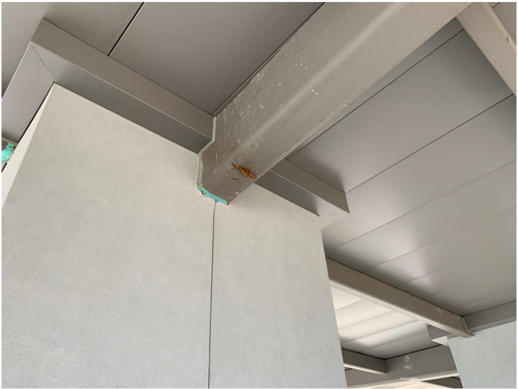
Figure 5 – Awning at drop off leaks and needs to be sealed and repainted where damaged
