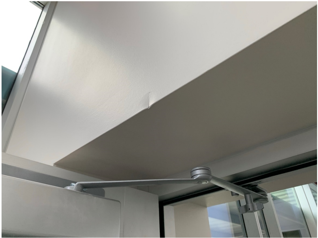
Figure 7 – Damage Noted North Entry
