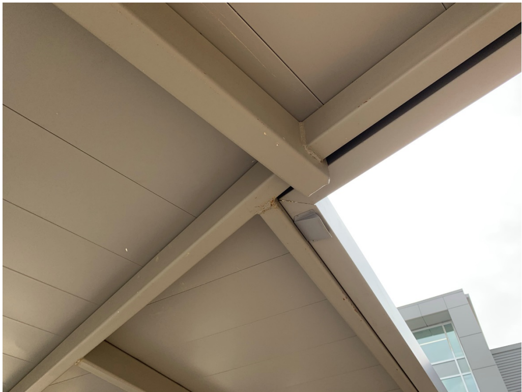
Figure 4 – Divertors at Awning do not Match in color and need to be painted to match
