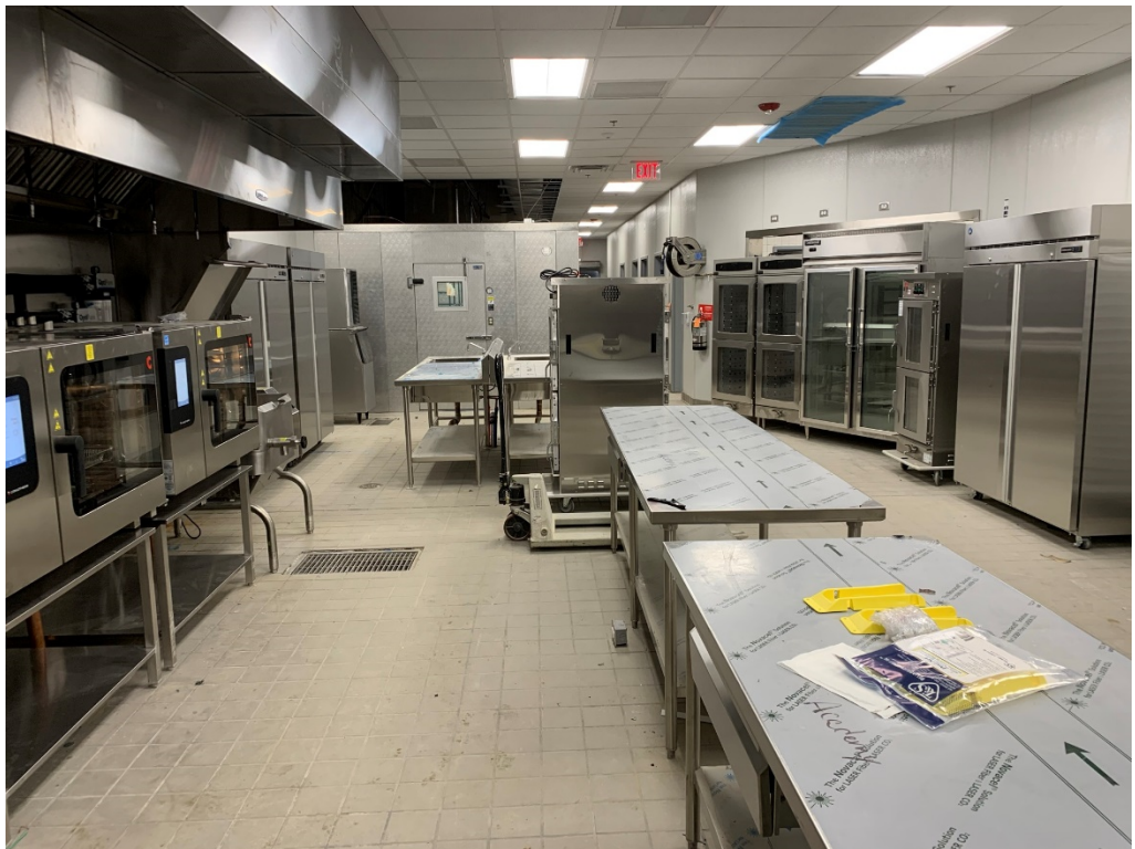
Figure 18 – Kitchen Equipment Installed
