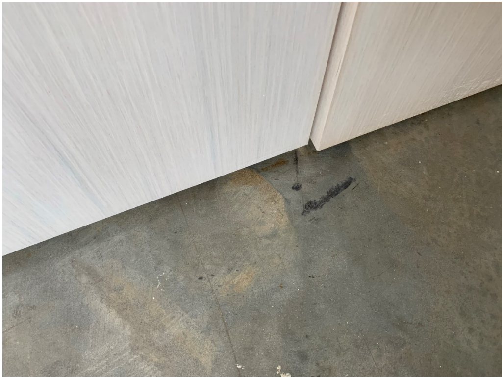
Figure 13 – Installed Double Doors (out of square and need adjustment for proper functionality and aesthetic)
