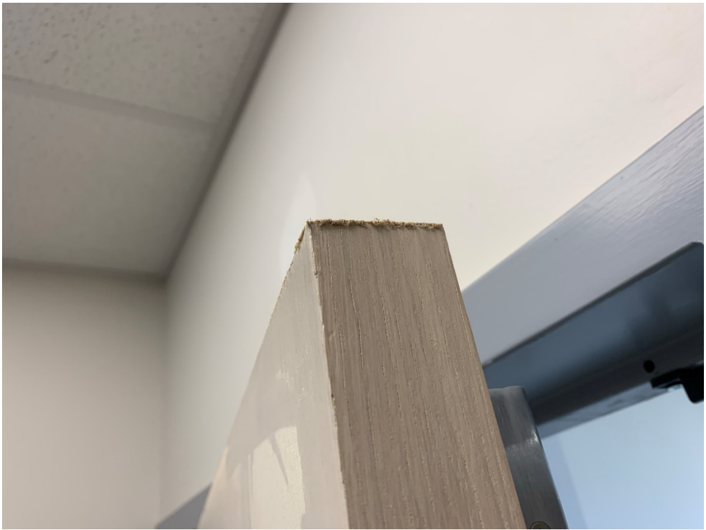
Figure 9 – Poor Carpentry at Door where cut due to Out of Square Installation
