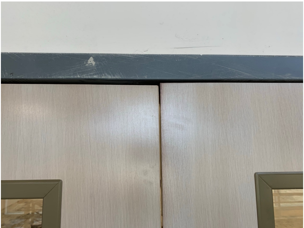
Figure 10 – Installed Double Doors (out of square and need adjustment for proper functionality and aesthetic)
