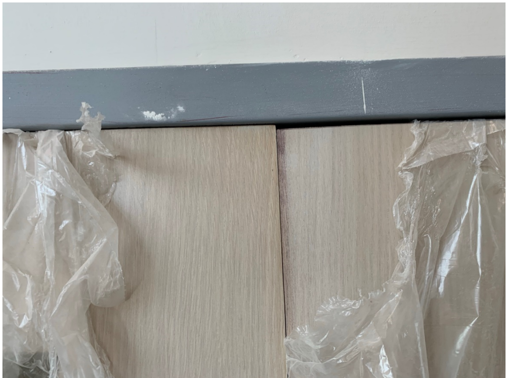
Figure 12 – Installed Double Doors (out of square and need adjustment for proper functionality and aesthetic)
