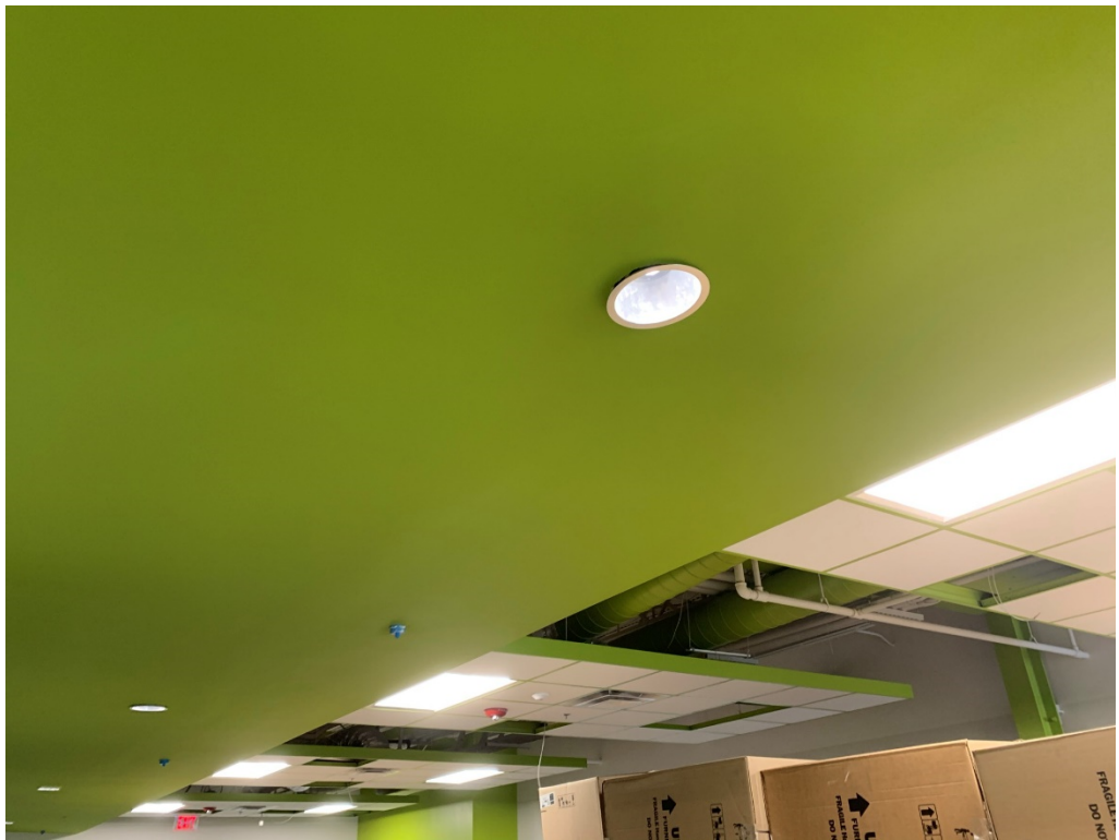
Figure 6 –Finish Electrical is Ongoing (note to check all can lights for flush installation at drywall)
