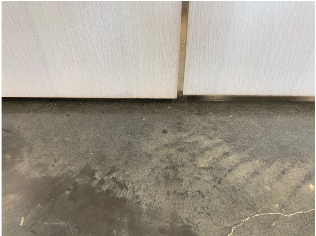
Figure 11 – Installed Double Doors (out of square and need adjustment for proper functionality and aesthetic)
