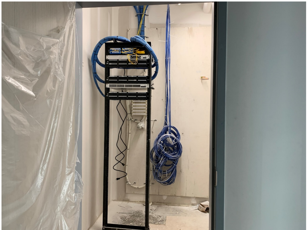
Figure 8 – Communication Cabling Installed
