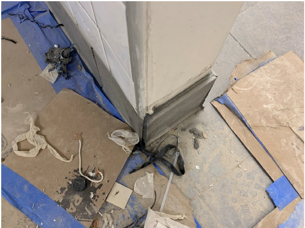
Figure 20 – Corner Tiles at base in several locations need correction (cut back wall tiles so that end tile does not create a larger shelf than is typical)
