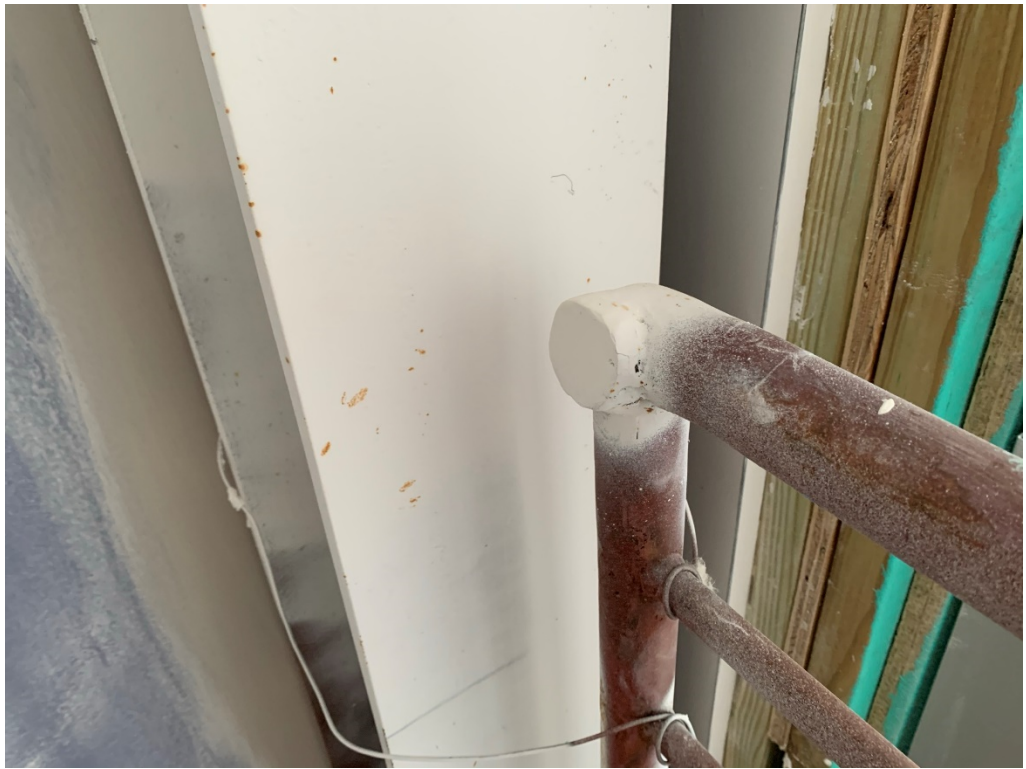
Figure 37 – Handrail that still need correction (cut section should be further cut back so that it looks like it was never there)
