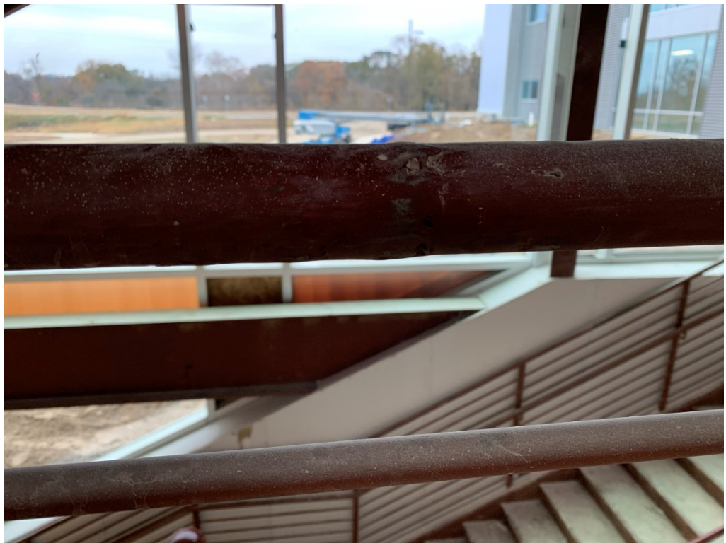
Figure 34 – Handrail that still need correction (built up weld need further grinding)
