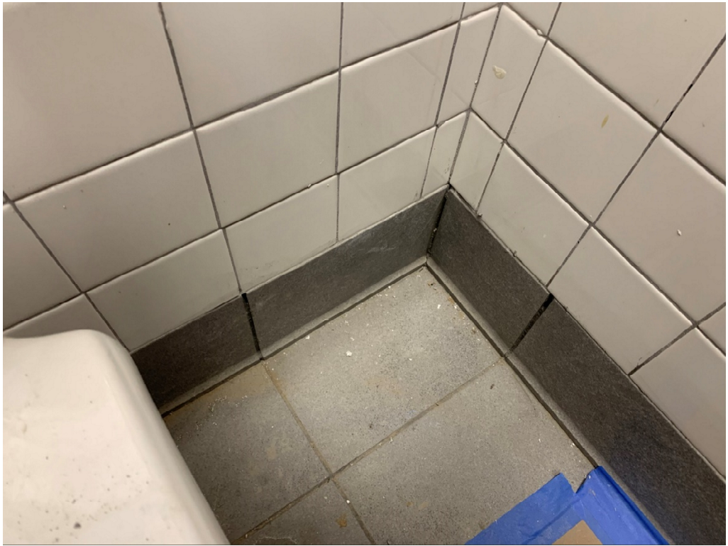
Figure 19 – Corner Tiles at base in several locations need correction (grout missing between base and upper tiles)
