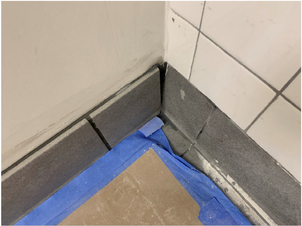
Figure 21 – Corner Tiles at base in several locations need correction (reinstall so they are square to each other)
