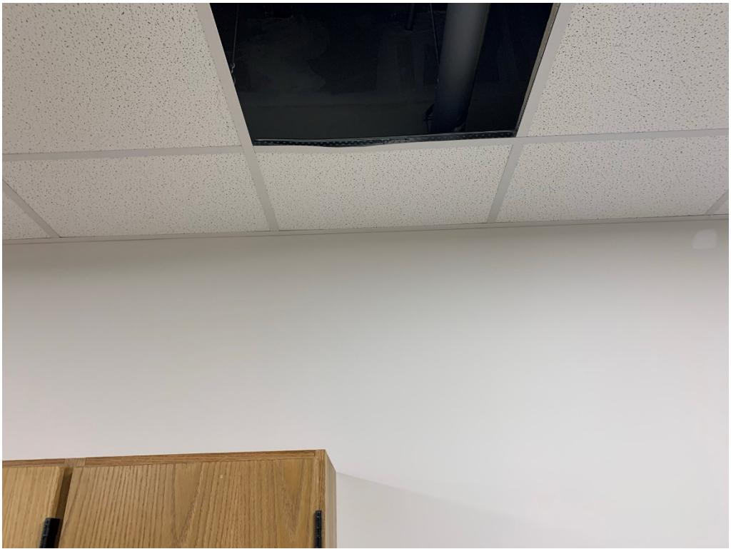
Figure 27 – Ceiling grid throughout has been damaged and will need replacing
