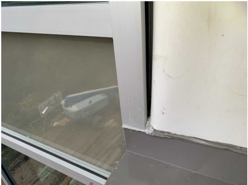
Figure 44 – Solid Storefront Jamb required for proper flashing at this section of roof; use of this style jamb creates refuge for water and/or insects
