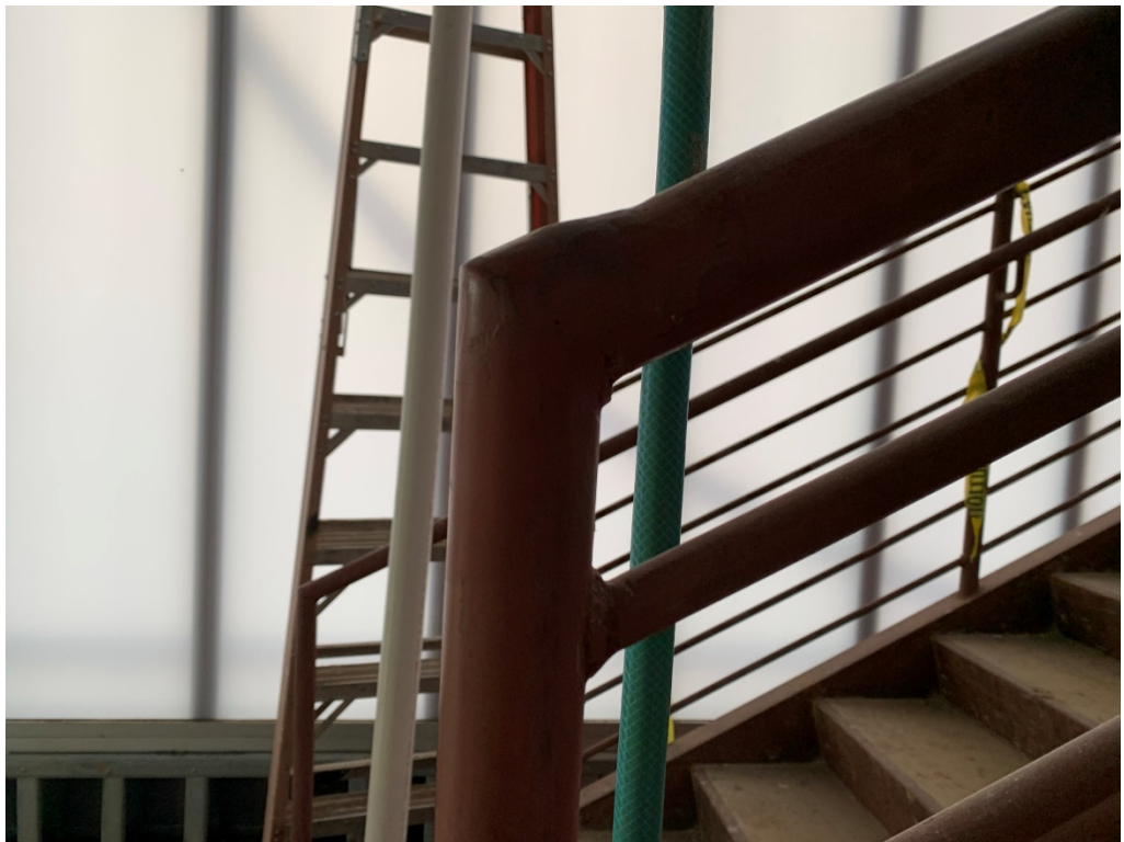
Figure 36 – Handrail that still need correction (dip in rail)
