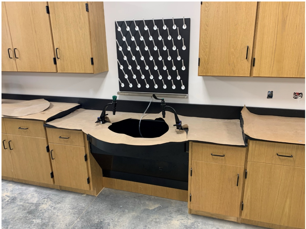
Figure 26 – Lab Fixtures installed
