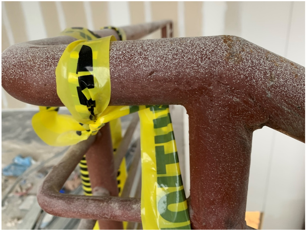
Figure 35 – Handrail that still need correction (mottling at weld)
