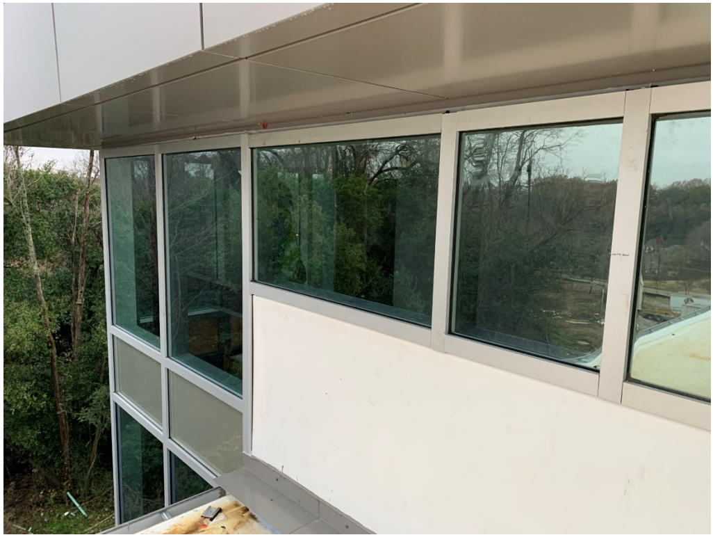
Figure 43 – Curtain Wall at South Central Roof; this junction is not properly flashed and just over the edge of roof, bare wood is showing which needs metal flashing as covering
