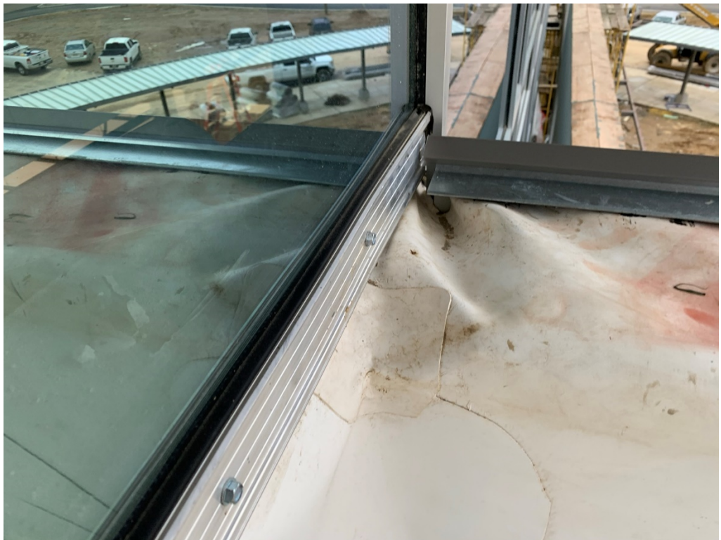
Figure 42 – Fold in TPO creates well for water to collect and drain into wall cavity; this work needs correction
