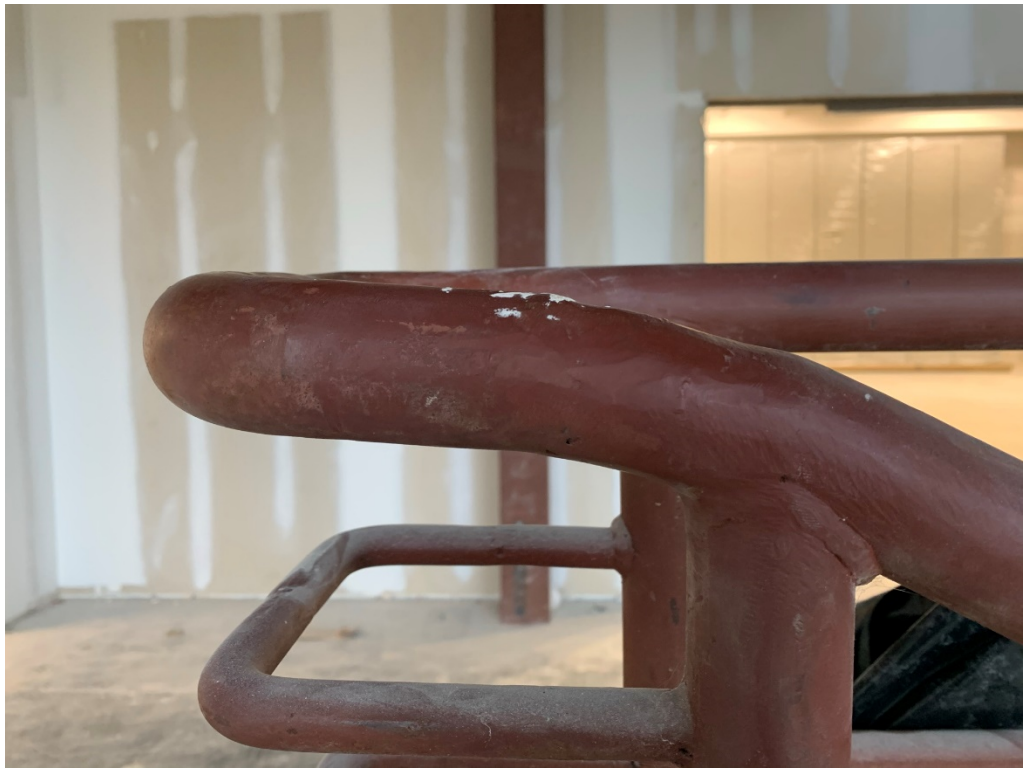
Figure 33 – Handrail that still need correction (dip in rail needs correction)
