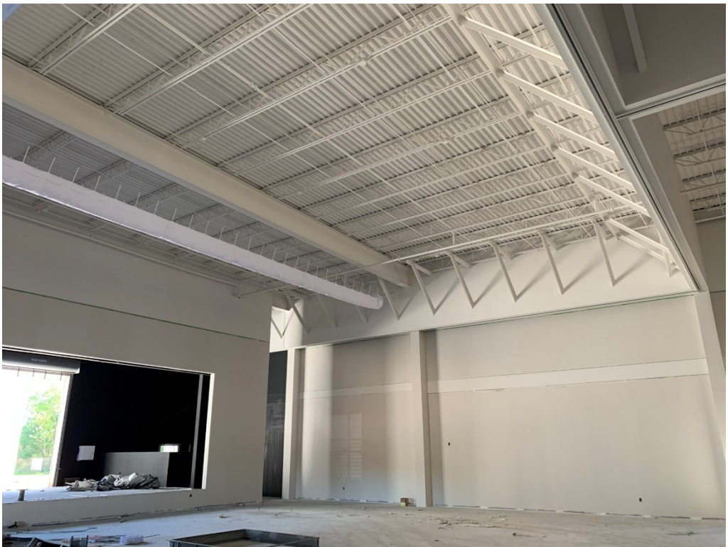
Figure 18 – Paint at Gym
