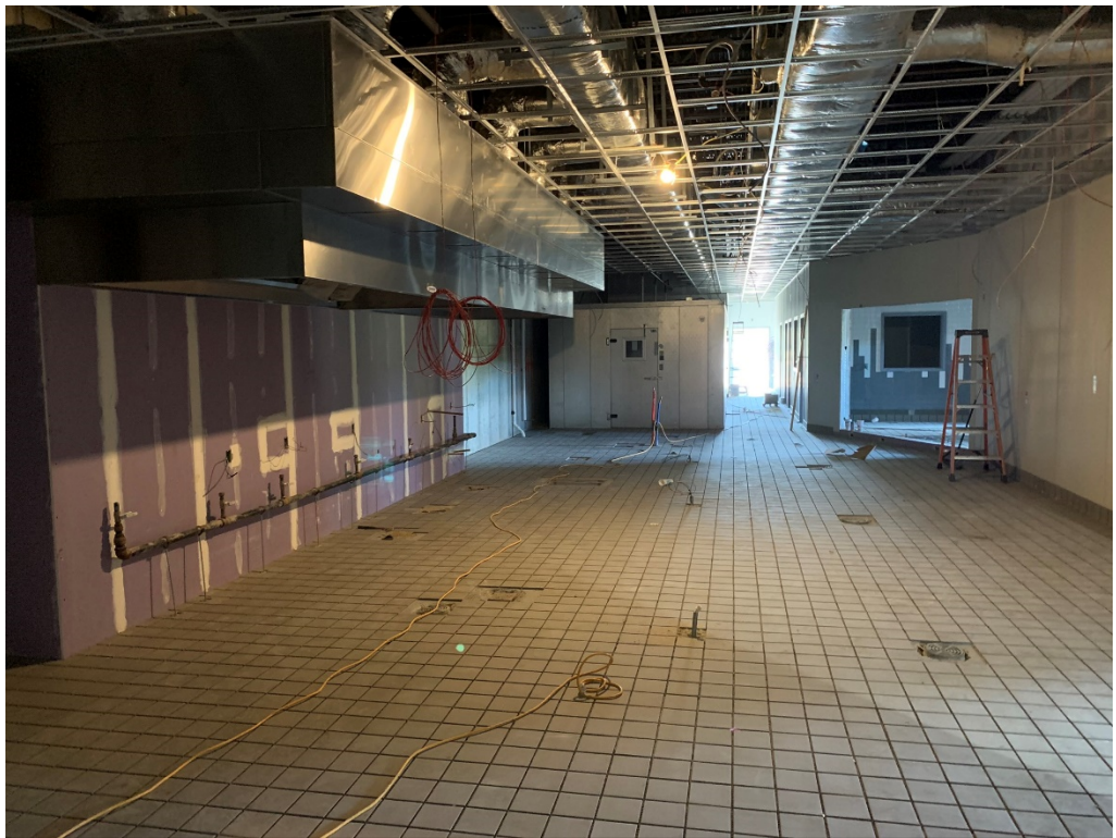
Figure 16 – Ceiling Grid & Tile at Kitchen
