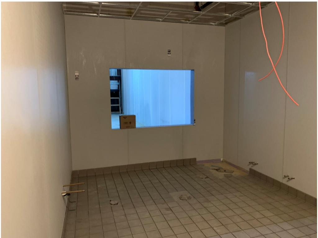
Figure 14 – FRP at Dish Wash
