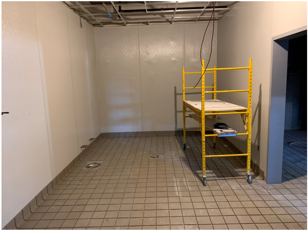
Figure 15 – FRP at Dish Wash
