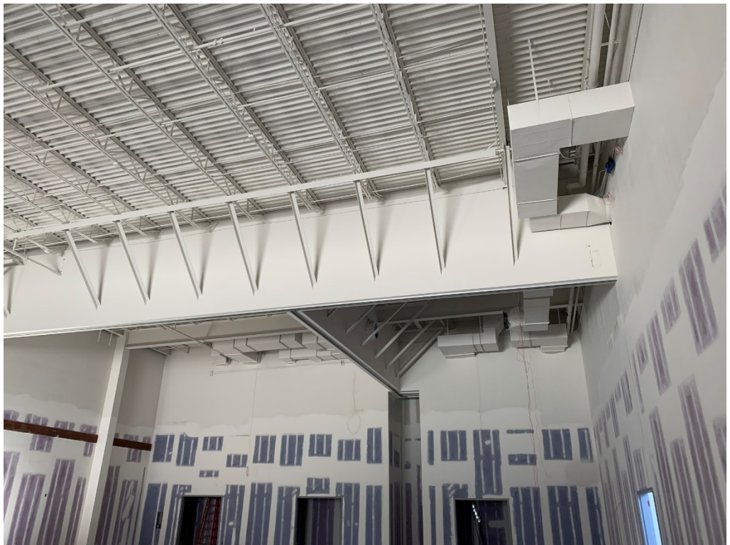
Figure 20 – Paint @ Gym Ceilings
