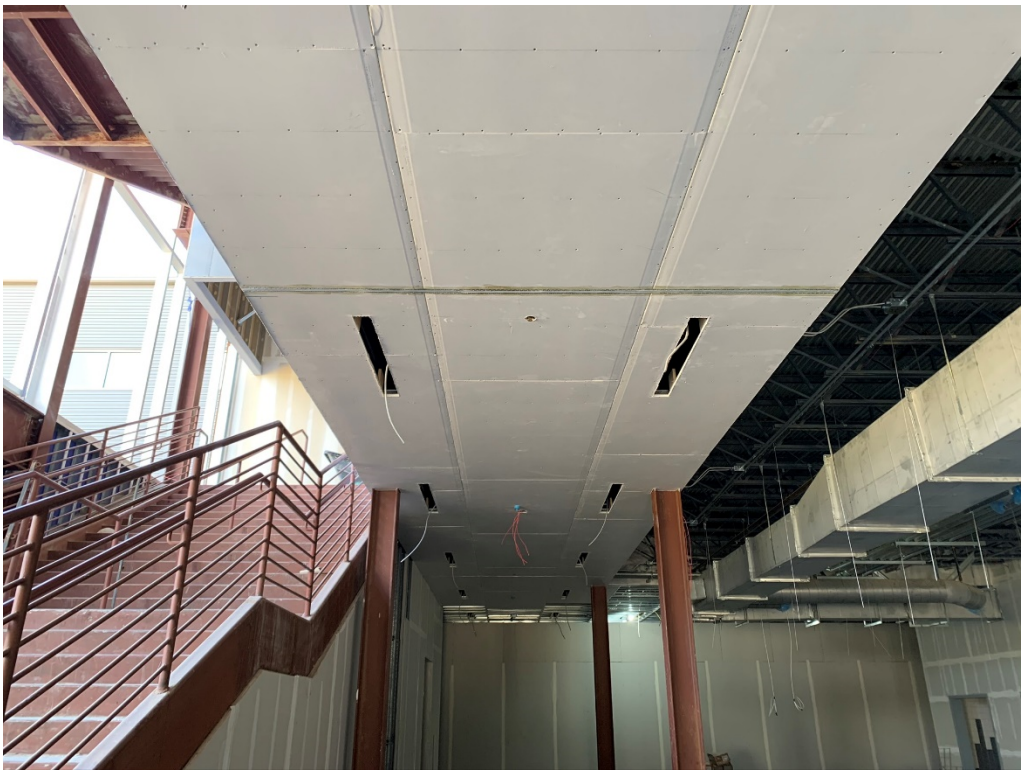
Figure 18 – Hard Ceiling at Cafeteria Stair Connection
