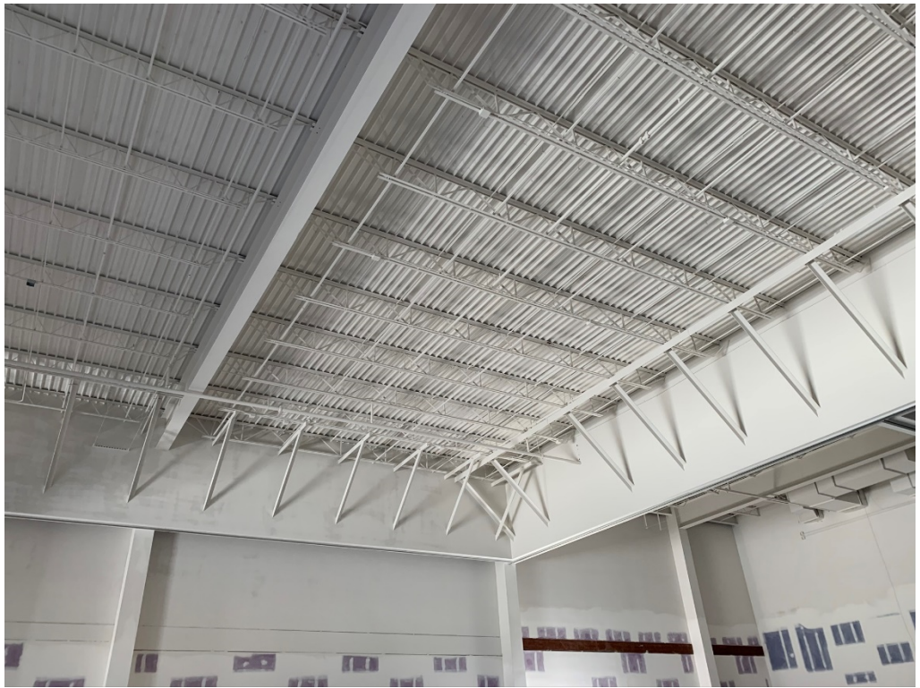
Figure 19 – Paint @ Gym Ceilings
