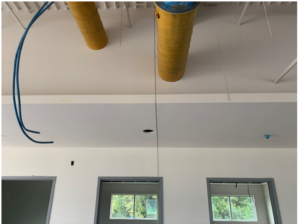
Figure 20 – Paint and Drywall at Versatile Teaching Space 210
