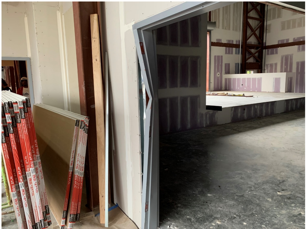
Figure 10 – Damaged Door Jamb at Gym
