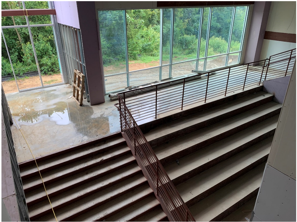
Figure 17 – Glazing Impeding Drywall Installation Here
