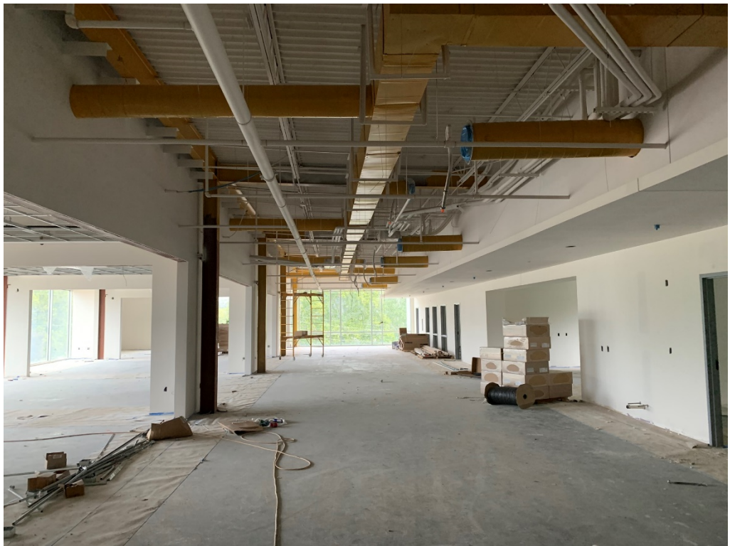
Figure 18 – Paint at 3 rd Floor Versatile Teaching Space 210
