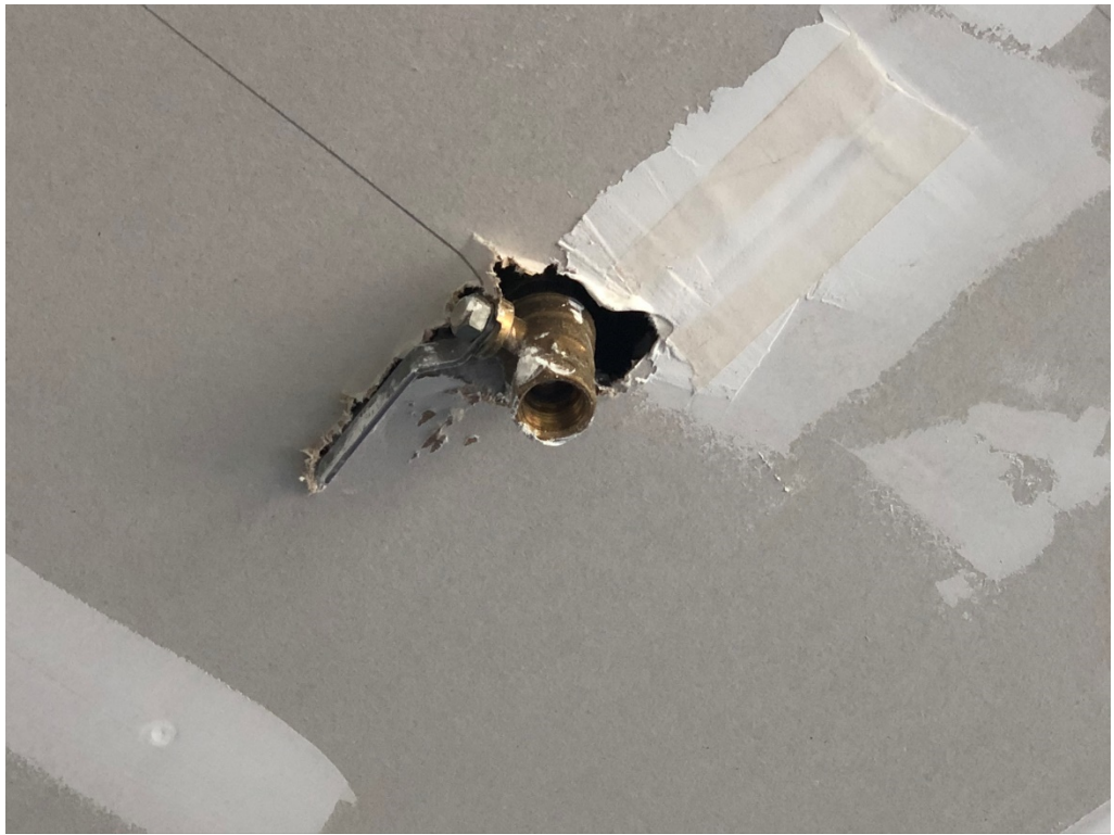
Figure 25 – Conflict with Cut Off (Is this a permanent installation?)
