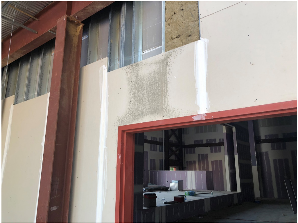
Figure 9 – Mildewed Drywall Panel Requires Remediation
