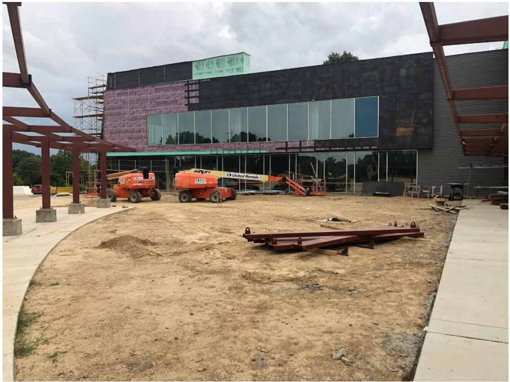
Figure 13 – North Elevation Metal Siding Installation is Ongoing; at the second level furthest panel to the right, glass is off colored and requires replacement
