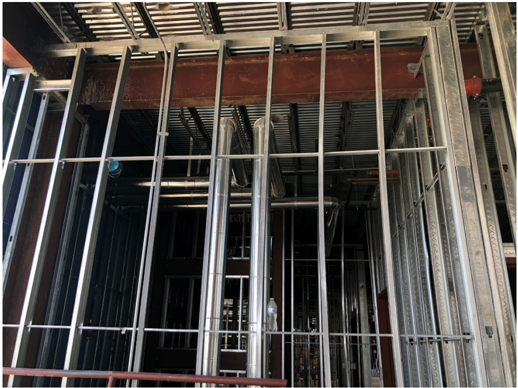
Figure 15 – Studs at 2 nd Floor Top of Stair Deformed; Reset Before Drywall Installation
