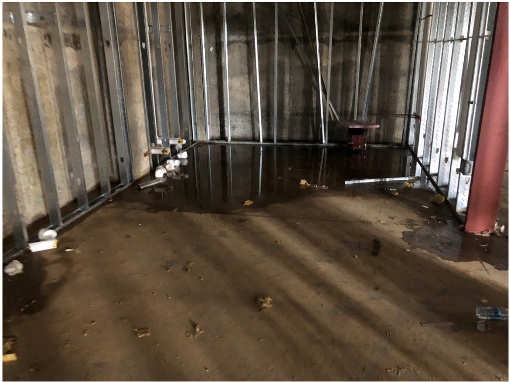
Figure 13 – Ponded water at Lower Level
