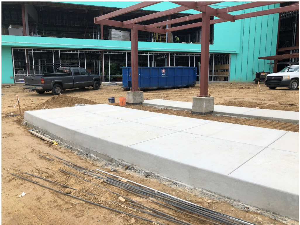
Figure 2 – Drop Off Concrete
