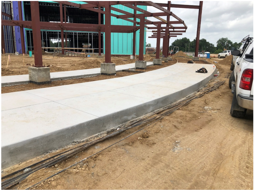
Figure 1 – Drop Off Concrete
