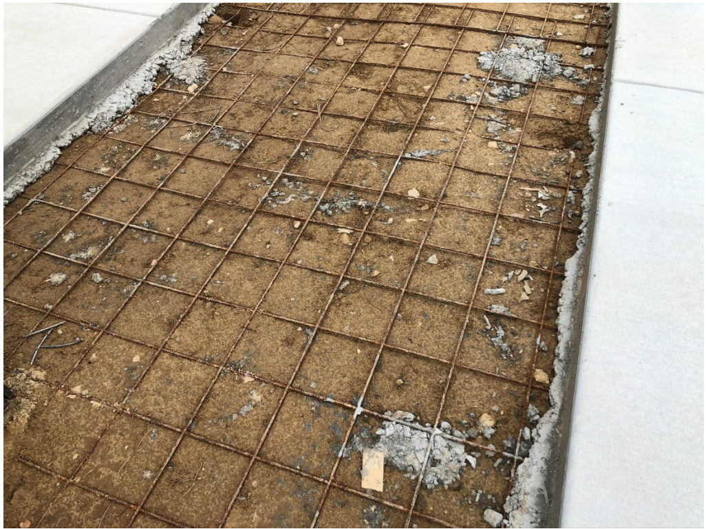
Figure 3 – Remesh at Sidewalk is Incorrectly Placed at the bottom of the Concrete
