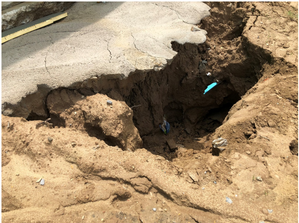
Figure 14 – Erosion at North Structure Continues to be an Issue
