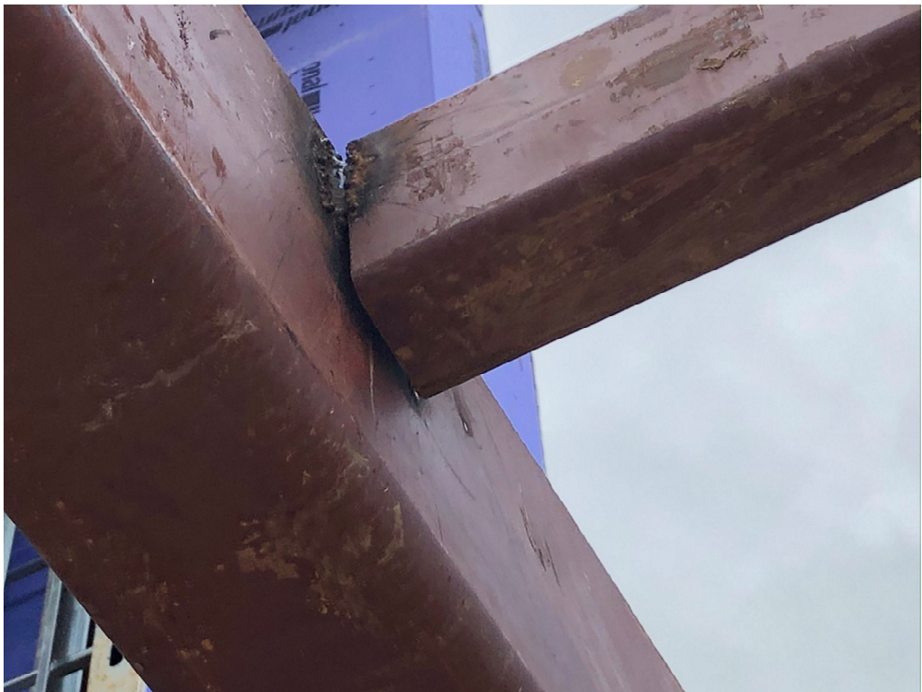
Figure 6 – Welds at Steel Canopy Should Be Continuous and Smooth Per S3.7
