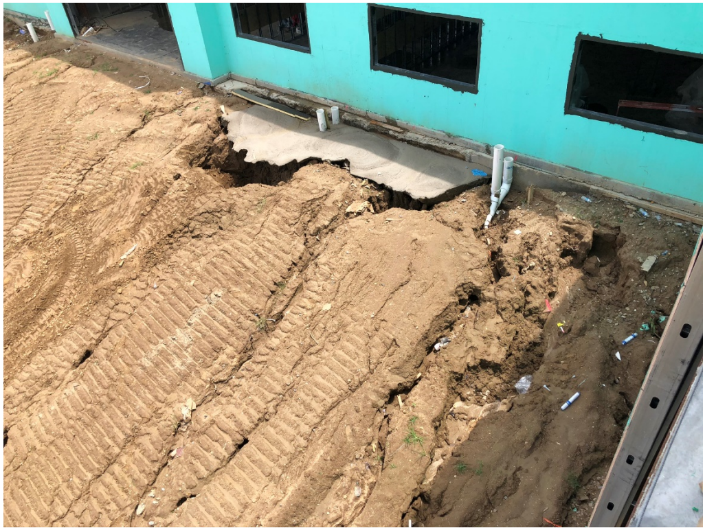
Figure 13 – Erosion at North Structure Continues to be an Issue
