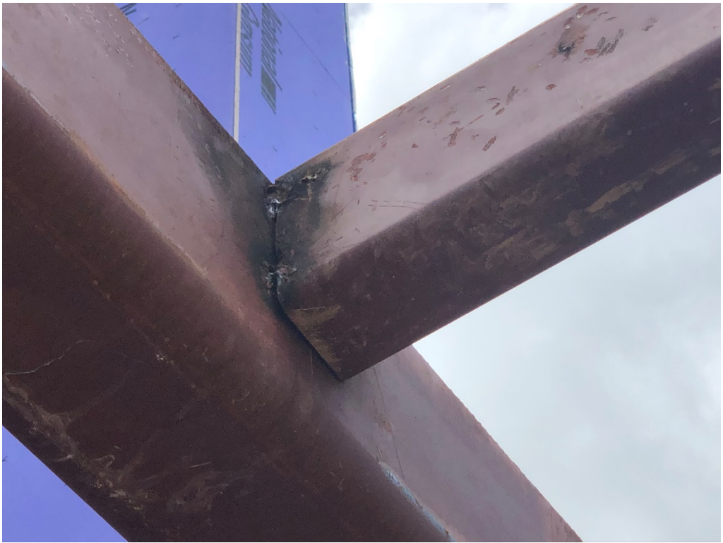
Figure 5 – Welds at Steel Canopy Should Be Continuous and Smooth Per S3.7
