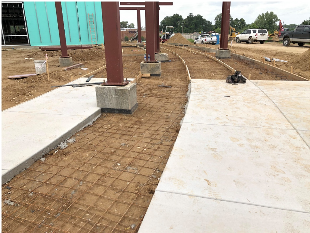
Figure 4 – Remesh Should be lifted to Center of Concrete or Floated Up during Install
