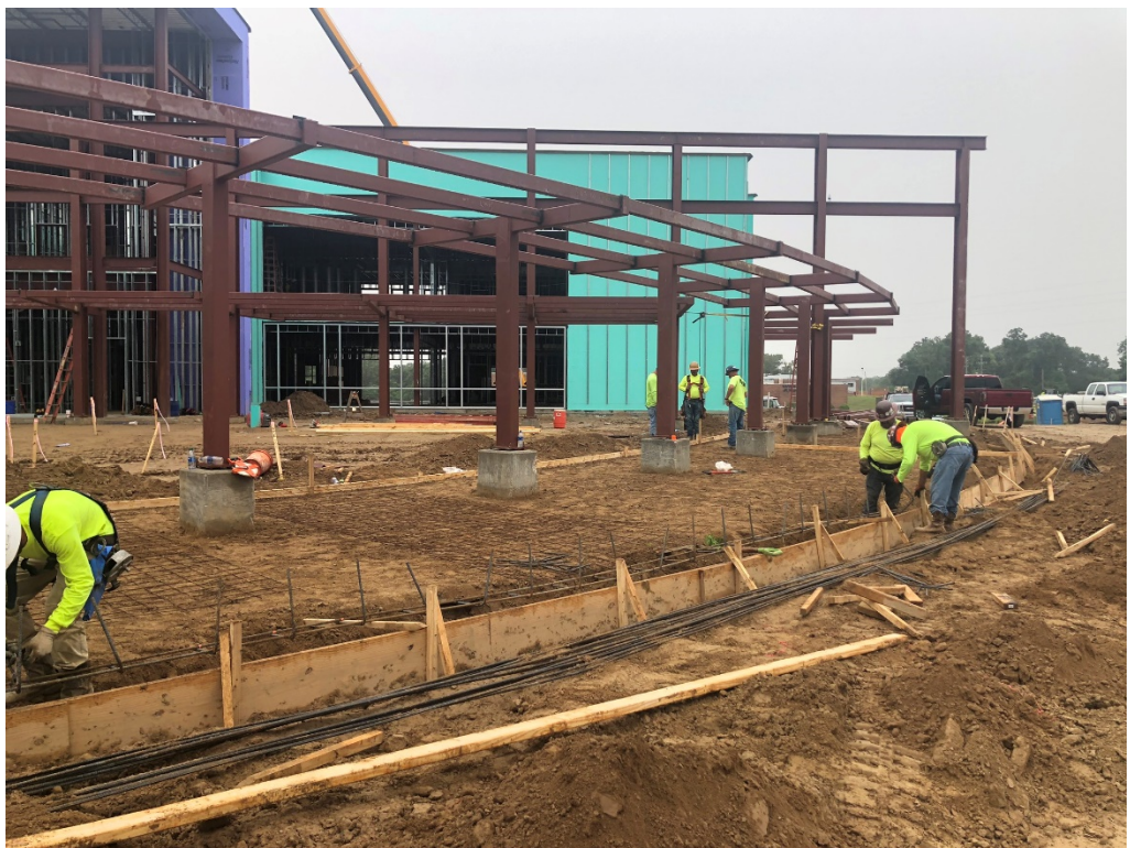
Figure 2 – Drop Off Concrete Reinforcing
