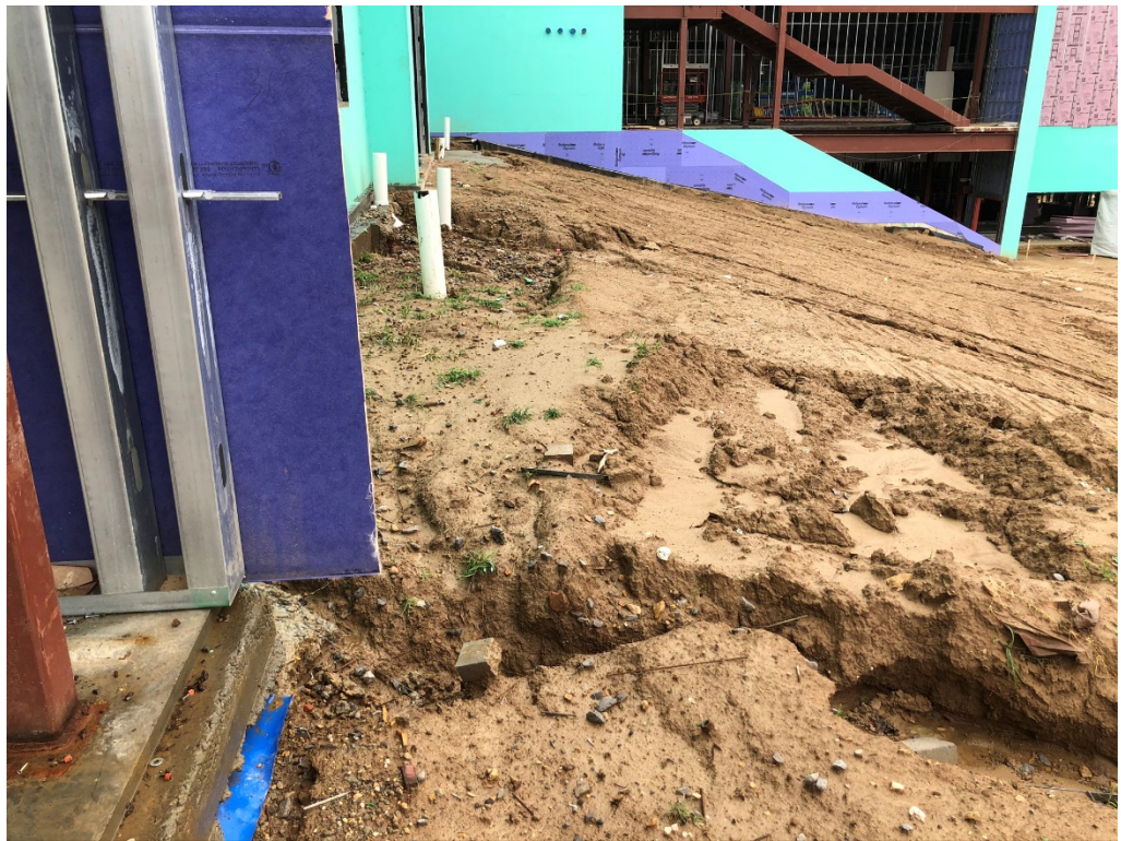
Figure 20 – Note Concrete @ Eroded area in Rear of Image
