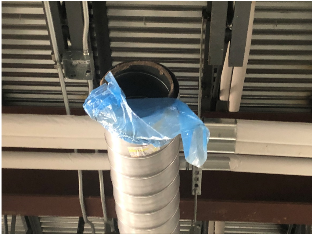
Figure 9 – Not Typical, but there was one uncovered Duct in East Building Lower Level
