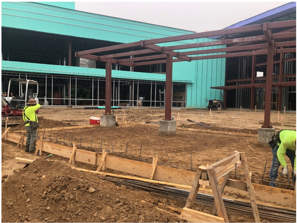
Figure 1 – Drop Off Concrete Reinforcing
