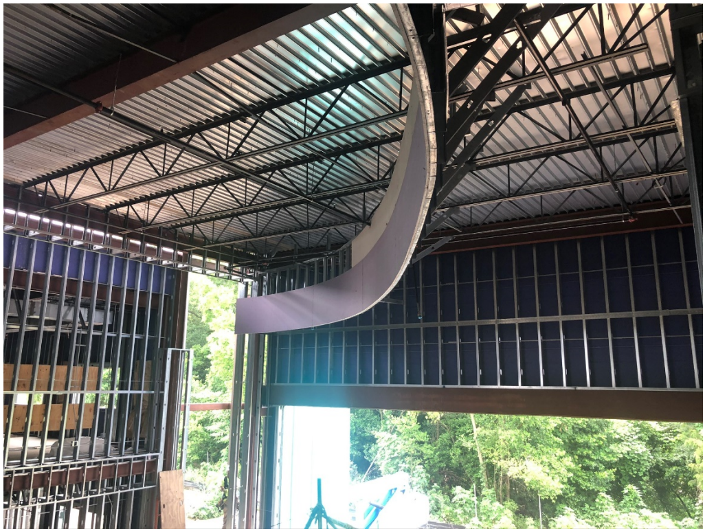
Figure 14 – Straight Portion of Curve Appears to be Corrected
