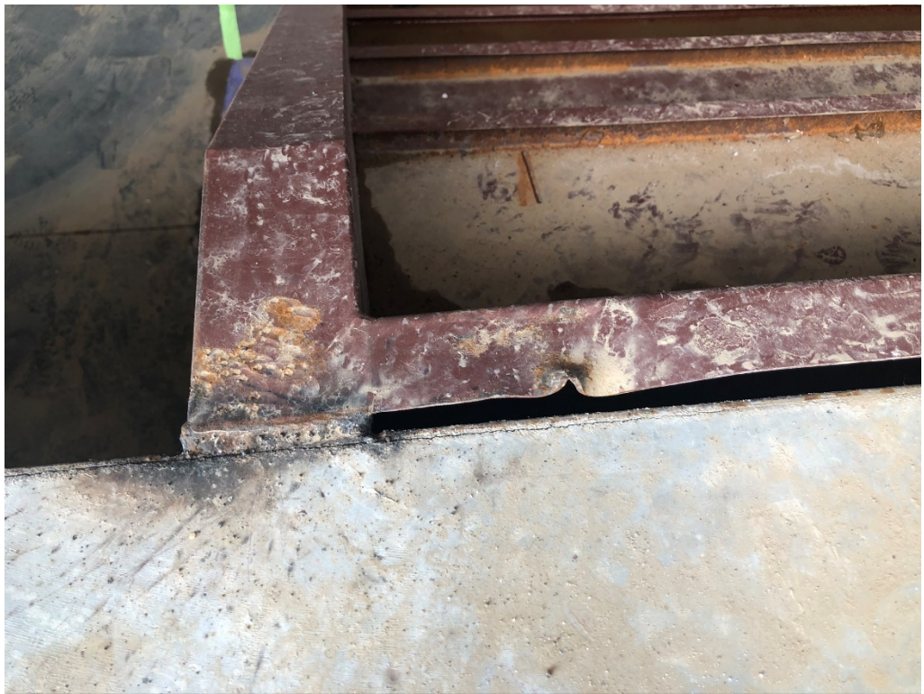
Figure 8 – Damage Noted at Metal Pan Stair
