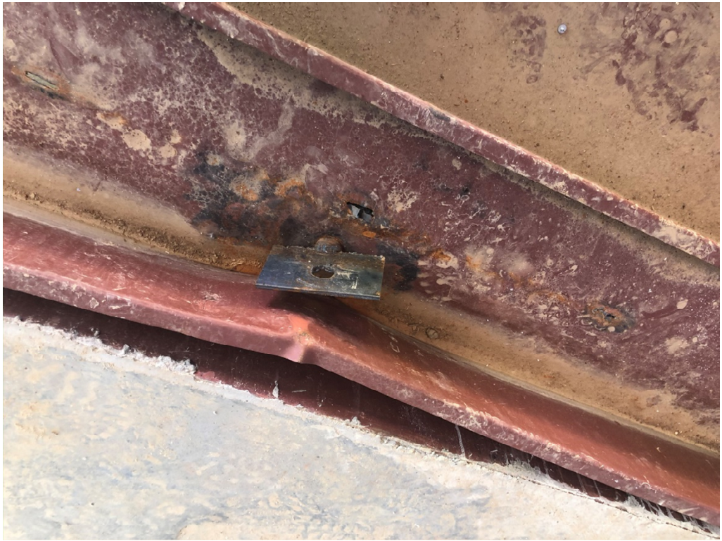
Figure 9 – Damage Noted at Metal Pan Stair
