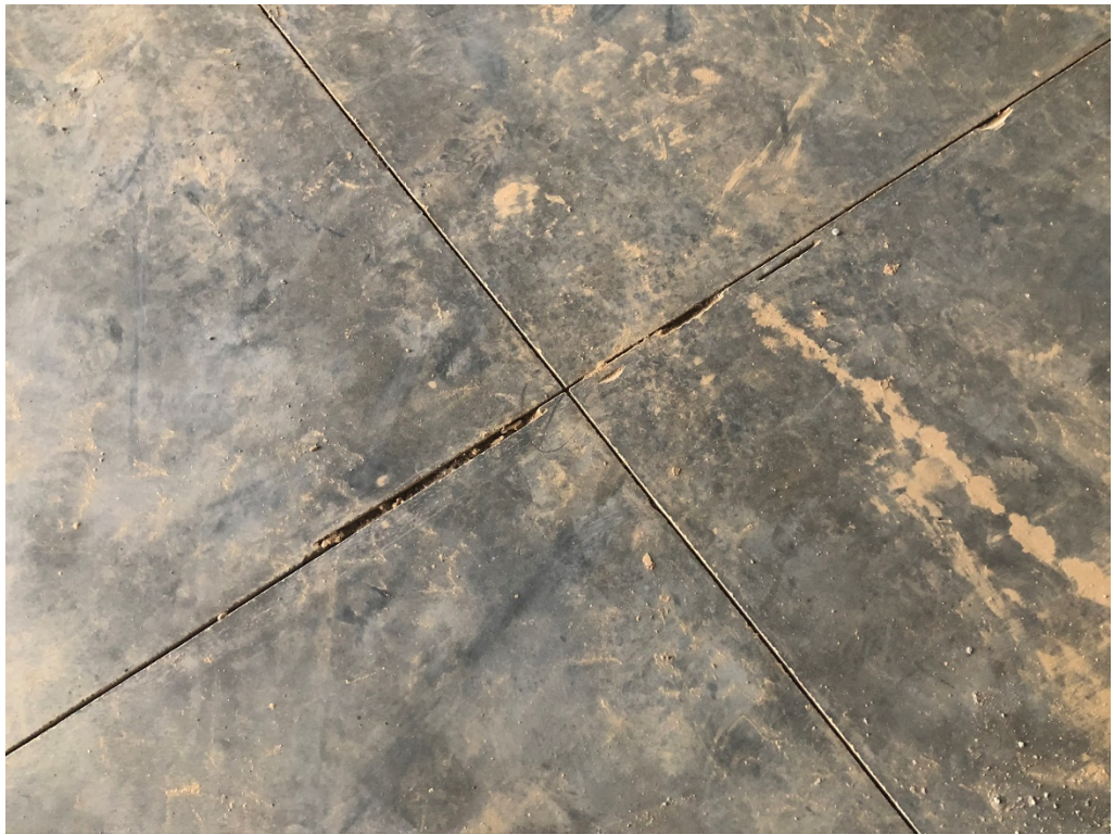
Figure 11 – Bad Saw Cut; Anyway to repair?
