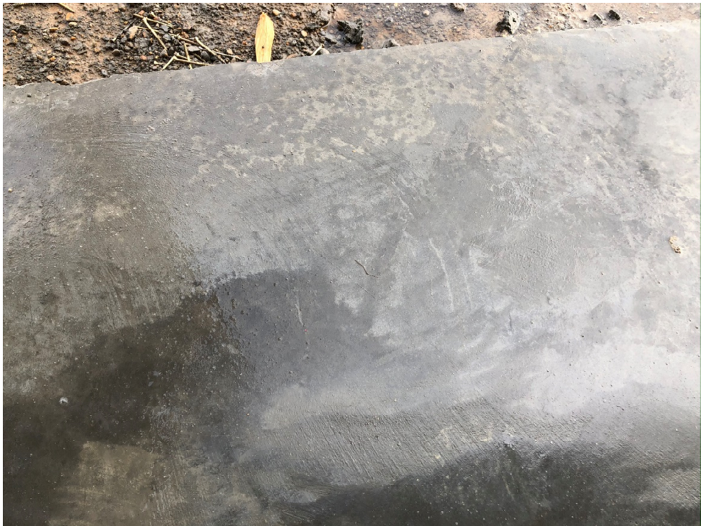
Figure 8 – North Edge of Slab Not Troweled Smooth (near Stairwell)
