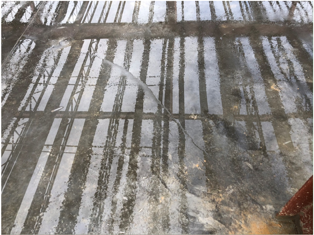
Figure 9 – Large Stress Crack @ Column NW of Room “Principal 104”
