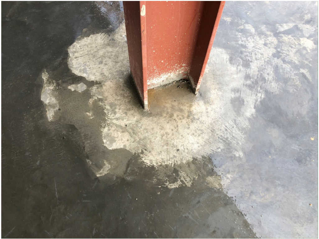
Figure 7 – Concrete @ North Column not troweled entirely smooth
