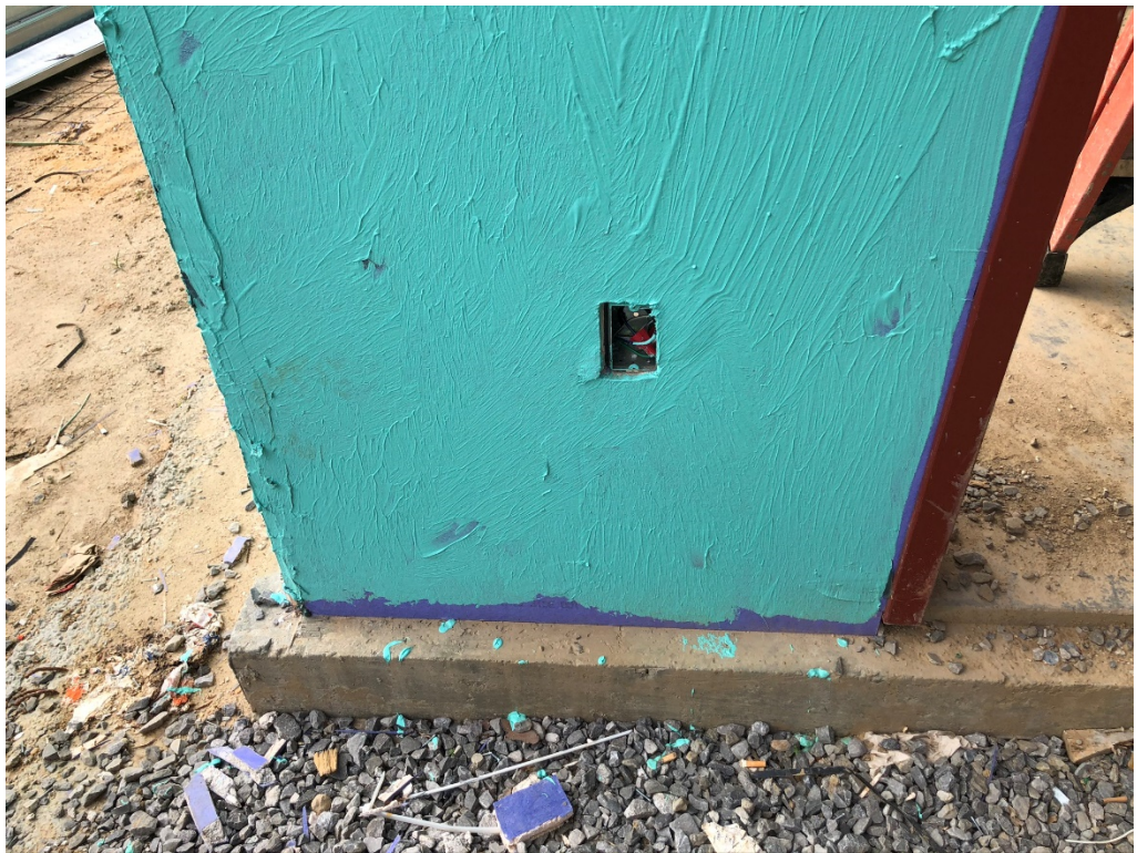
Figure 2 – Waterproofing touch up needed where smeared
