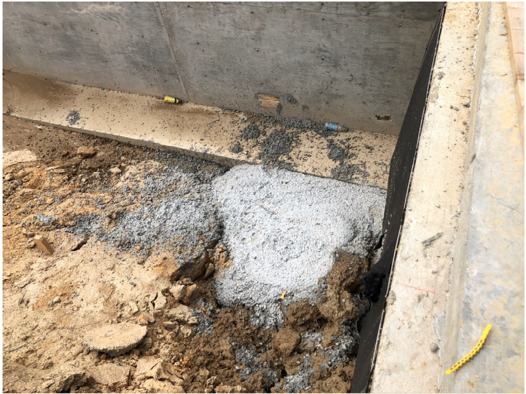
Figure 11 – Eroded area Filled with Concrete
