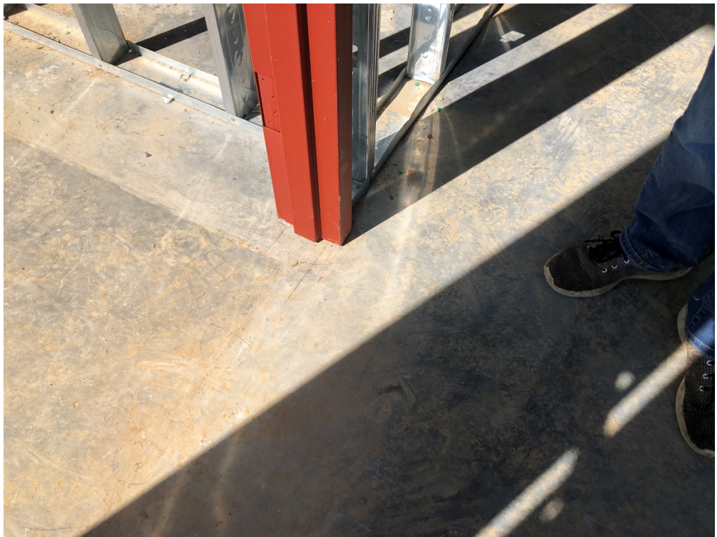
Figure 2 – Top Floor at East Section of Building where Concrete was poured after main slab showing stress crack and floor not entirely smooth and level here
