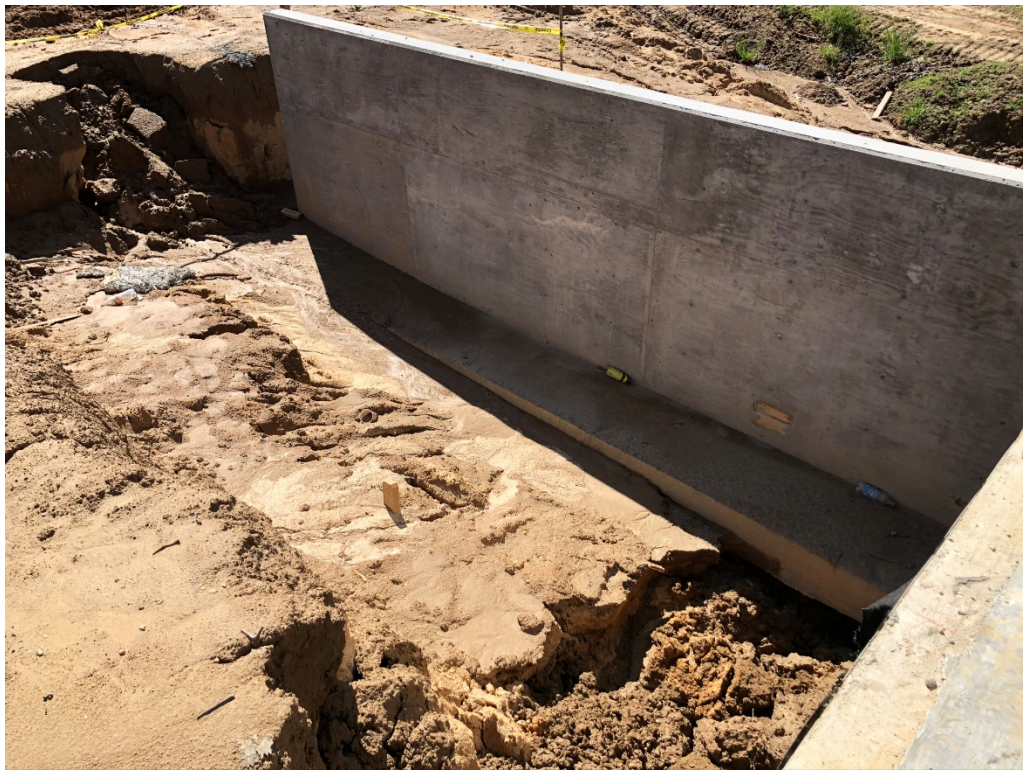
Figure 12 – Erosion under New Footing
