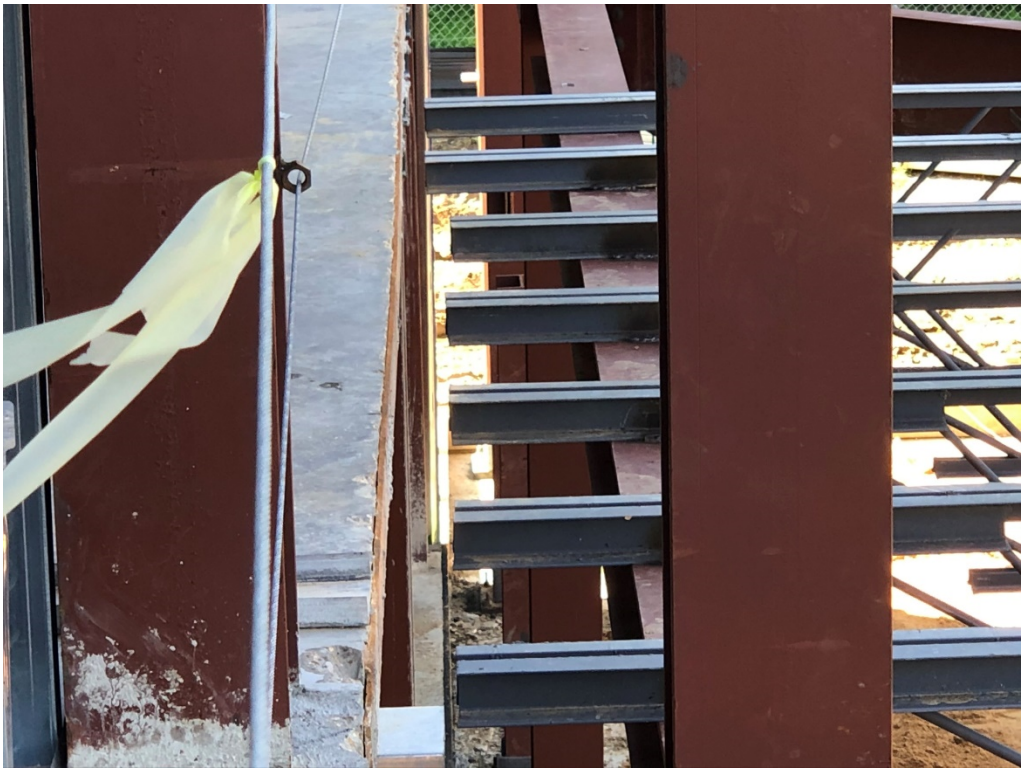
Figure 7 – Mis-aligned end joists
