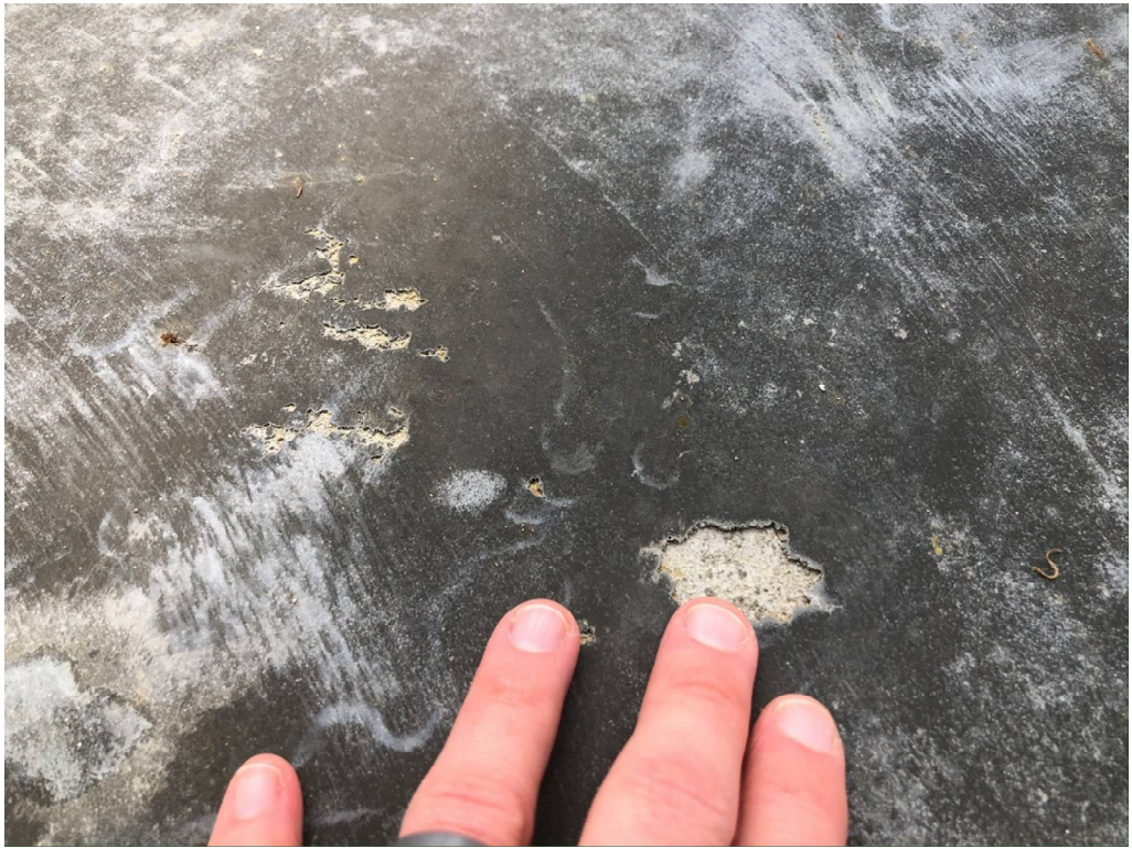
Figure 13 – Spalling at Concrete
