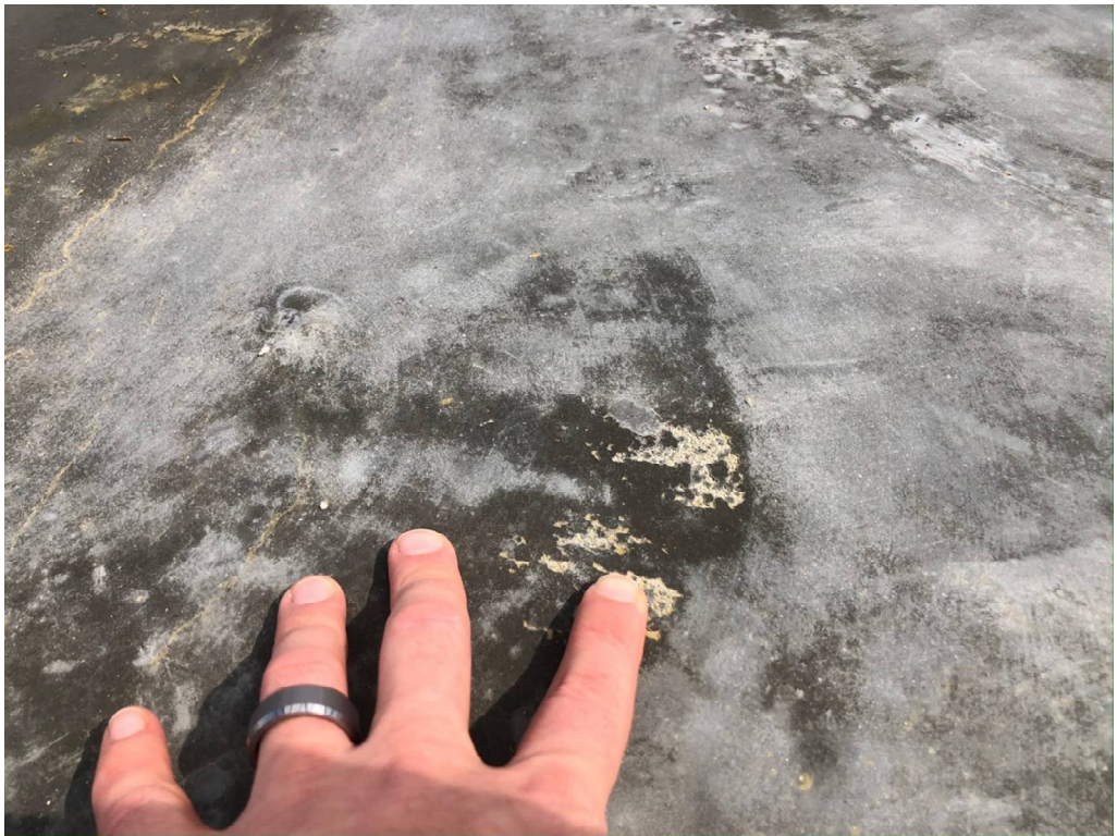
Figure 16 – Spalling at Concrete
