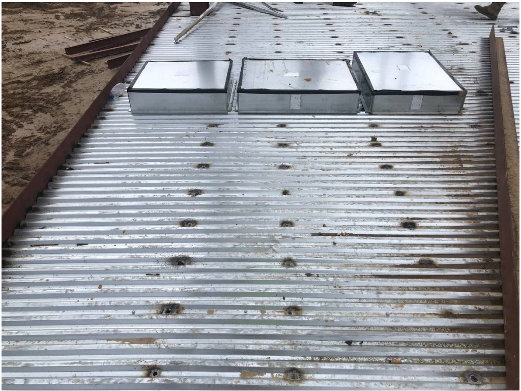
Figure 9 – Contractor Noted Conflict Between Mech & Floor Joists Here
