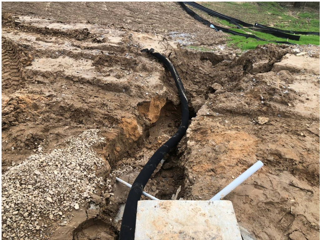
Figure 12 – Continued Wash Out @ Southwest Corner of Lower Building
