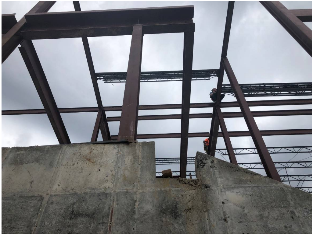
Figure 13 – Mis-Alignment of Concrete Recess and Steel Column
