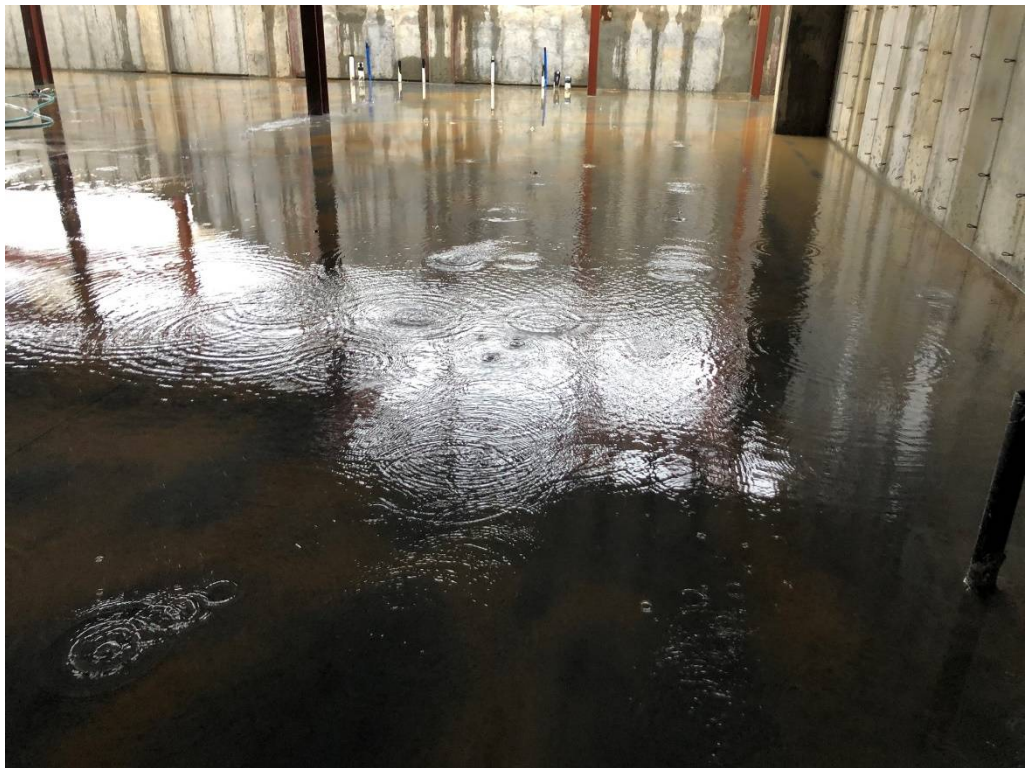
Figure 12 – Potential Low Area in Slab @ East Wall in Lower West Level
