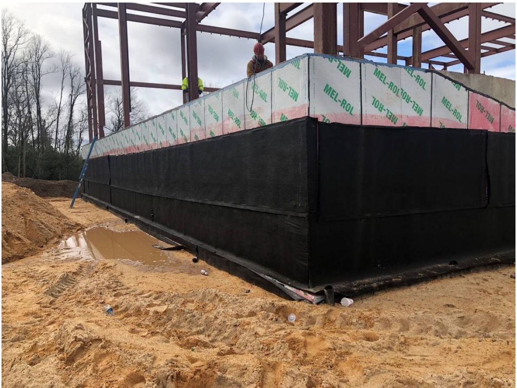
Figure 16 – Note Potential Drainage Pad Break at Corner
