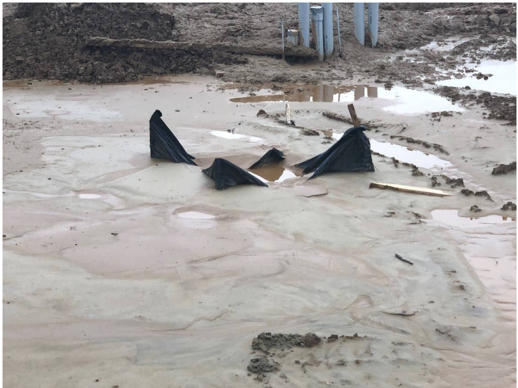
Figure 10 – Storm Sewer Overwhelmed at West Edge of Building Near Parking
