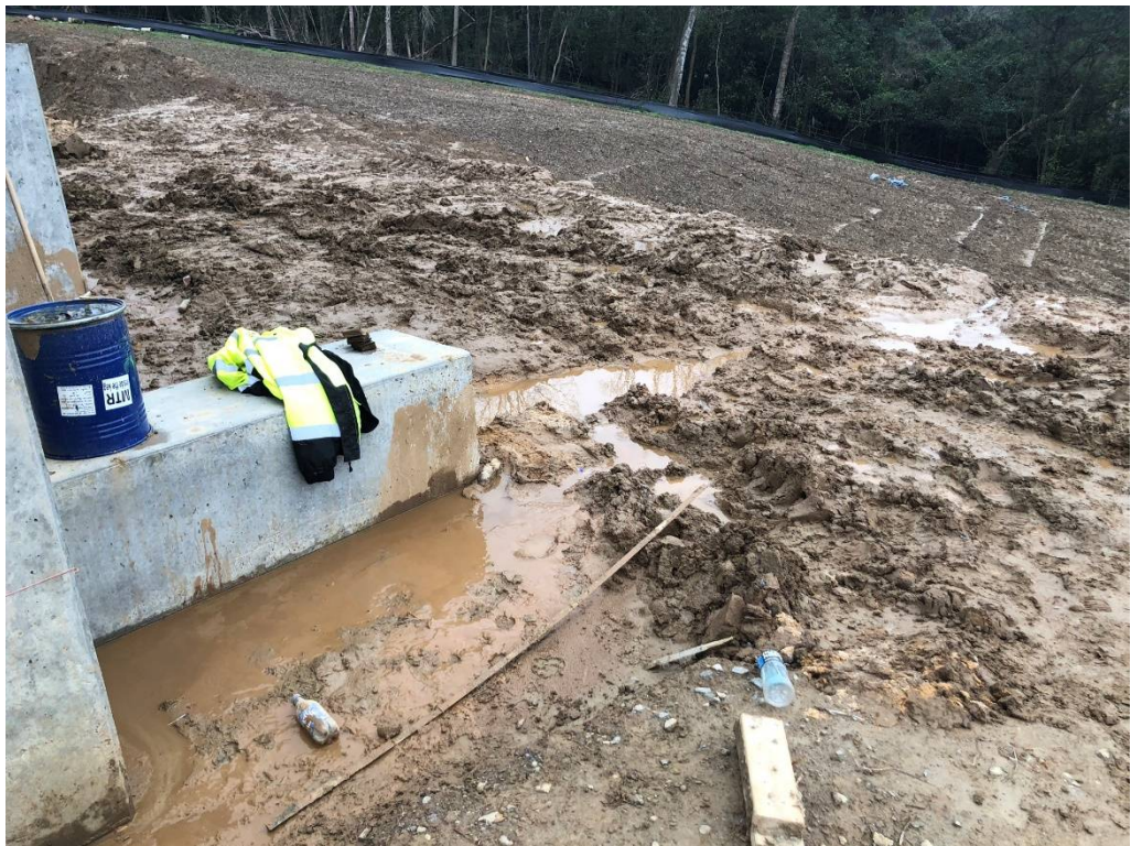
Figure 18 – Southwest Footing Where Previous Erosion Occurred
