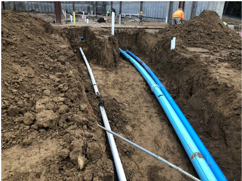
Figure 12 – Services Coming into Building
