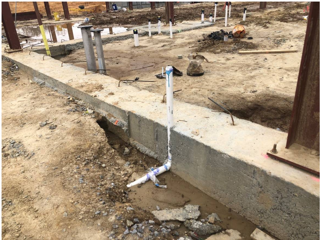
Figure 4 – Erosion @ Southwest Footing (Wednesday)
