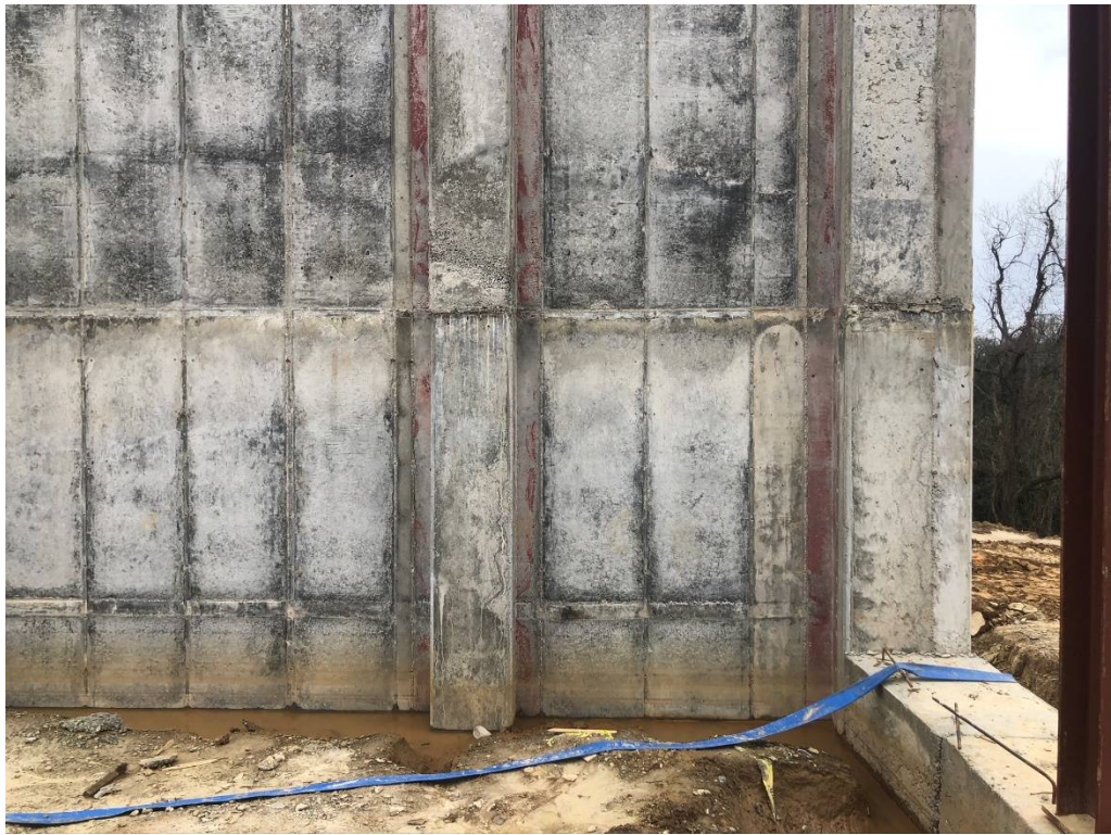
Figure 5 – Inside of Section where Erosion Occurred (Wednesday)
