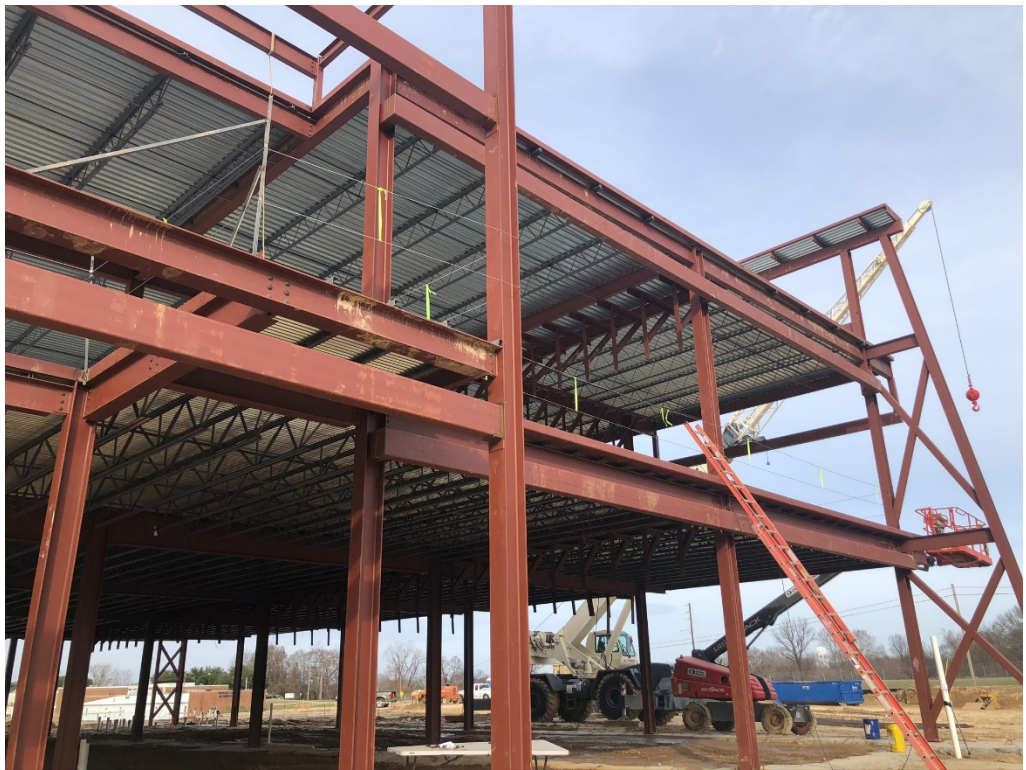
Figure 2 – Safety Wire In Place at 2 nd Floor
