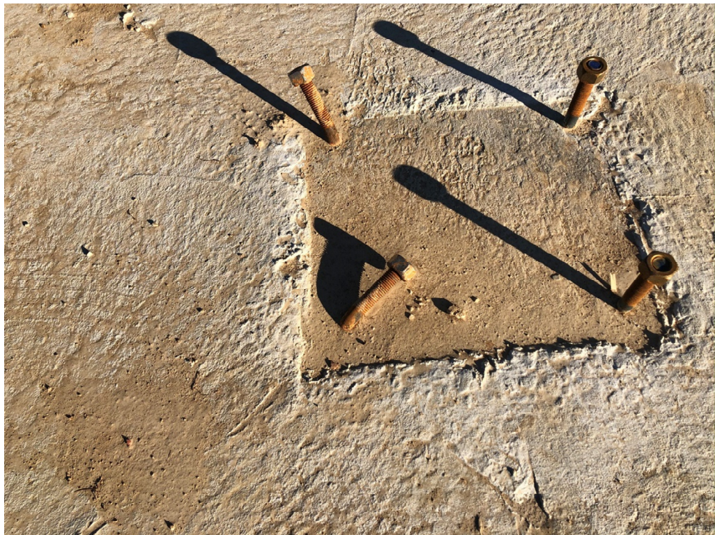
Figure 10 – West Side Upper Slab (damaged bolts @ structural connection)
