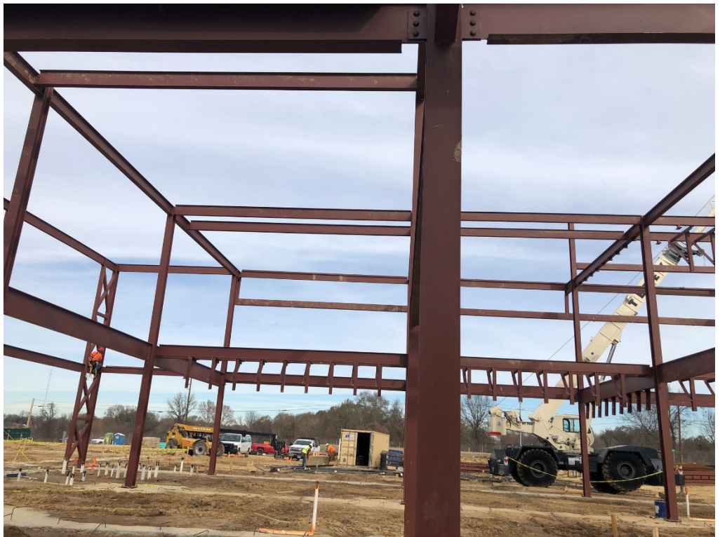
Figure 2 – Steel at Second level slightly out of Plumb (atypical)
