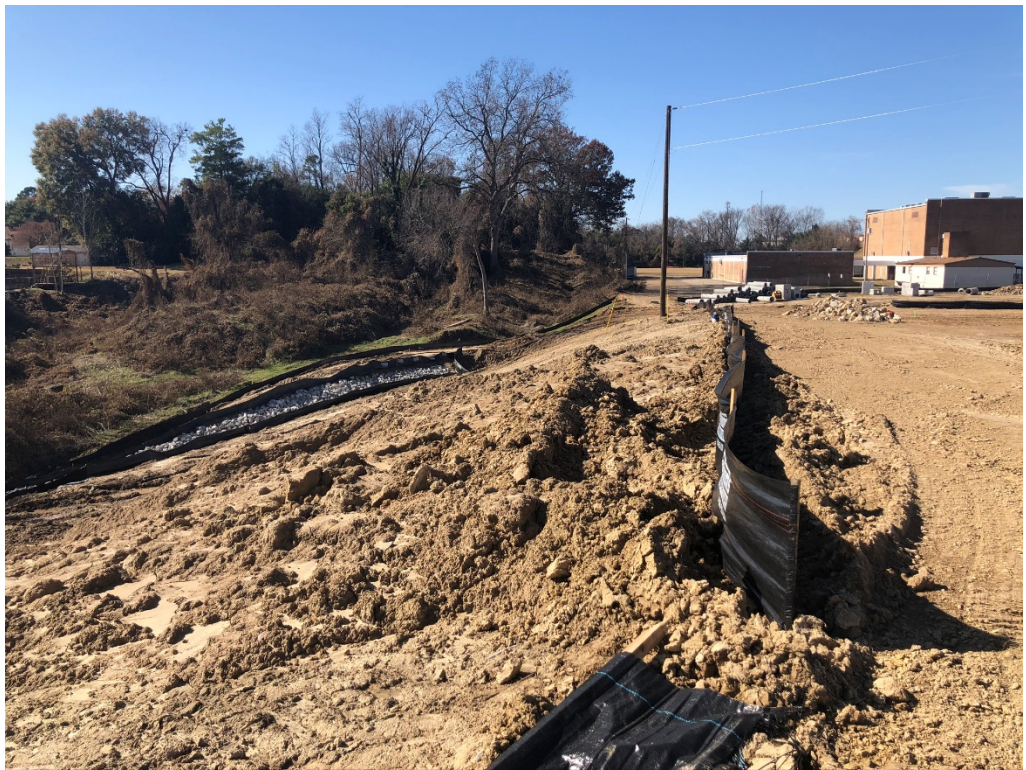
Figure 8 – New Silt Fence at South Edge Of Parking (Also Note New Rip Rap at lower Section)
