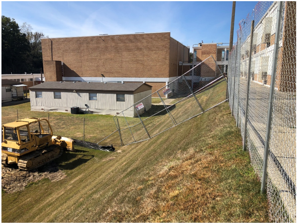
Figure 17 – National Fence Closed Gap in Fencing
