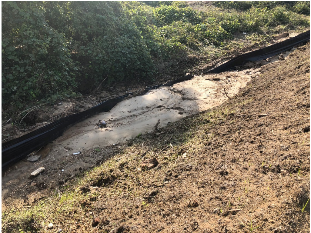
Figure 9 – Low Point in Silt Fencing
