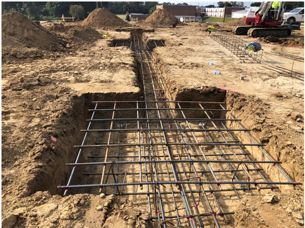
Figure 2 – Isolation footing with Beam (confirm concrete coverage of rebar per Section 032000.3.01/D/5 is adequate)
