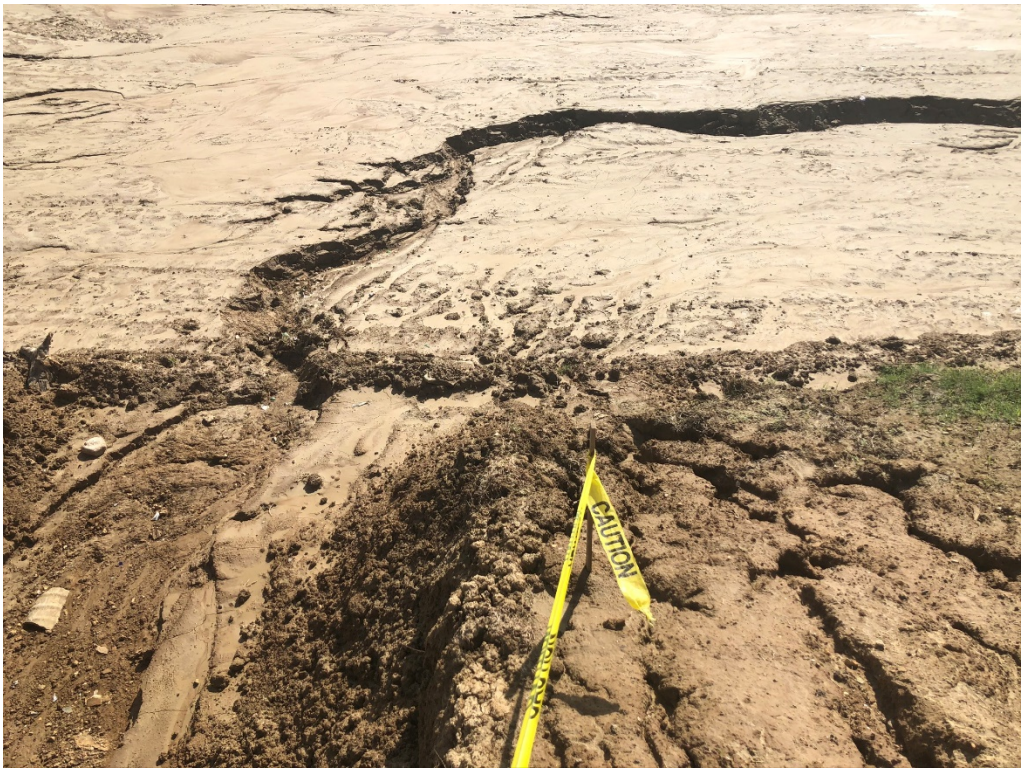
Figure 5 – Wash Out Due to Storm Sewer
