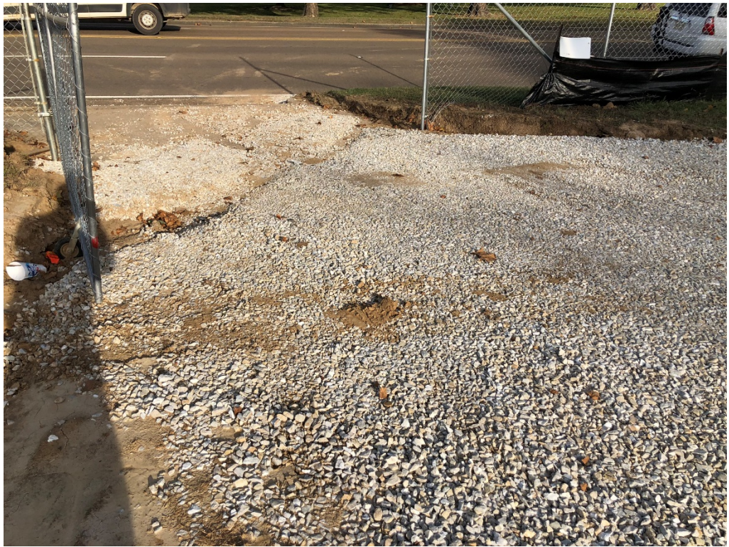
Figure 15 – Natural Drainage Across Temp Drive @ East Entry
