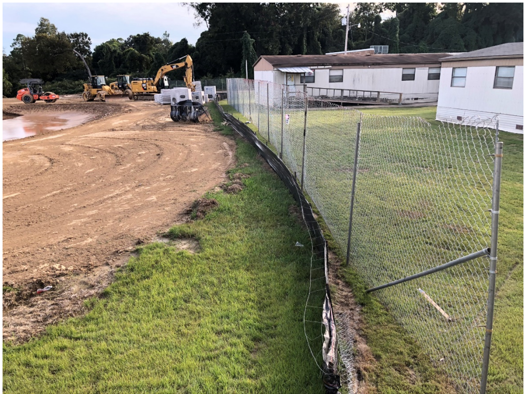
Figure 8 – Temp Fence (gap @ steep slope)
