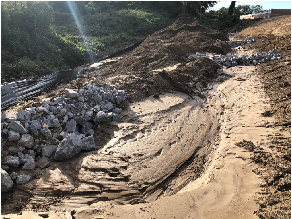
Figure 4 – Riprap Used in Detention (silt fencing in background potentially overwhelmed)
