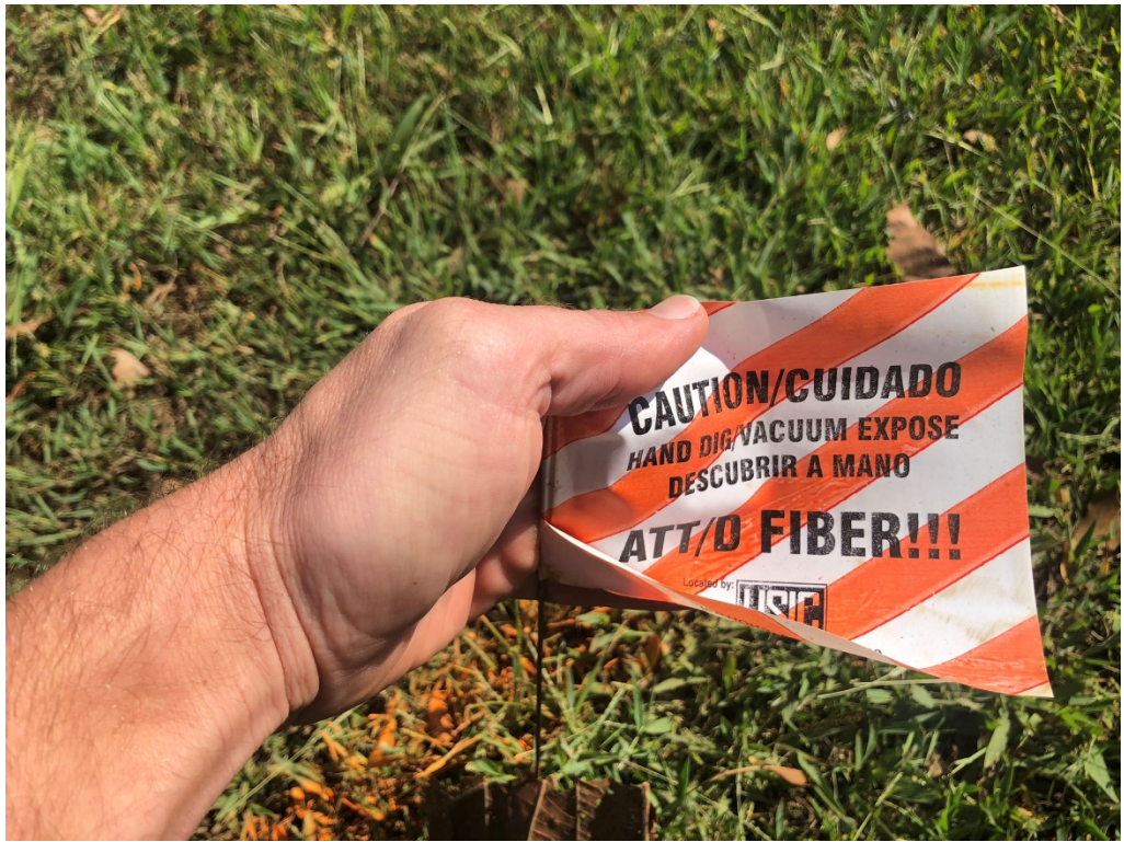
Figure 13 – Orange Marking ATT Fiber at East Side of Site
