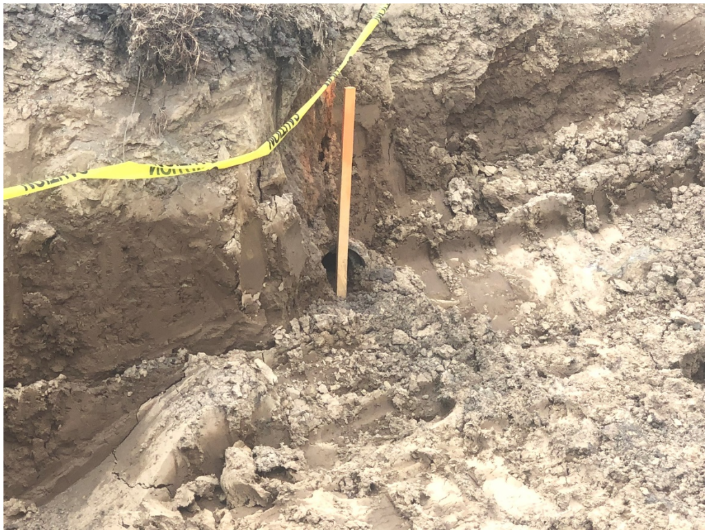
Figure 16 – Hydrant Connection (Removed for Construction)
