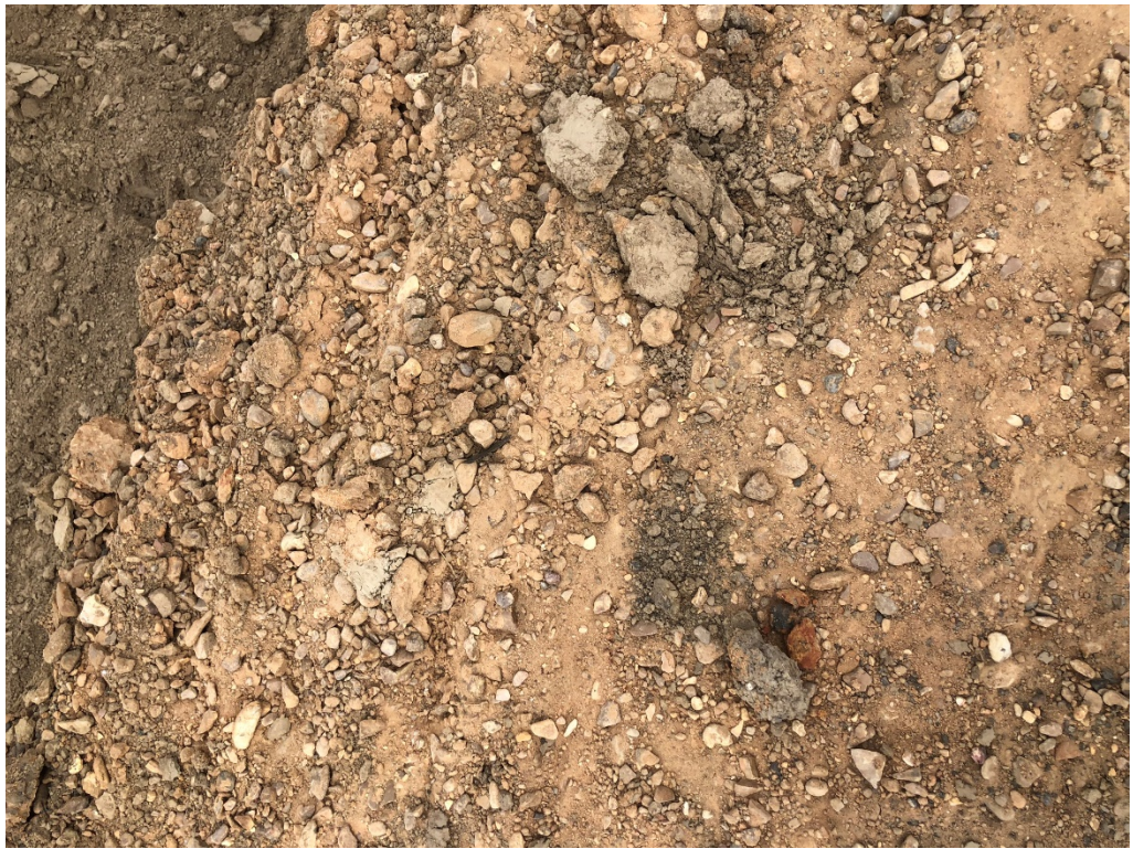
Figure 15 – Aggregate Change NOT Typical @ South Side of Project (road bed)
