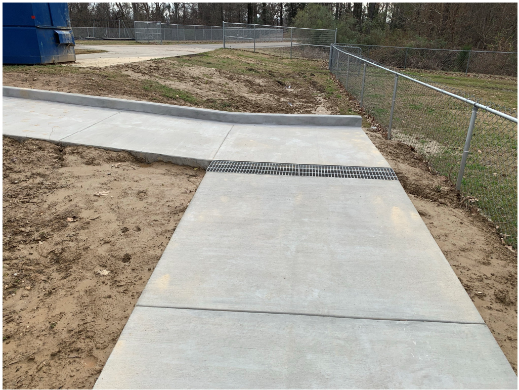
Figure 7 – ADA Ramp Clean Up (note disturbed dirt needs seed or sod to keep from further erosion)
