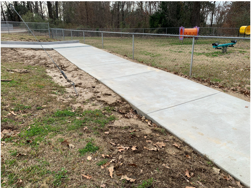
Figure 4 – ADA Ramp Clean Up (note disturbed dirt needs seed or sod to keep from further erosion)
