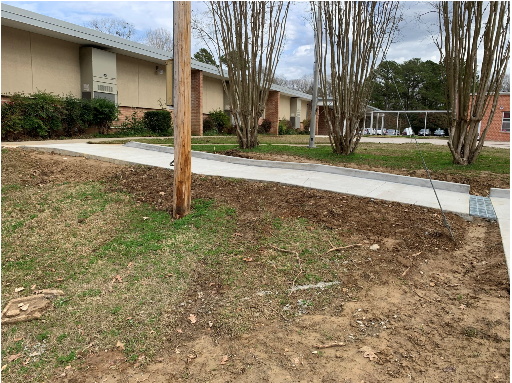
Figure 3 – ADA Ramp Clean Up (note disturbed dirt needs seed or sod to keep from further erosion)
