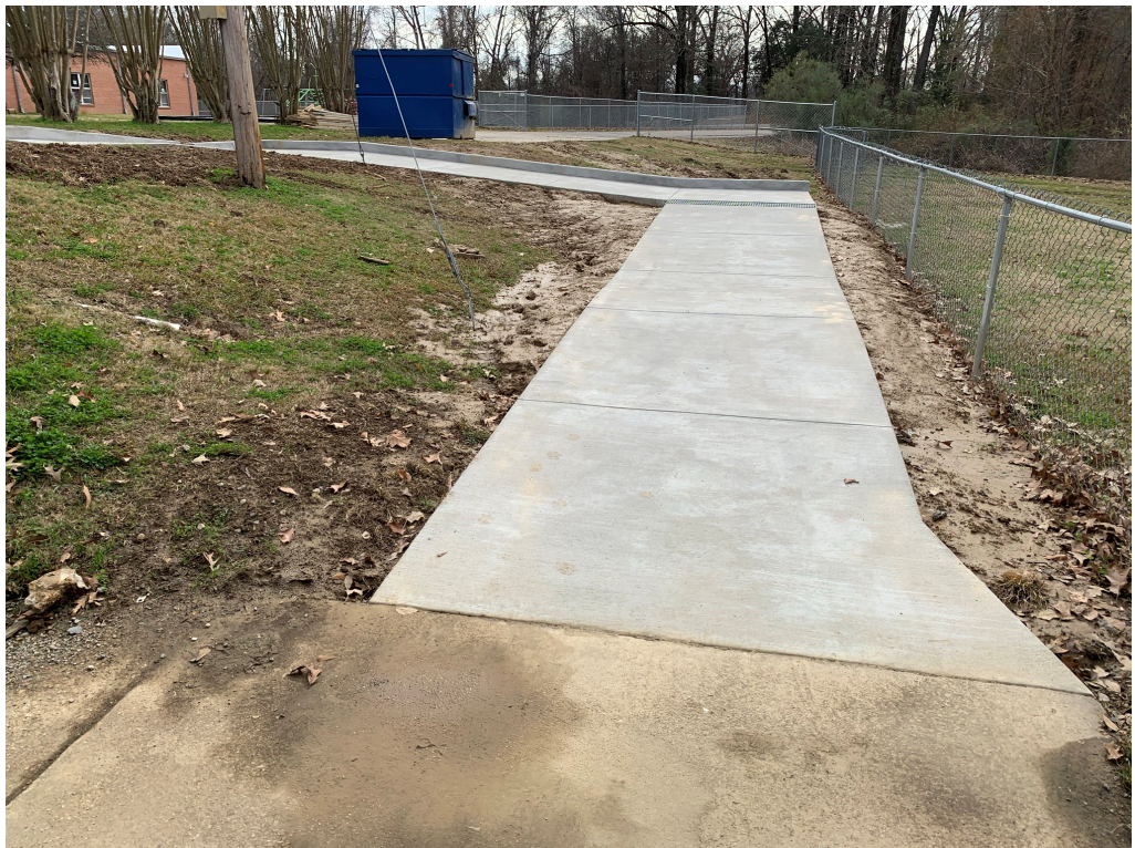
Figure 8 – ADA Ramp Clean Up (note disturbed dirt needs seed or sod to keep from further erosion)
