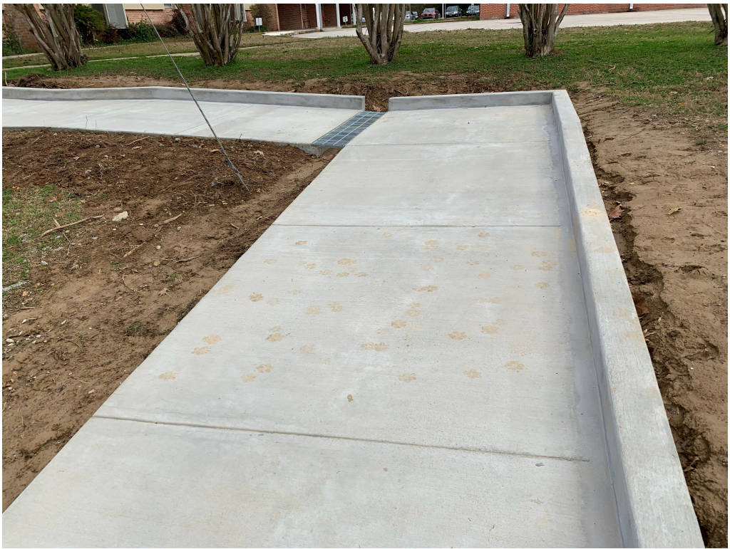
Figure 5 – ADA Ramp Clean Up (note disturbed dirt needs seed or sod to keep from further erosion)
