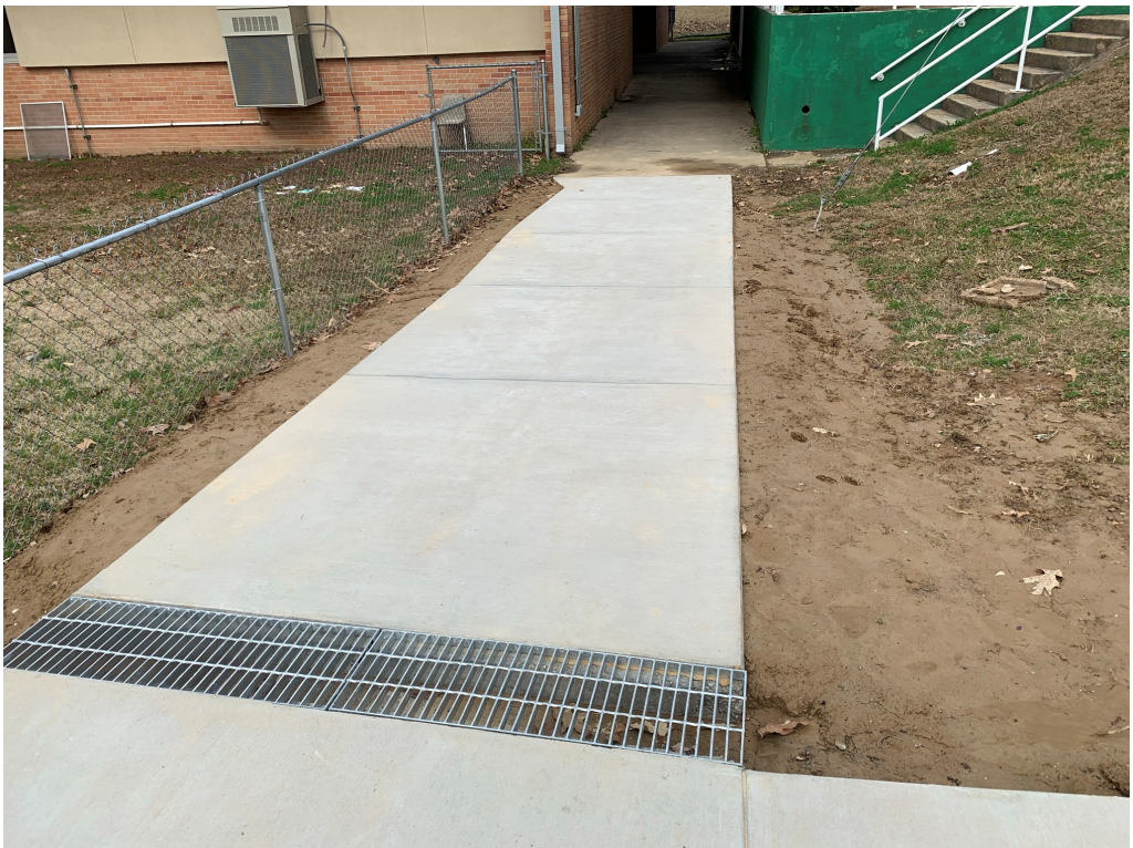
Figure 6 – ADA Ramp Clean Up (note disturbed dirt needs seed or sod to keep from further erosion)
