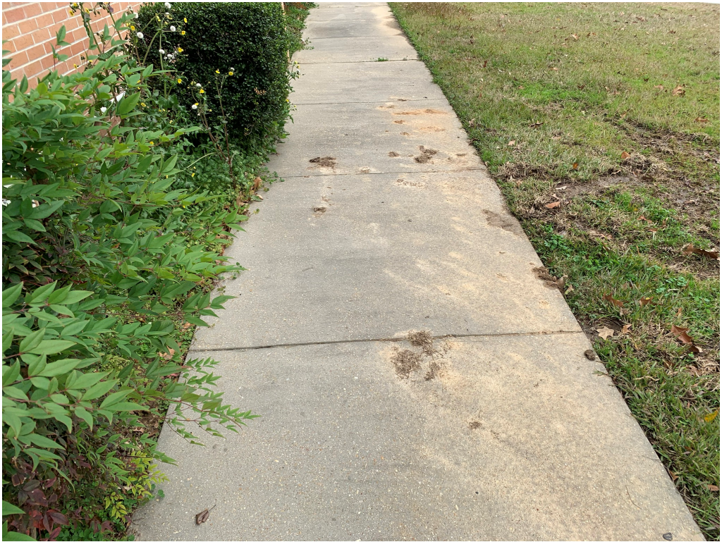
Figure 1 – Tracked Dirt at Existing Sidewalk
