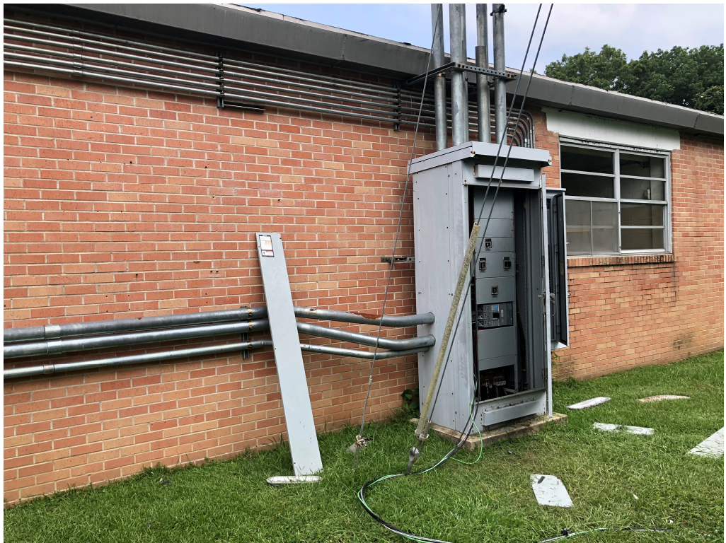
Figure 2 – Temporary Power Run from Main Panel (temporary protection or caution tape needed around open panel if left open continually throughout the day)
