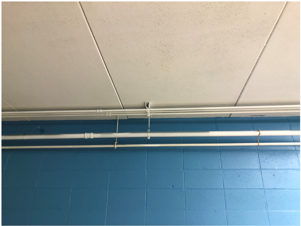
Figure 1 – Ceiling paint Work; Pipes should be fully painted if attached to ceiling.
